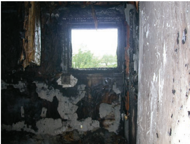
Figure 5.15 Inside a room in which a pig carcass had decomposed for 42 days, after a simulated arson. (Photo courtesy of Dr. Gail Anderson.)
