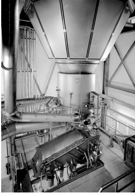
Fig. 3.16 Drying chamber cone with integrated fluid-bed dryer and sieve with cleaning-in-place (CIP) nozzles. Data by permission of A.J. Partridge (personal communication) and GEA Process Engineering (Niro A/S), Gladsaxevej 305, Soeborg, Denmark.
