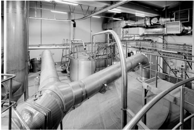
Fig. 3.22 Air exhaust ducting from top of the spray drying chamber equipped with cleaning-in-place (CIP) nozzle. Data by permission of A.J. Partridge (personal communication) and GEA Process Engineering (Niro A/S), Gladsaxevej 305, Soeborg, Denmark.
