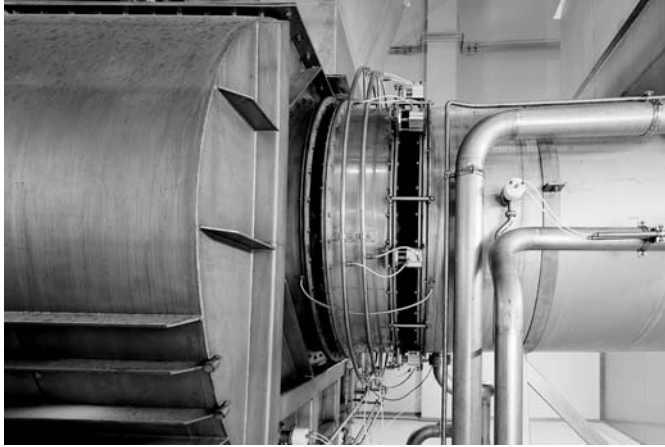
Fig. 3.24 Vapourtight damper that isolates and keeps the Sanicip™ dry during the wet cleaning of other parts of the dryer. Data by permission of A.J. Partridge (personal communication) and GEA Process Engineering (Niro A/S), Gladsaxevej 305, Soeborg, Denmark.
