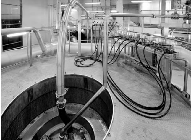
Fig. 3.20 Spray drying chamber in cleaning-in-place (CIP) mode; the atomiser nozzles are removed from atomisation zone and a CIP turbine cleans the surface of the inner chamber walls. Data by permission of A.J. Partridge (personal communication) and GEA Process Engineering (Niro A/S), Gladsaxevej 305, Soeborg, Denmark.
