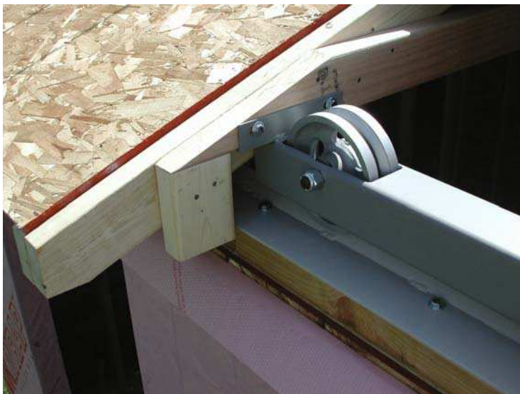
Figure 1.25. “Rocky Plains Observatory” roller system – the wheels are V-groove, same as suggested in our plan but Bob has ingeniously enclosed them in a steel box beam – each roof section carries its own two sets of box beams enclosing the wheels. (Courtesy of Bob Luffel) (See Color Plates ).
