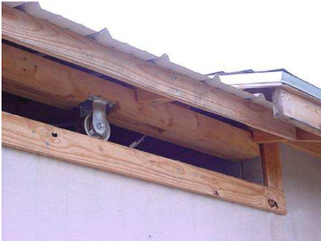
Figure 1.30. “Ballauer Observatory” – illustrating how roll-off roof tucks under the higher warm room roof above it. Note casters and the large air gap between roof and walls. (Courtesy of Jay Ballauer) (See Color Plates ).
