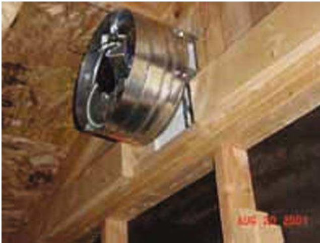
Figure 11.5. Photo of internal fan housing fitted to inside of gable wall. (Courtesy of Jay Ballauer).
