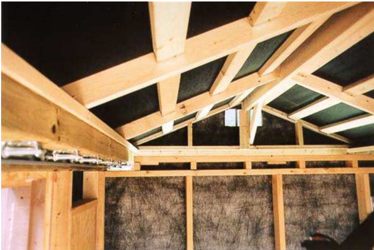
Figure 1.20. "The Ussher Observatory" – roof interior showing rafters and no collar ties. (Courtesy of Terry Ussher) (See Color Plates ).
