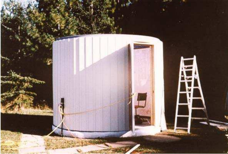
Figure 11.2. Photo of vinyl siding application on domed observatory exhibiting its elegant appearance. (Photo by John Hicks).
