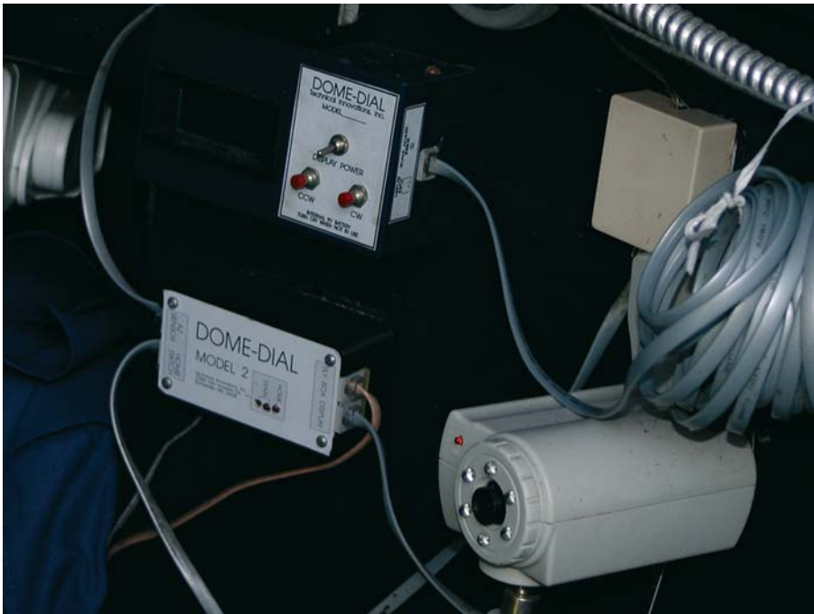
Figure 2.14. Dome-Dial display unit and relay box, mounted on observatory wall. Black-and-white security camera is also shown. (Used with permission, Technical Innovations, Inc.)
