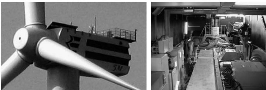
Figure 6.41 Exterior and interior of the nacelle of a 5 MW wind turbine
