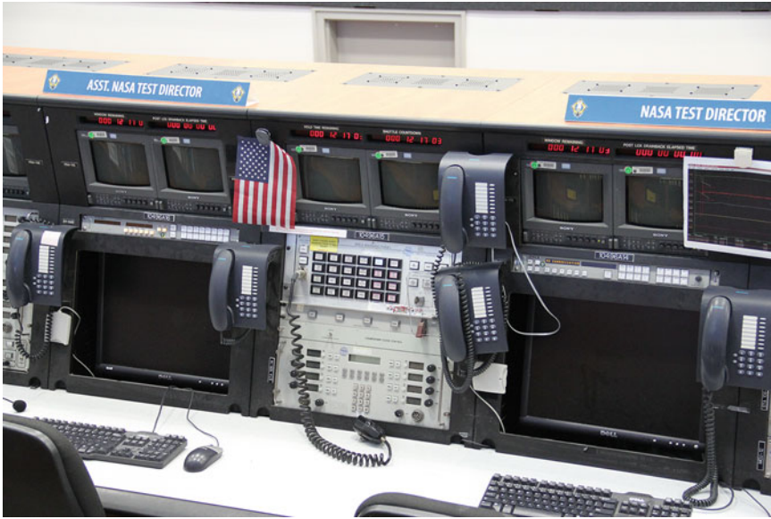
Fig. 3.2 A typical workstation in the Launch Control Center at the Kennedy Space Center as it was during the Space Shuttle era. From here, launches were monitored and controlled. As soon as the crewed spacecraft have launched, control is handed off to the Mission Control Center (MCC) in Houston, Texas (Image: B. Ganse)
