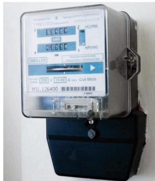
▲ The electricity meter shows how much energy you have used in kWh.
