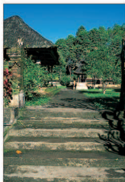
Steps to temple hindering wheelchair access
