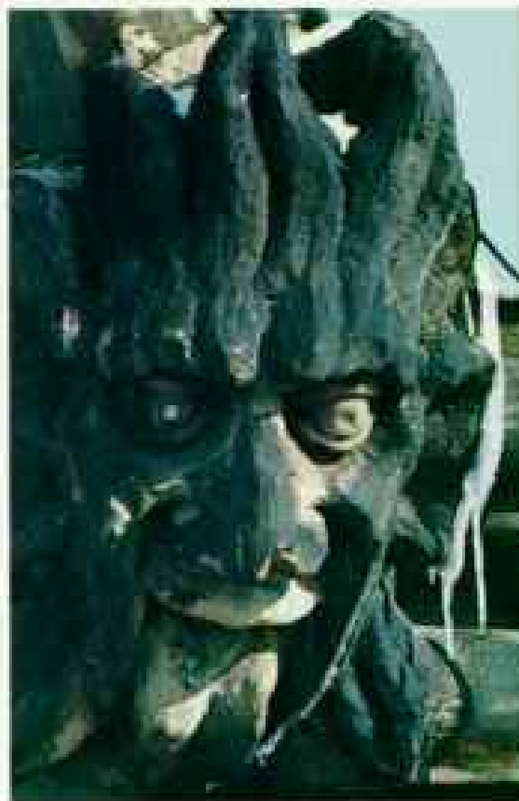
SARGOYLE ON CANADA'S PARLIAMENT BUILDINGS IN OTTAWA CORRODED BY AIR POLLUTION. PHOTOGRAPH BY TED SPIEGEL, BLACK STAR
