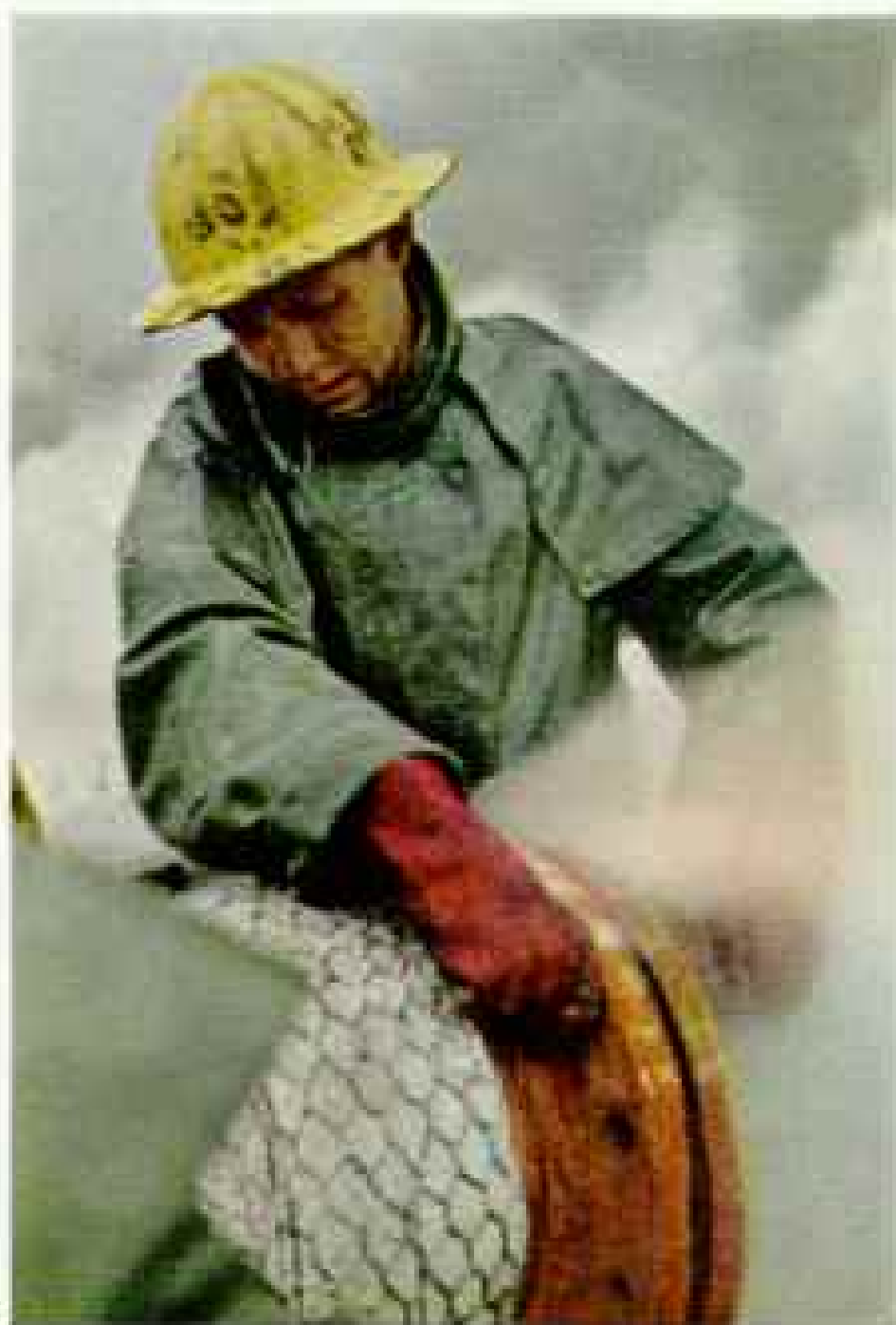
Scalding steam escapes from a pipe connection. Hard hat and rubber coat and gloves protect the workman.
