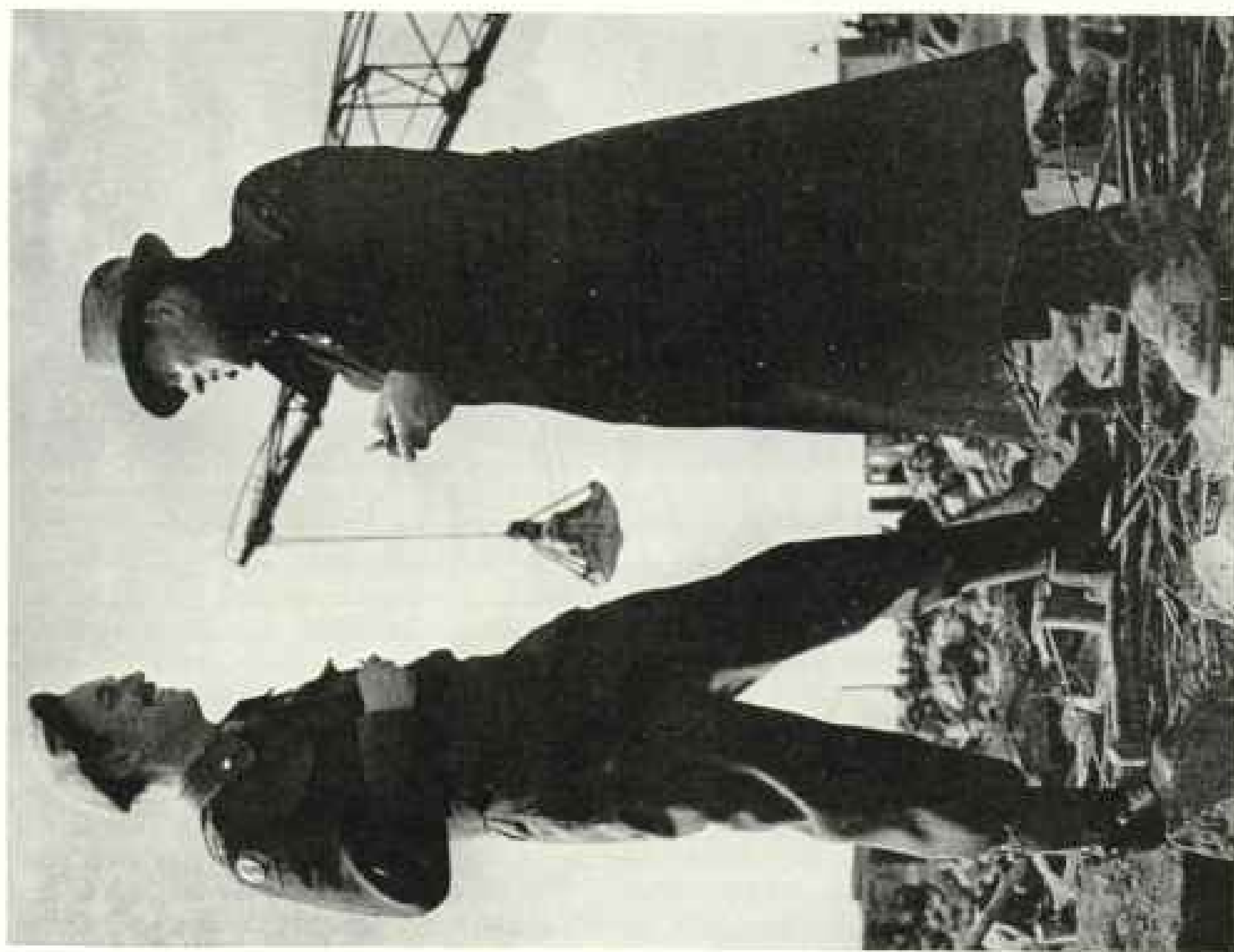
A British Brigadier and Dutch Engineer Discuss the Job's Progress If the gaps had not been closed, Walcheren might have been washed away, closing the port of Flushing (Vlissingen) and interfering with navigation to Antwerp.
