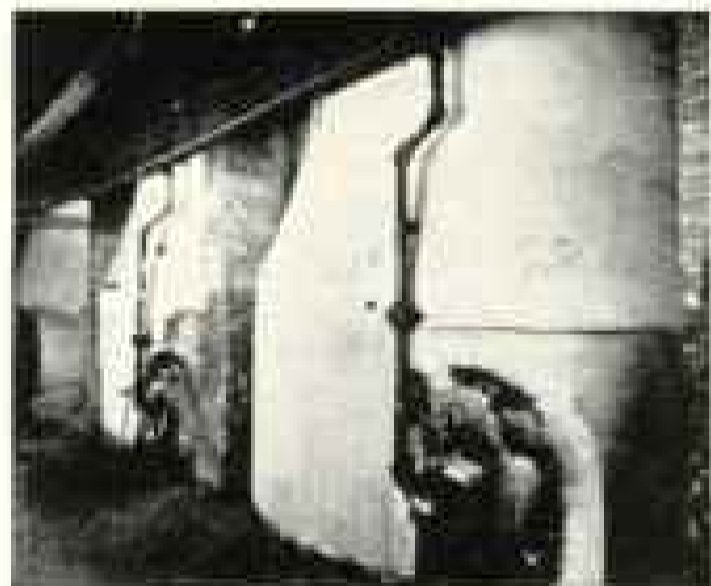
The George W. Prentiss Co. of Holyoke, Mass., greatly improved the efficiency of an old furnace by insulating it outside with Johns-Manville Superex, 85% Magnesia and No. 502 Cement.
