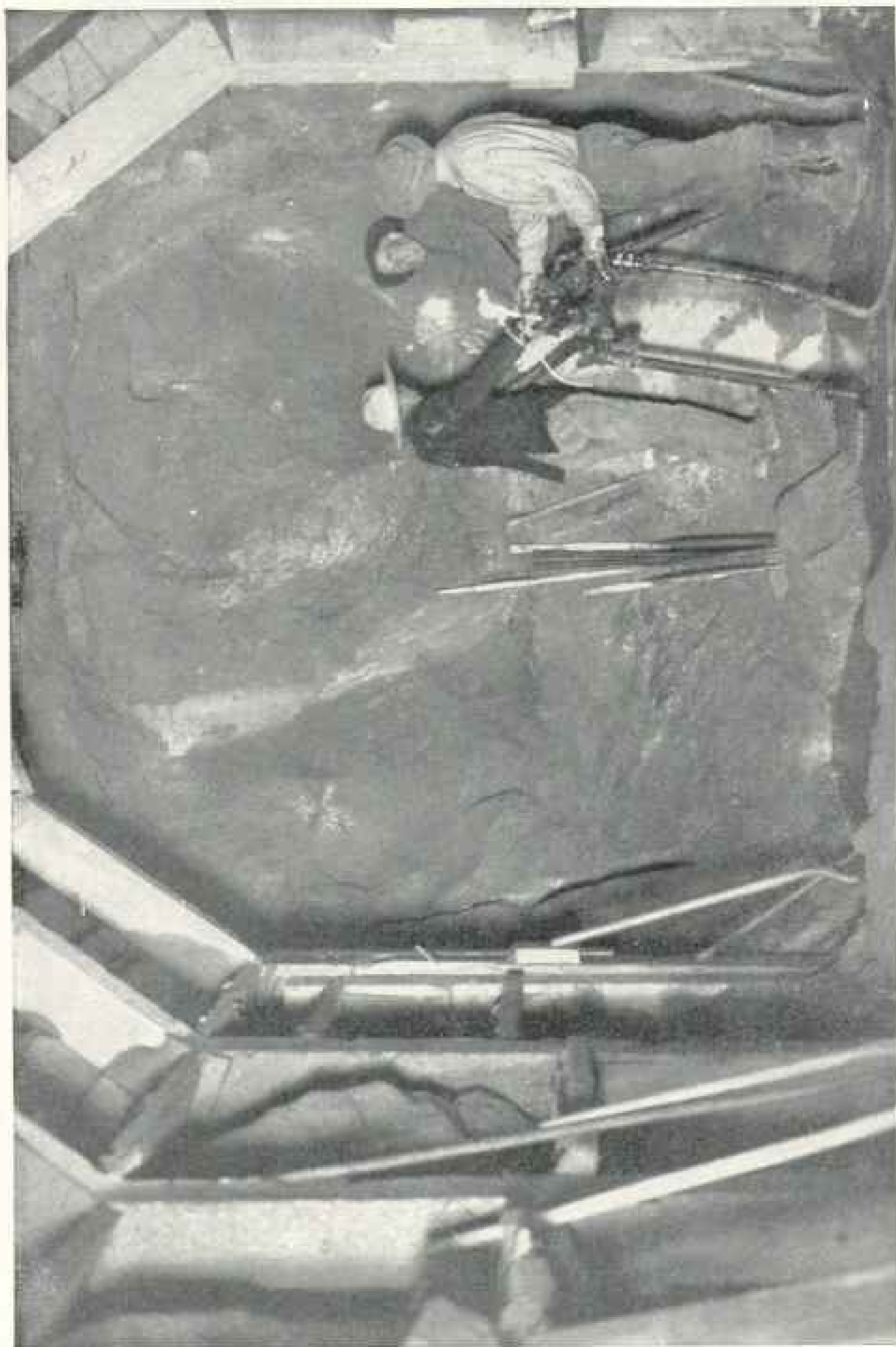
IN THE SOUTH PORTAL OF THE ELIZABETH TUNNEL, WHICH IS NEARLY FIVE MILES LONG (26,800 FEET), AND PASSES UNDER THE COAST RANGE
