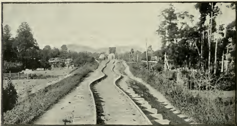
TWISTED BY AN EARTHQUAKE.
