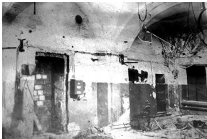
Fig. 6.32. Old photograph of 1985 which reveals the condition of the Church of Our Lady's Nativity right after the departure of the factory authorities. This photograph can be seen on the billboard with information on the history of the church's reconstruction next to the entrance. The legend says "The final resting place of Peresvet and Oslyabya, the heroes of the Kulikovo Battle. 1985." We made a copy of the photograph in 2000; what we see is a picture of utter devastation.
