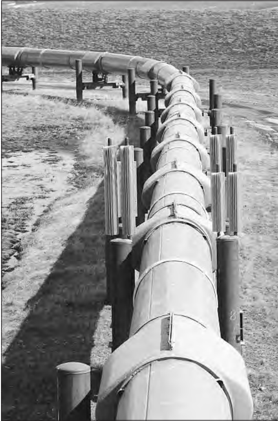
A section of the Alaska Pipeline, which carries crude oil from the state's northern slopes to Valdez on Alaska's southern coast. (PhotoDisc)
