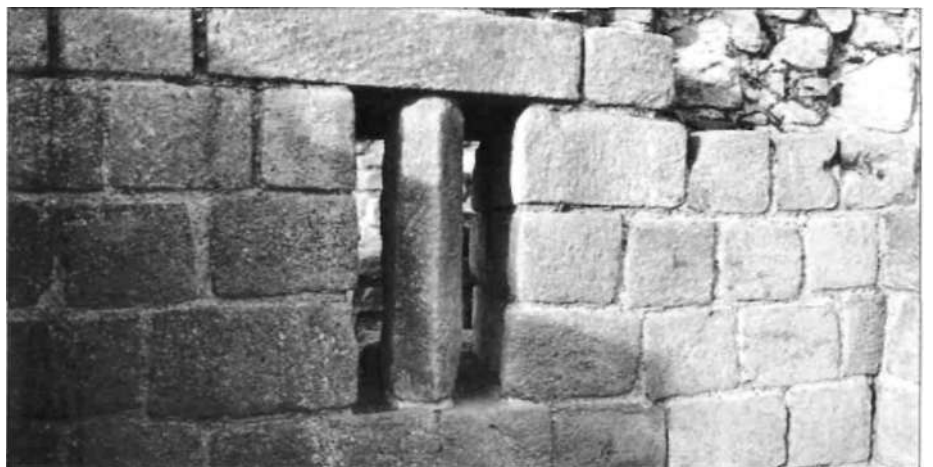
Detail of an under-floor ventilator with central mullion at the west granary of Corbridge ( Coria ).This ventilator allowed air to circulate under the floor and thus protect foodstuffs from becoming damp. (Author's Collection)
