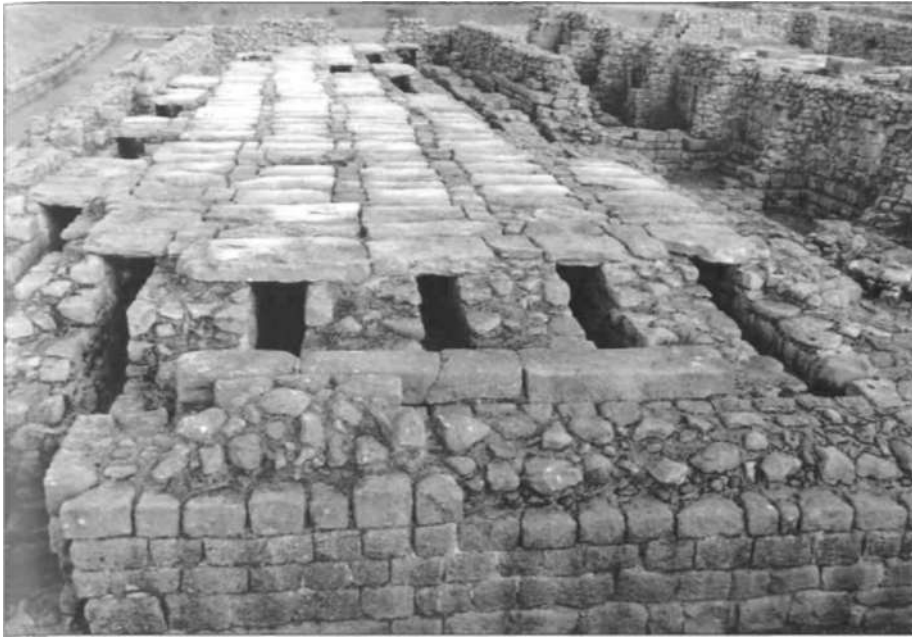
The longitudinal dwarf-walls that support the flagged floor of the east granary at Corbridge (Corifl). The flooring is overlying channels that allowed air to circulate freely throughout the building's sub-structure, thereby preventing damp. (Author's Collection)
