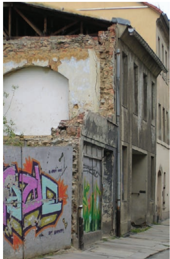
Figure 2.28 Forward lean of wall with tension cracks showing in return wall.
