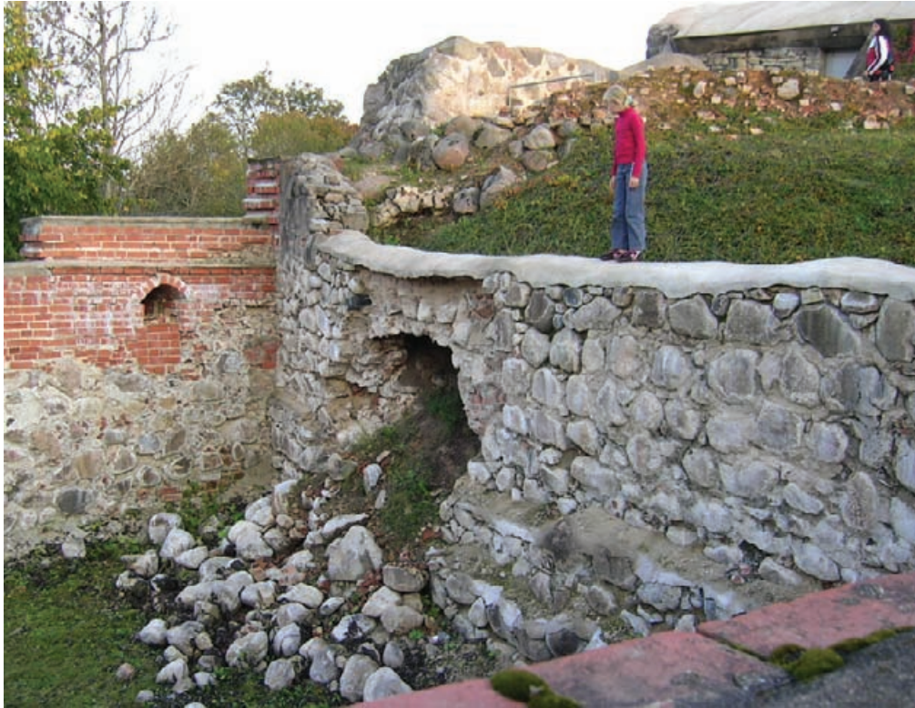
Figure 2.31 Retaining wall failure under earth and water pressure.
