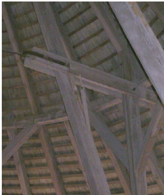
Figure 2.14 Evidence of lightning strike, Cesis Castle, Latvia.
