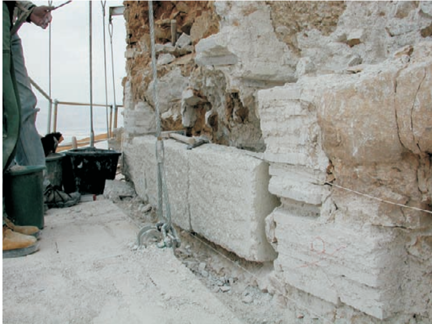
Figure 10.24 During the progress of the facing work the surviving original stones can be seen in the foreground. Adjacent to them are two stones which have been repaired with split tile and lime mortar. Beyond the repairs can be seen three of the cast lime blocks with a roughened texture. The consolidated Tholos wall is now a mixture of original stone faces, repaired original stones and new cast stones where the facing was missing. Every part of the original face was secured and saved.
