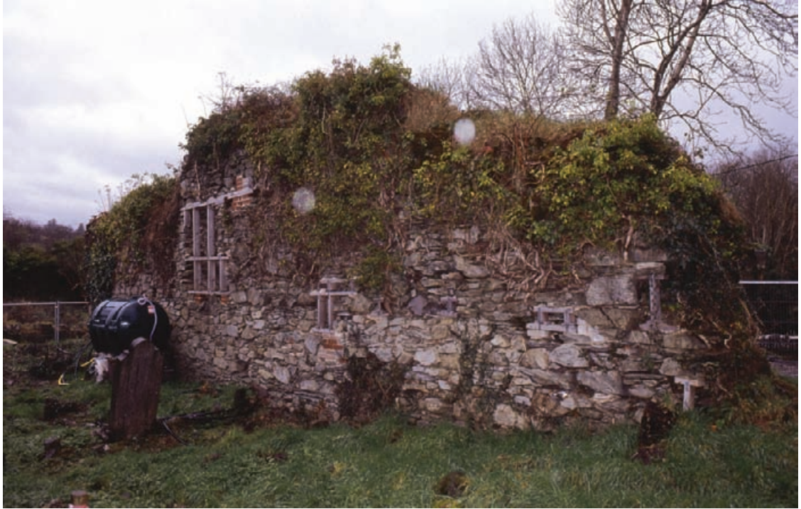
Figure 3.4 Mourneabbey, Cork, Republic of Ireland: the absence of protective roofs and wall plasters leaves ruined walls vulnerable to uncontrolled water ingress and invasive, destructive plant growth.
