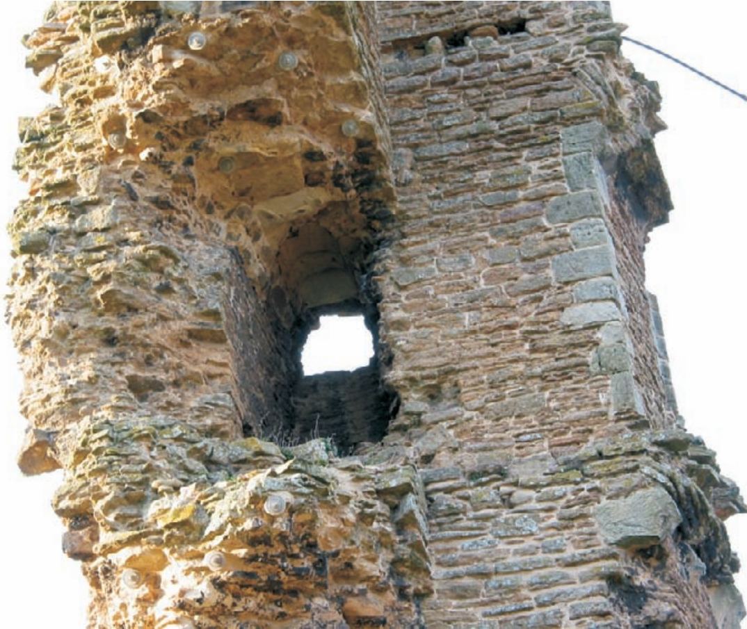
Figure 4.40 Pattress plates and anchors used to tie back overhanging core work at Sheriff Hutton Castle.
