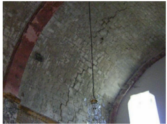
Figure 2.45 Cracked vault related to wall movement.
