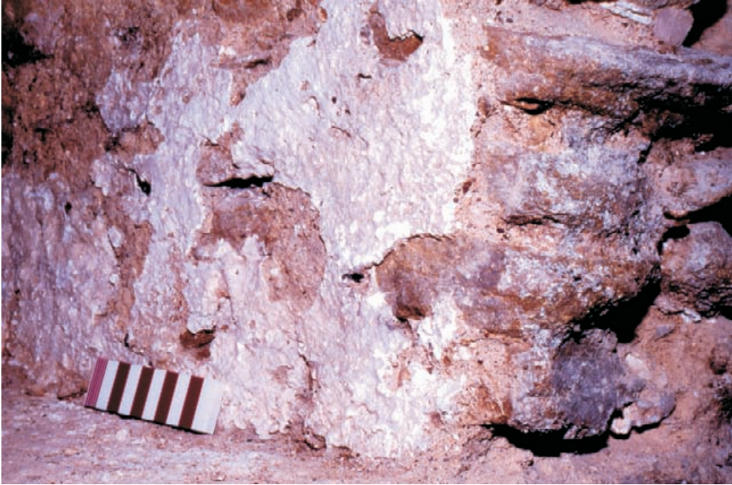
Figure 10.5 Detail of Norman plaster (in Figure 10.5) applied to the merlon in the tower's first phase of construction.
