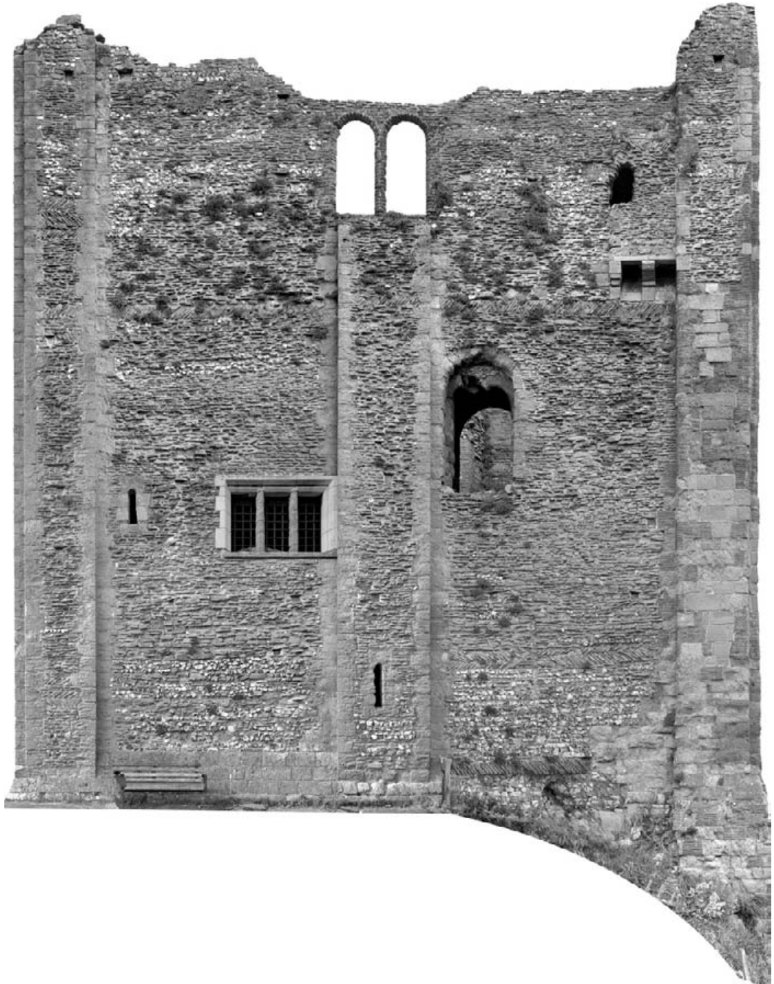
Figure 3.19 Guildford Castle. Rectified photographs can be used in the absence of elevation drawings.
