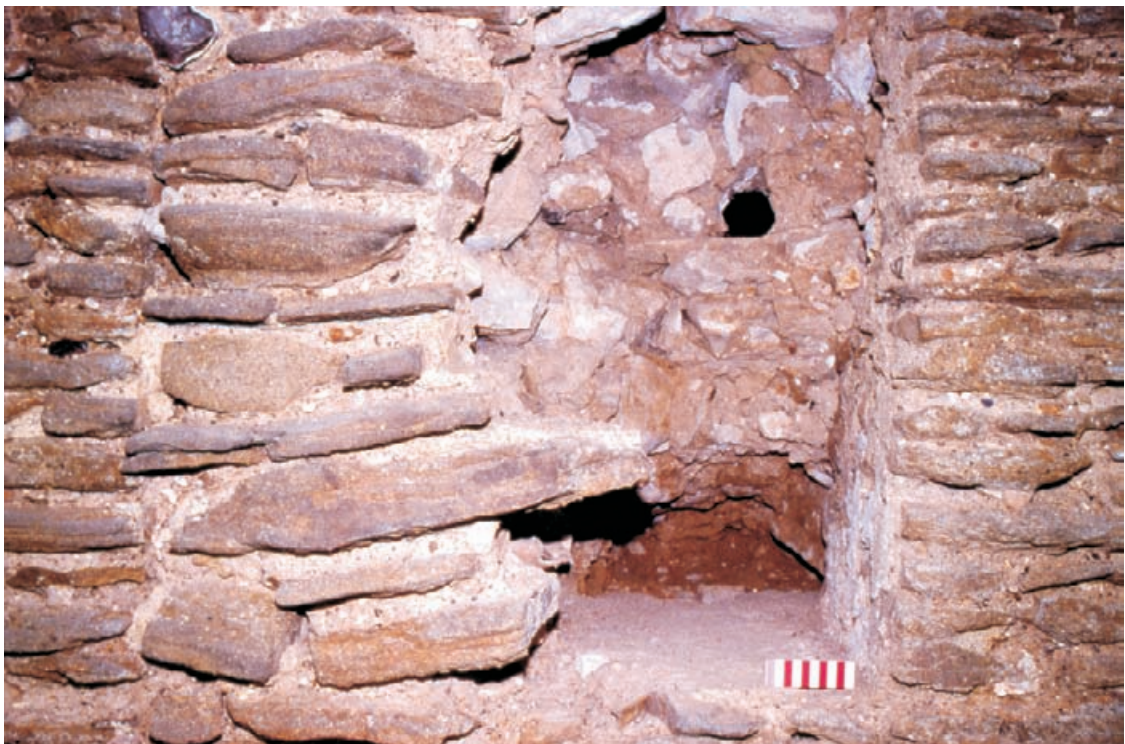
Figure 10.4 Blocked embrasure on the west elevation in the course of excavating fill to expose the plastered vertical face of the merlon.
