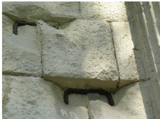
Figure 2.49 Corrosion damage from Roman iron cramps.
