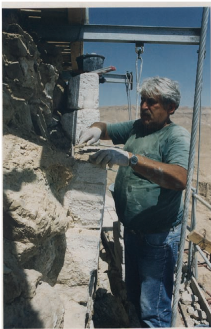
Figure 10.21 Work proceeding from a suspended scaffold placing cast blocks back on the line of missing stones.
