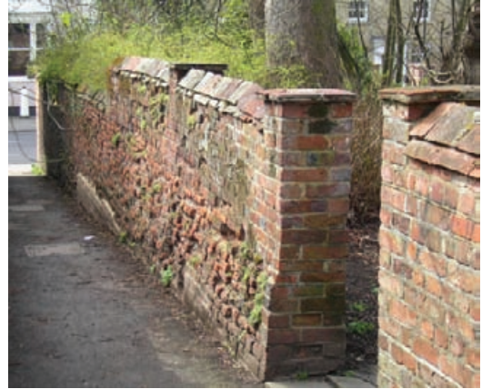
Figure 2.18 Common frost damage caused by accumulation of soil.
