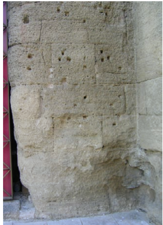
Figure 2.19 Stress cracking of the Roman Theatre at Orange (1).
