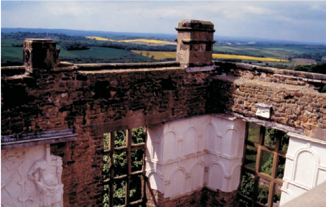
Figure 4.74 Plaster survival in wet conditions. Decorative plaster at this level, seen at Hardwick Old Hall, is particularly susceptible to damage by water and colonisation by organic growth. In the absence of a roof, protection is provided by small, timber board projections of 300–450 mm, covered with lead. The upturn of the lead against the wall must be into a carefully formed wall chase, secured with stainless steel screws and washers. Maintenance is essential, including the use of thin lime washes.
