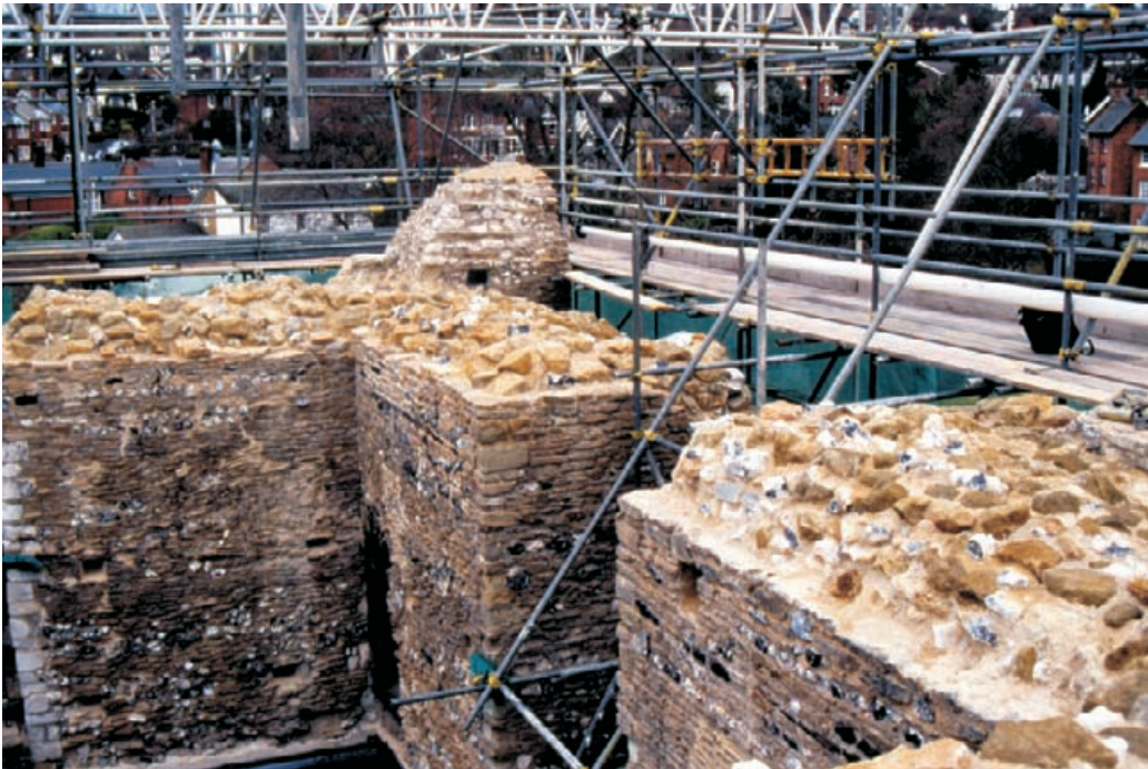
Figure 10.6 Existing flat screeds were removed and core work constructed to shed water off the wall heads and indicate their broken form prior to 'rationalisation' in the nineteenth and twentieth centuries.
