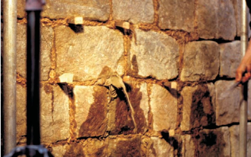
Figure 4.47 At the base of the wall this illustration shows grout emerging from one of the escape holes provided, confirming the rise of grout behind the face stones. The blocks here are shown levelled with oak pegs and the joints plugged, in the traditional way with tarred rope.
