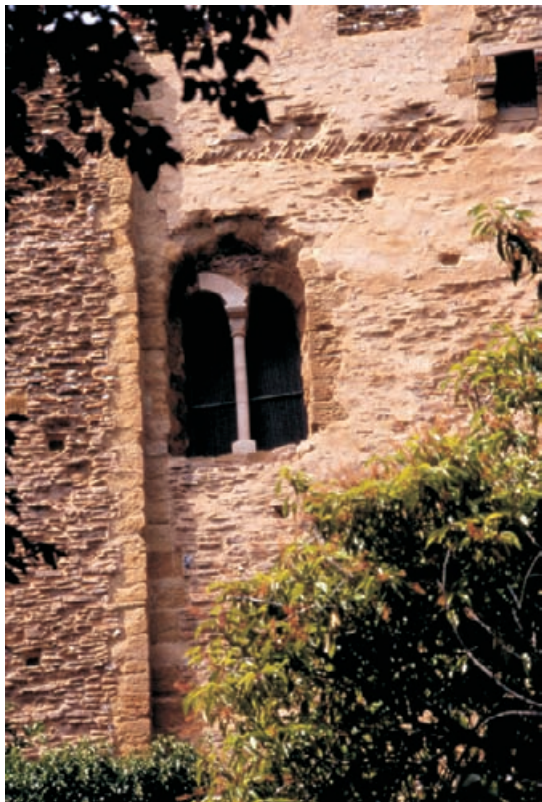
Figure 10.8 None of the Norman window mullions survived and one was reinstated in the south window to support the remaining voussoirs and interpret the early window detail.
