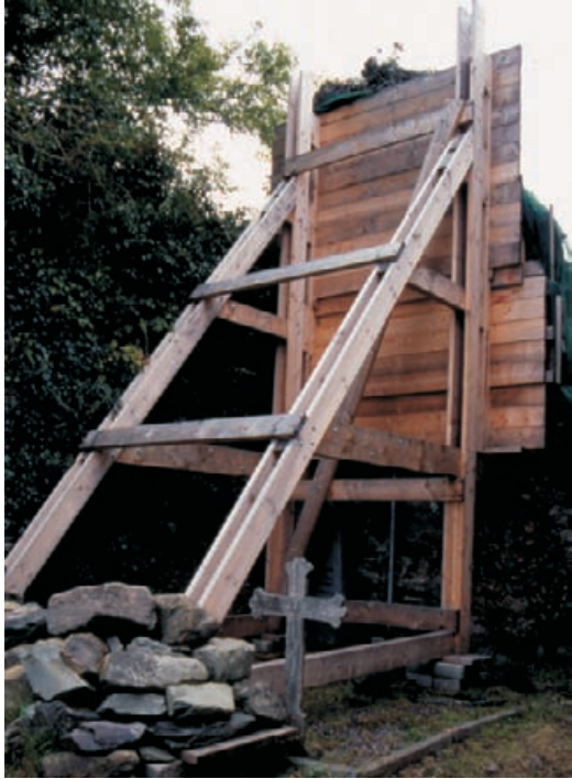
Figure 4.8 Temporary support of high leaning wall in the form of board facings and flying shores.
