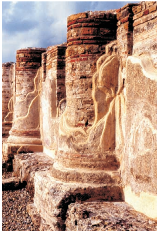
Figure 4.73 Plaster survival in dry conditions. Multi coat plaster at Paestum. Plasters in these conditions can become detached through the activity of soluble salts migrating in the wall, especially after excavation. Detachments may need to be grouted with weak hydraulic lime and broken edges closed up with weak hydraulic lime mortar, carefully cured. Regular inspection of these important plasters is essential and replacement of protective mortar fillets may be needed from time to time.
