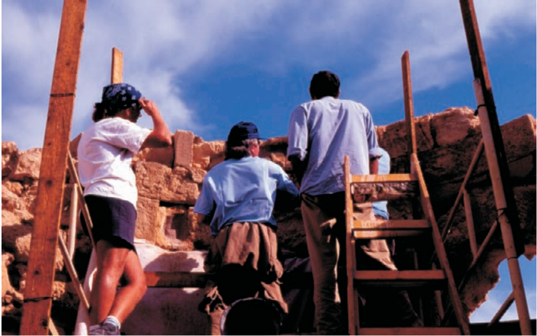
Figure 8.4 Site training with Asi Shalom's conservator team on the Byzantine Church at Masada. Stabilisation of weak surfaces and consolidation of wall heads.
