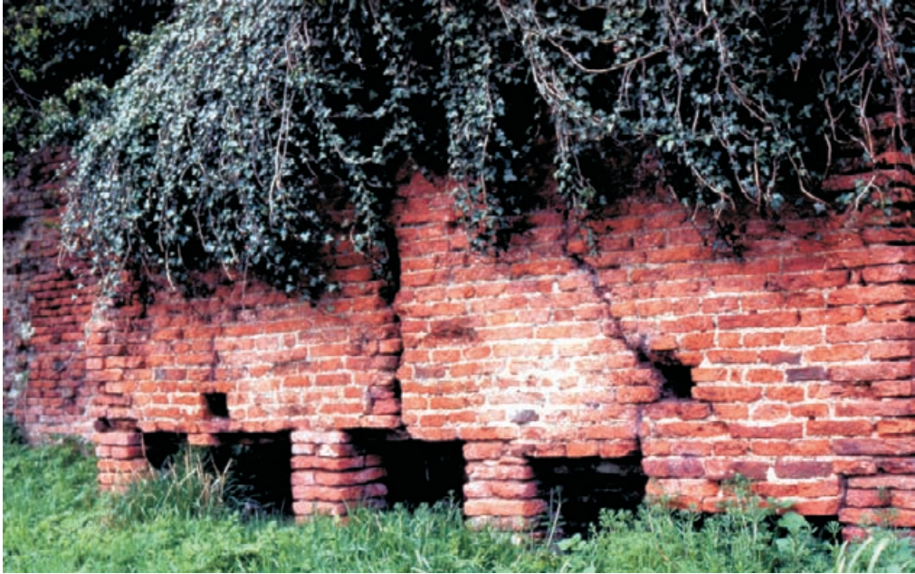
Figure 6.7 The late fifteenth/early sixteenth century brick precinct wall of a monastery, with its moat, now generally dry but seasonally wet, showing settlement fractures with brick underpins, mortar deterioration and luxuriant ivy growth. The wall is host to bats and masonry bees, sometimes to owls, and frogs, slow worms and newts are sometime inhabitants of the moat. The Conservation Management Plan includes recommendations for the management and maintenance of the site which must embrace and balance the preservation needs of the historic fabric and the needs of the natural inhabitants and their environment.
