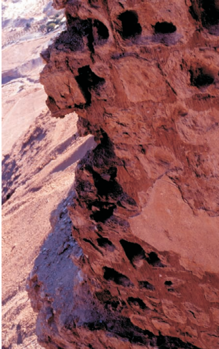
Figure 10.18 The northern wall of the caldarium showing the fragile, egg crate-like form of the weathered stones (top centre) where they are not protected by plaster (bottom right).
