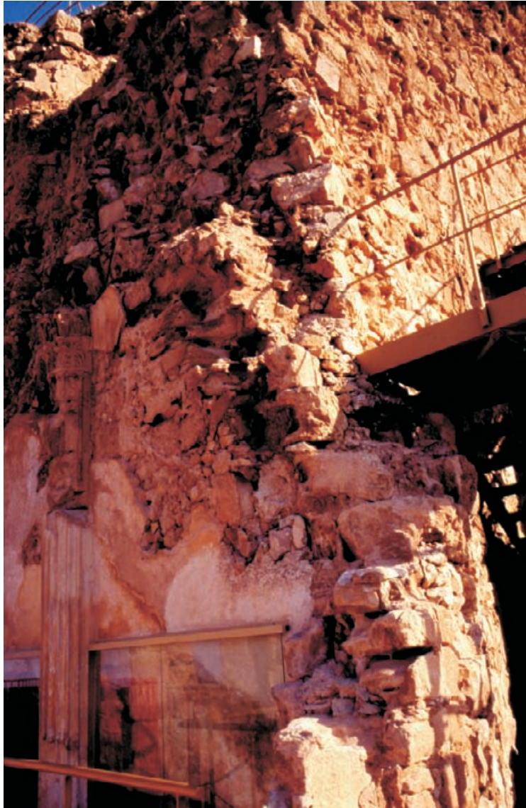
Figure 10.17 The middle terrace northern wall, showing at its base the coloured plasters of the tridinium on the lower terrace. The fragile condition of both rock and stones can be seen.
