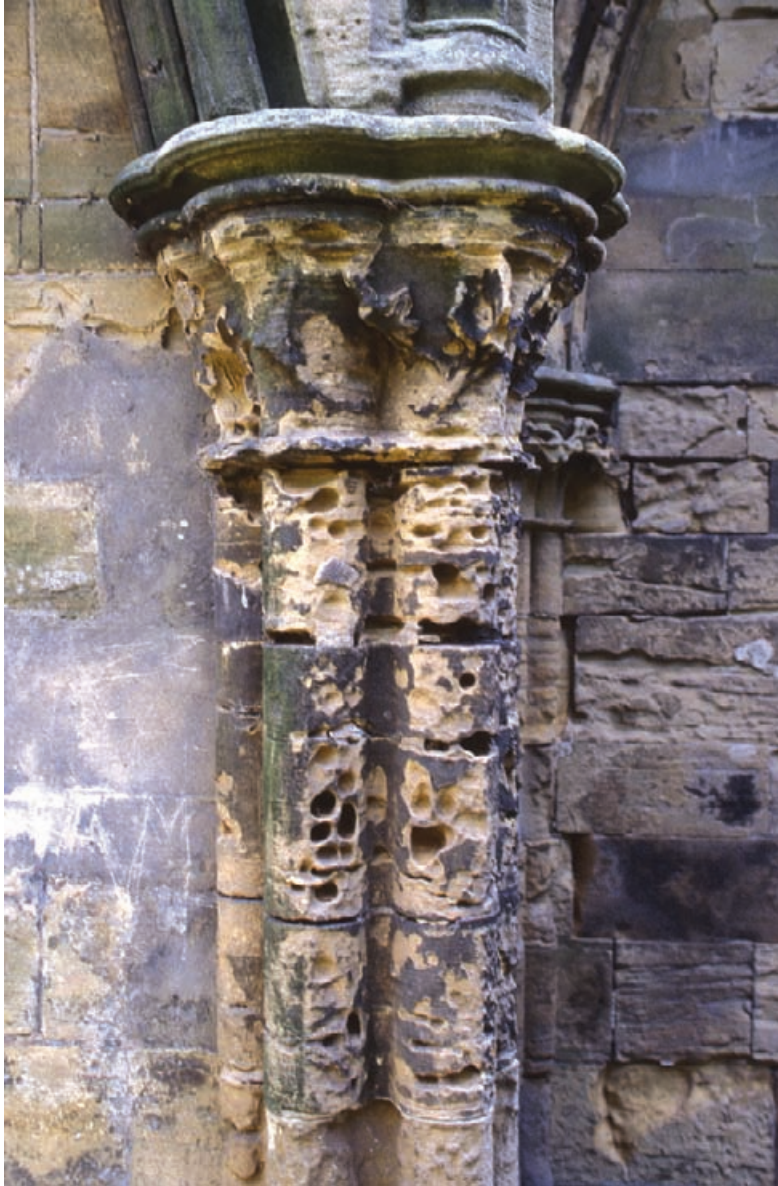
Figure 3.8 Alveolar weathering of White Mansfield sandstone. The age, weathering, and lack of maintenance and repair over the lifetime of a ruin are often associated with advanced patterns of decay.
