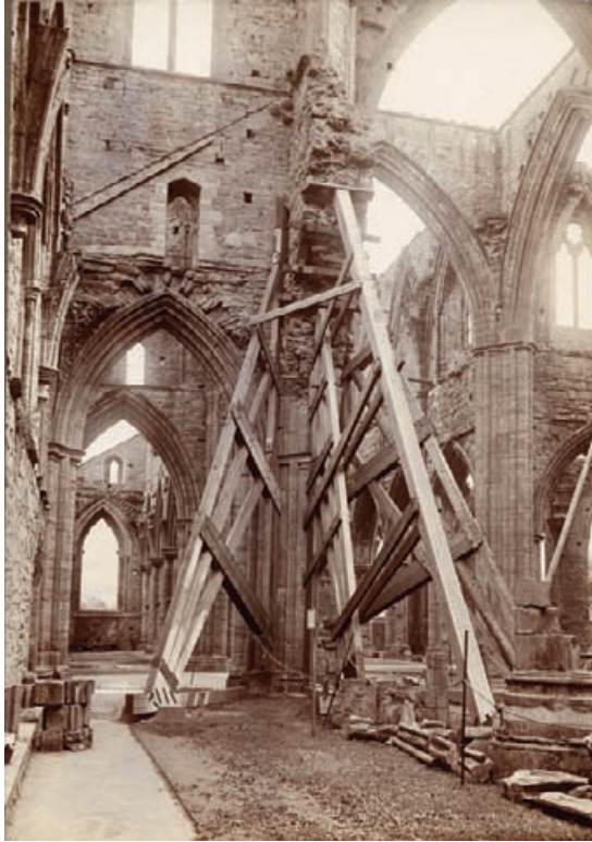
Figure 4.4a Tintern Abbey - North west pier showing timber shoring under broken nave arcade. This overhanging masonry was repaired in the manner shown in Figure 4.4b.
