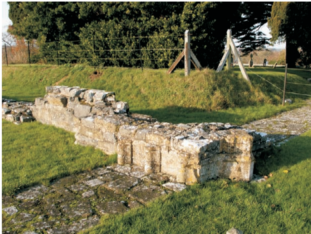
Figure 9.3 (b) The use of different forms of masonry consolidation and capping at Muchelney Abbey to distinguish between building phases of construction illustrating another early house style of presentation (see page 251).
