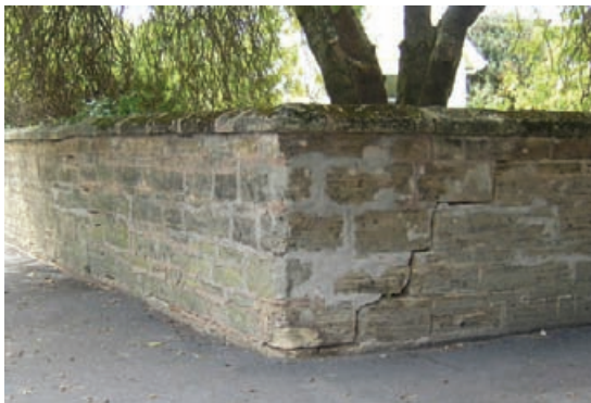
Figure 2.26 Tree root lift.
