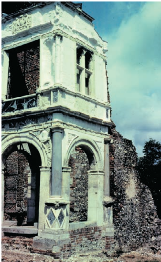
Figure 4.75 The conservation work required on Bacon's late sixteenth century entrance porch included mortar repairs, stainless steel and ceramic stitches to hold edge bedded columns together, conservation and replication of Roman marble, consolidation and surface treatment of a range of decorative stones and consolidation of heavily decayed wood sculpture.
