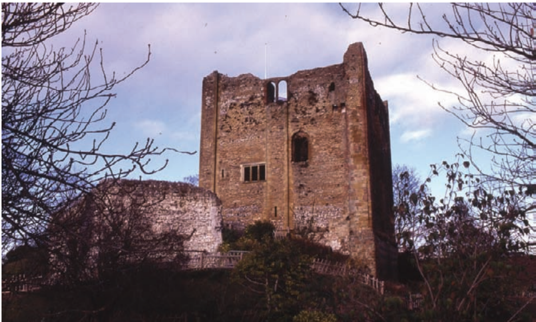
Figure 3.2 The Great Tower at Guildford Castle in Surrey: ruins are often romantic places which create special challenges for the surveyor to leave intact.
