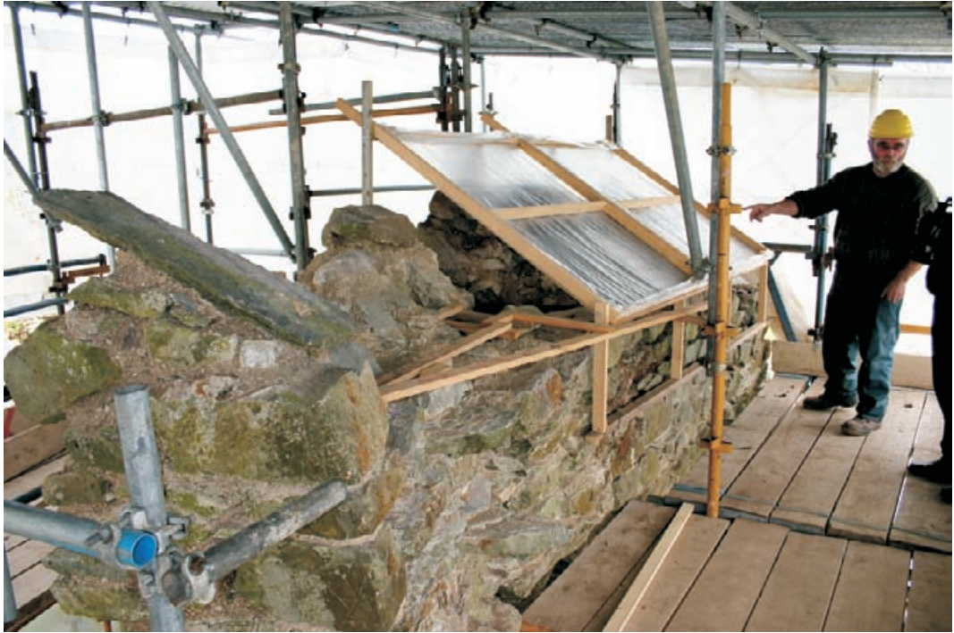
Figure 4.21 Planning frames shown in position for recording wall tops. The frames will need to be capable of repositioning in exactly the same position during the rebuilding process. Note, left, tilestone consolidated in the position found on the wall head.
