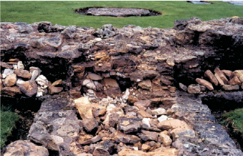
Figure 4.15 Low-lying walls such as this are very vulnerable to frost damage in cold climates and to disruption by visitors anywhere. These walls are ideal candidates for soft capping, following consolidation. Note how hard capping has been placed over unconsolidated core with disastrous results as the capped zone lifts and cracks. Thornton Abbey.
