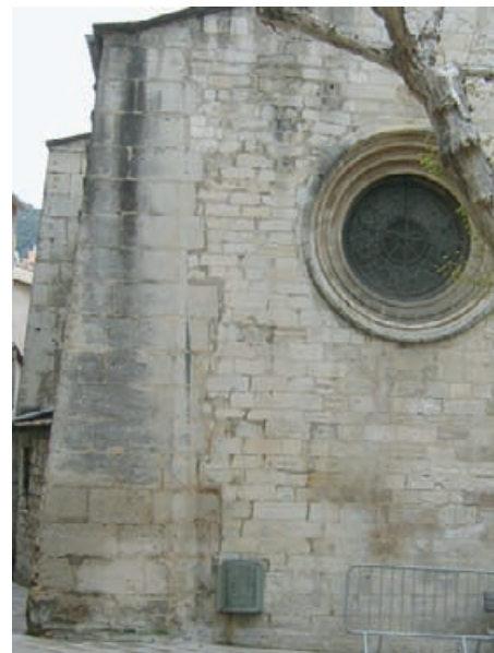
Figure 2.13 Massive added buttress to wall fractured during seismic activity, Manosque, France.
