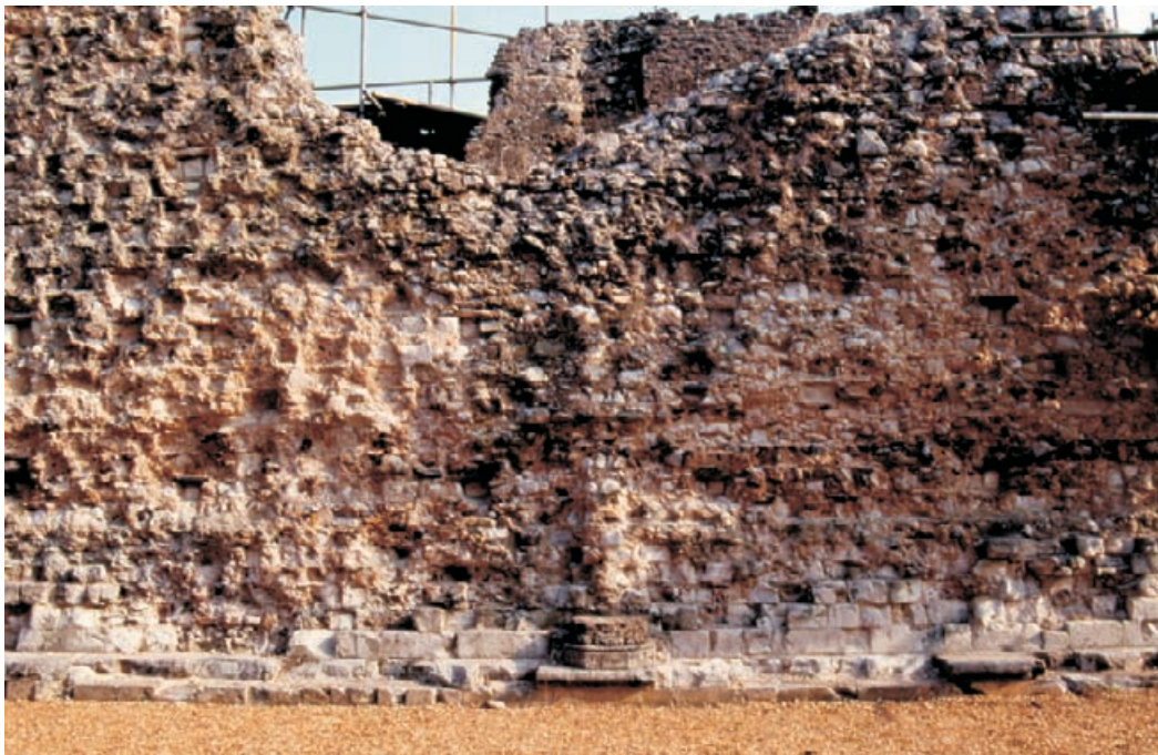
Figure 4.34 Almost all facework has been lost from his medieval composite wall. Only the core provides a record of the stone coursing and other features such as a column and vault springing line. Such core needs careful treatment; in particular, the wall heads must not be so consolidated that they become water-shedding. Either lime-mortared core or a 'soft top' of vegetation should be used. Waverley Abbey.
