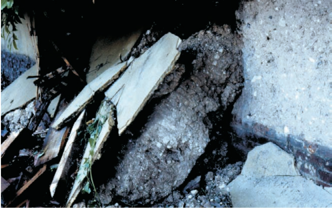
Figure 4.69 The use of a cement rich plaster applied to earth walls is seen here in dramatic failure mode. Cracking of the plaster occurred within 6 months and failure within one year. During its lifetime it held water against the ancient earth wall causing softening and significant losses for the first time in many centuries.
