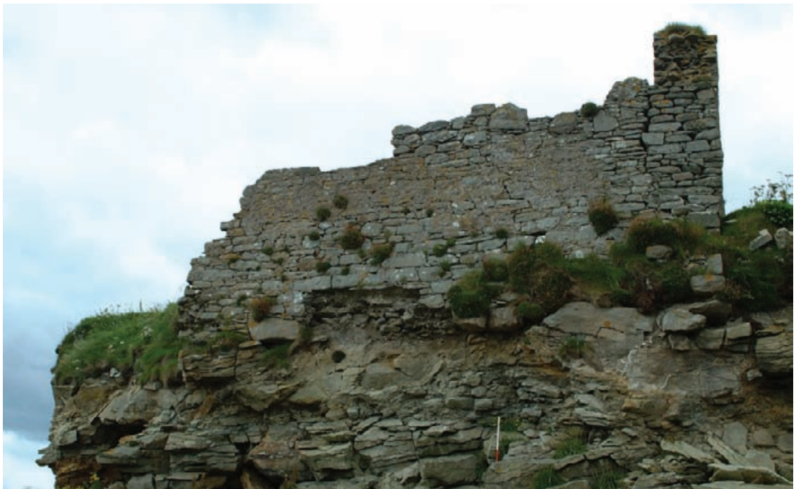
Figure 7.9 Erosion of the sandstone bedrock beneath McSwynes Castle by wave action and corrasion by the boulder/cobble beach element leading to partial collapse of the outer face of masonry.
