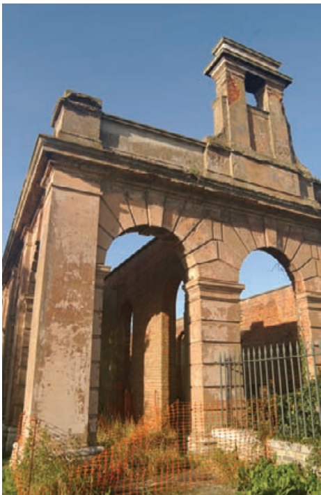
Figure 10.39 Cement stucco used to replicate rusticated masonry is particularly vulnerable to the ruined condition of the building and needs careful maintenance.
