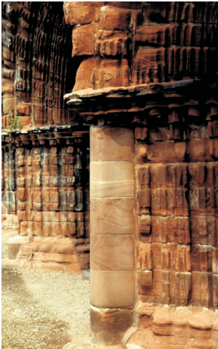
Figure 4.56 Philosophy in place at Furness Abbey. The missing outer orders of the arcade pier have been replaced in a similar red sandstone which provides the necessary structural support for the arch but which is visually rather unsuccessful. The new line of the pier face is too far forward, and has no articulation representing the base and cap. In addition, the course lines of the new stone do not run through to match the original coursing. Some shallow vertical channelling echoing the original roll and hollow moulding would have made it a much better intervention, whilst still remaining an obvious intervention.
