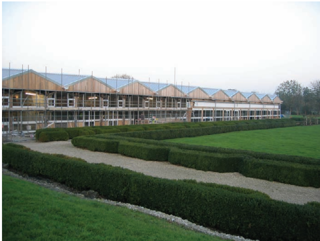
Figure 5.34 General view of the south elevation of the enclosure building at Fishbourne Roman Palace, in the process of modernisation and upgrading (photograph: C. Woolfitt).
