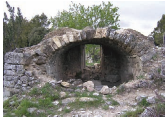
Figure 2.35 Arch close to failure due to spread at springing level.
