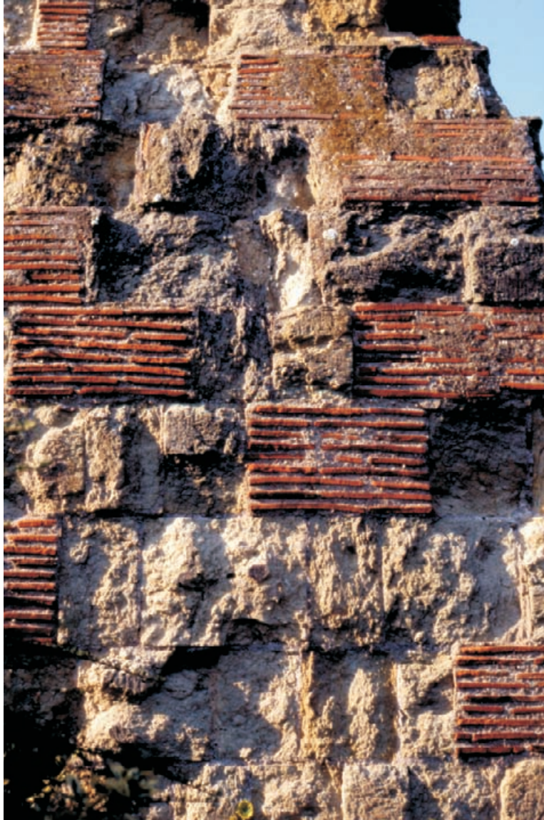
Figure 4.57 Philosophy in place at Guildford Castle. The 1914 period clay tile replacements for decayed stones were once rendered. These repairs were and are unmistakable interventions, which is exactly what was intended.
