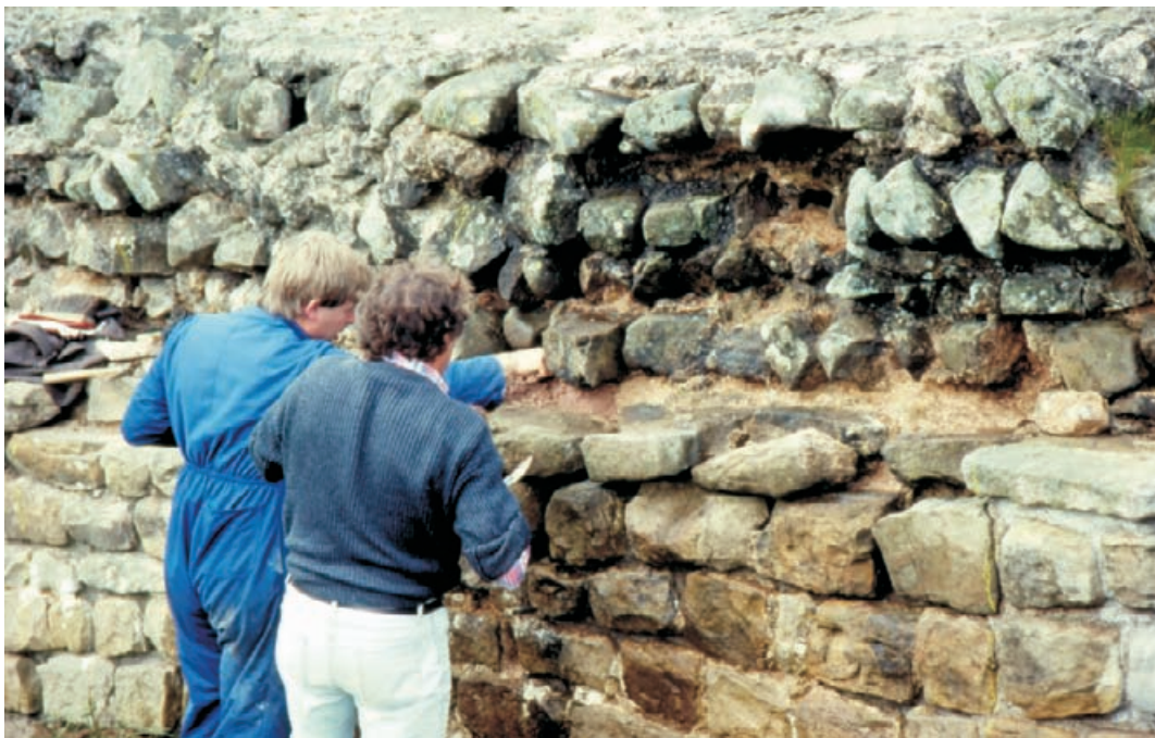
Figure 4.63 Exposed core of Hadrian's Wall with its wall head screed intact. Loss of face stones requires careful consolidation of materials not designed for weathering.
