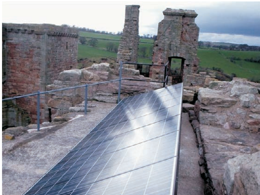
Figure 9.9 Eight photovoltaic panels are sensitively and reversibly sited on top of the remains of the fourteenth century tower and provide general power to a small shop and ticket office. The panels replaced a noisy generator, are fully reversible, and meet government initiatives and green tourism initiatives.
