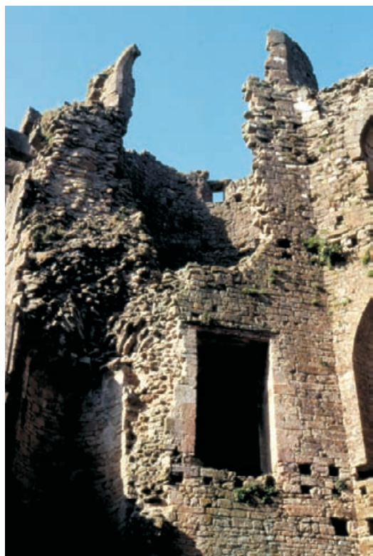
Figure 4.39 View of overhanging high level masonry supported by restraining cramps at Nunney Castle.
