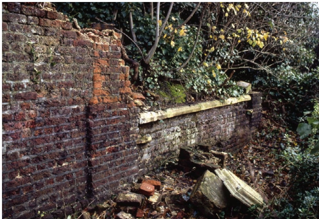
Figure 3.7 Waterlow Park in London: ruined seventeenth century viewing platform with brick piers, part of a formal garden landscape. Lack of maintenance to the structure and surrounding garden led to the partial collapse of the wall and loss of the wrought iron screen and decorative sculpture.
