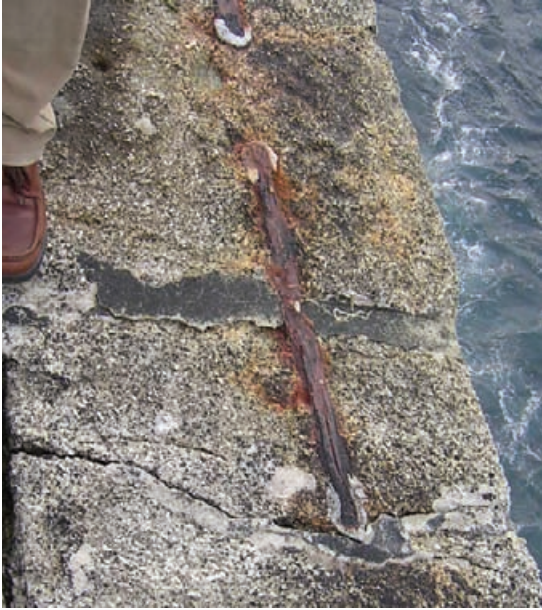
Figure 2.56 Granite cracking and steel straps, Cornwall.
