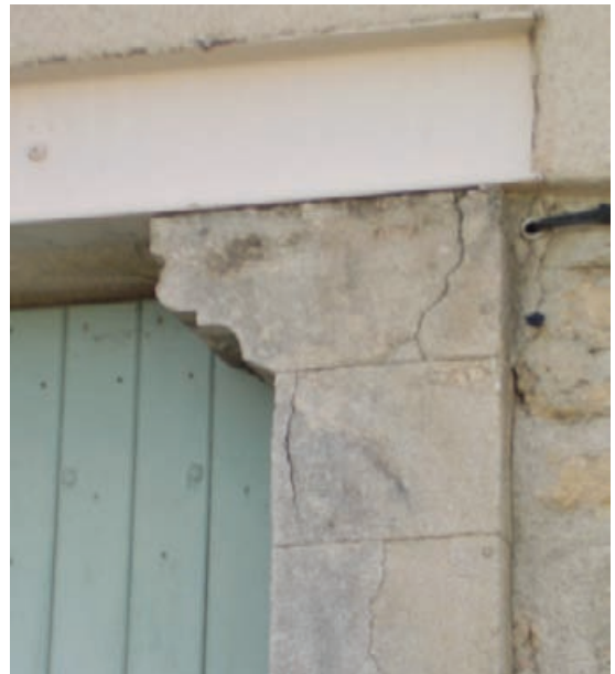
Figure 2.58 Cracked masonry related to corrosion of unmaintainable steel beam insertion, Provence.
