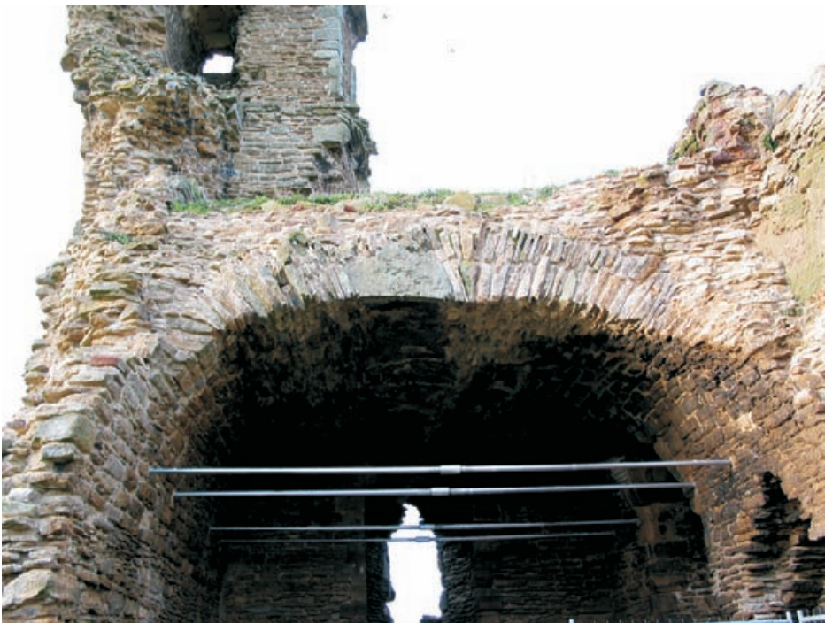
Figure 4.37 Stainless steel torsion bars introduced at the springing line of a broken vault, anchored into the core with pattress plates, to prevent the vaults spreading, fracturing and failing. Sheriff Hutton Castle.
