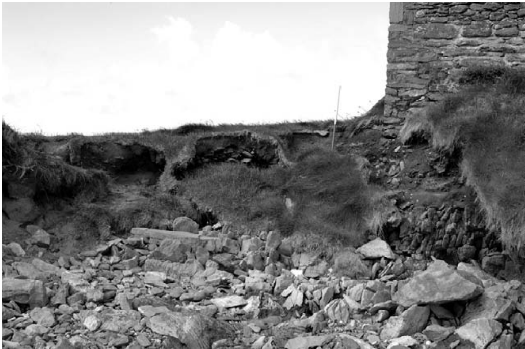
Figure 7.4 Erosion is now beginning to undermine the corners of the tower, with the cobble beach corrodng the cills of the principal historic stone entranceway.
