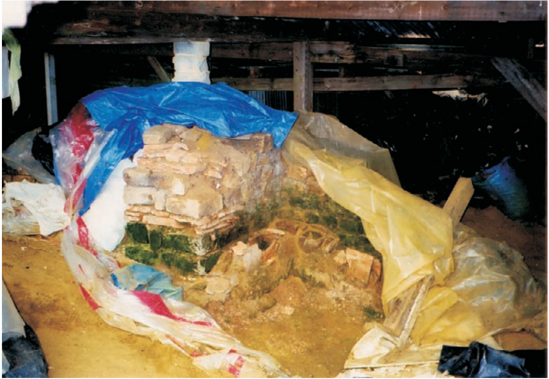
Figure 5.33 Detail of typical condition of masonry remains within the shelter shown in Figure 5.32, with damp conditions, deteriorating and friable surfaces supporting organic growth (photograph: C. Woolfitt).
