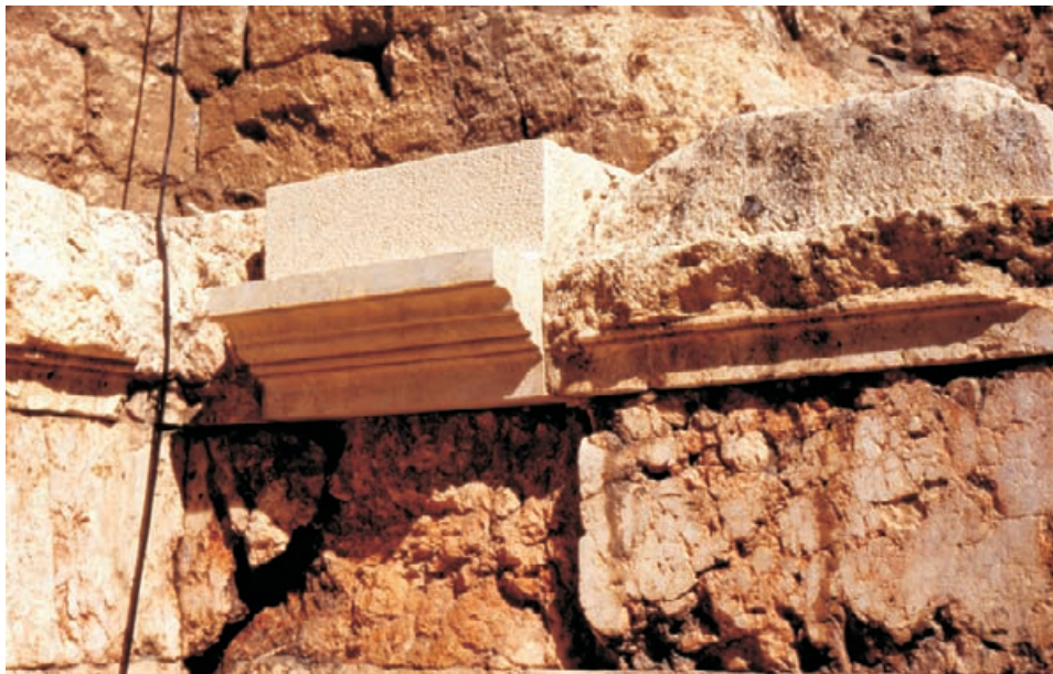
Figure 4.52 This section of Roman cornice has been prepared from templates made from a complete stone found in excavation. It is set in the wall to fill a gap and to show the original architectural line and detail. Beth Shean Israel.
