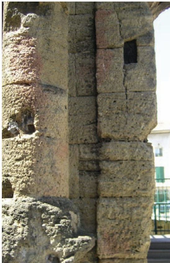
Figure 2.20 Stress cracking of the Roman Theatre at Orange (2).
