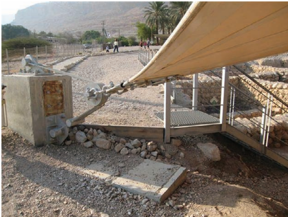
Figure 5.25 Detail of anchor for the Ein Gedi shelter shown in Figure 5.24 (photograph: Orit Bortnik).
