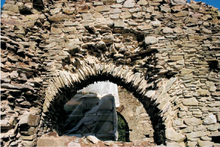
Figure 4.36 Consolidation work completed to a very high ‘as found’ standard with corbelled arch rings and corbelled out core. Complete stability has been achieved through the use of judicious masonry techniques and materials without any engineering device. Mourne Abbey.
