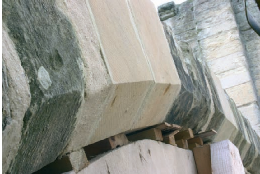
Figure 8.6 The distorted and failing arch of a medieval flying buttress has been temporarily shuttered to its distorted profile. For it to perform satisfactorily the curvature of the arch needs to be restored but instead a muddled hybrid, partly distorted, partly 'corrected' has been created resulting in a confused assembly of new and old stones.
