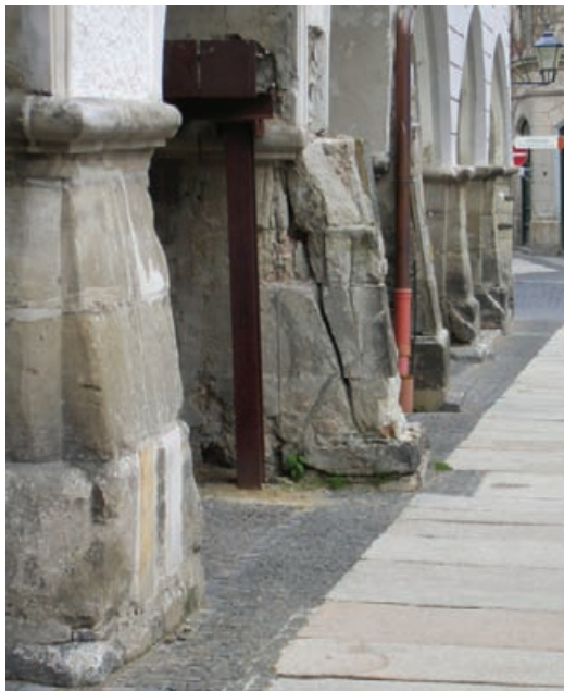
Figure 2.29 Shear cracks in buttress of leaning wall base.
