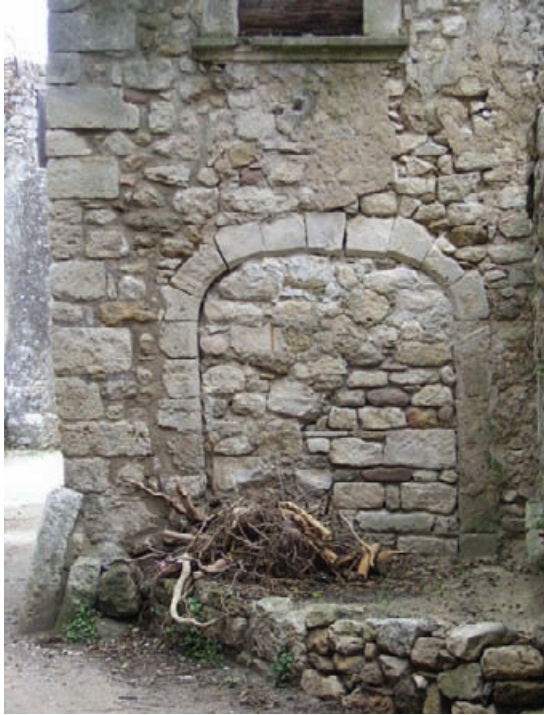
Figure 2.36 Arch close to failure moving towards the area offering least lateral support.
