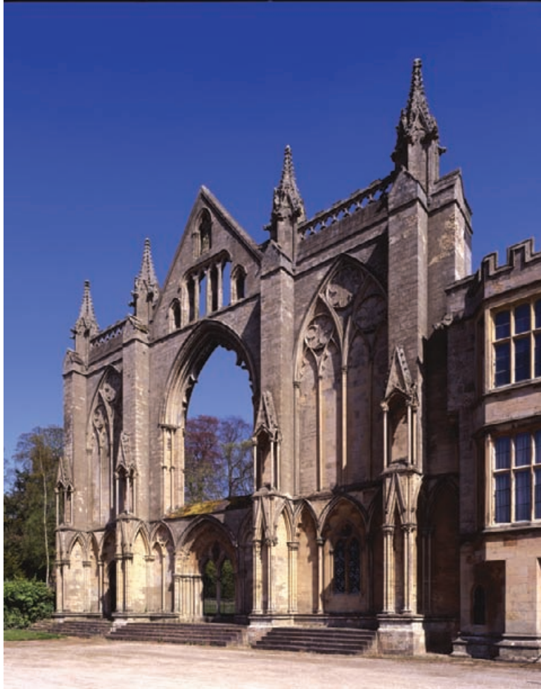
Figure 3.6 Newstead Abbey: the standing remains of the West Front of the Priory Church. The wall is now exposed on both the external and the internal elevations, increasing the potential for rainwater ingress and decay. Carefully considered and well-executed conservation work is required to reduce the maintenance burden, but maintenance and inspection levels of the masonry will always be comparable to, or exceed, those of a building with protective elements still in place.
