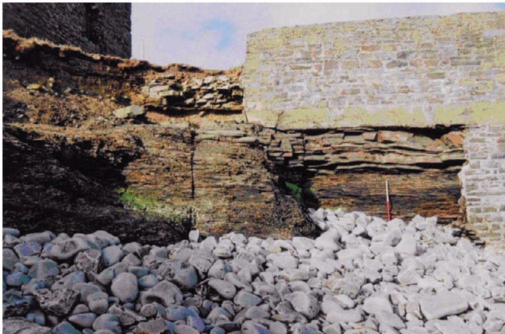
Figure 7.11 Erosion tends to become focused at the edges of coastal protection works and other masonry surfaces. Here the protective bawn wall of Carrigaholt Castle, recently repaired, is again under threat as erosion tunnels around behind the wall.
