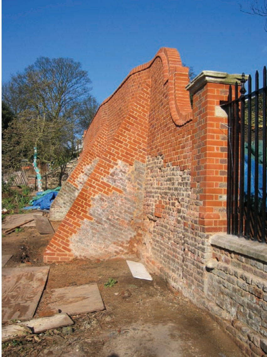
Figure 3.10 Waterlow Park: the lower terrace wall following conservation and repair. Condition survey had determined that the long-term survival of the wall was dependent on reinstating the missing wall head to shed rainwater and protect the brickwork below, but other significant benefits included improved legibility of the structure and enjoyment by the visiting public.
