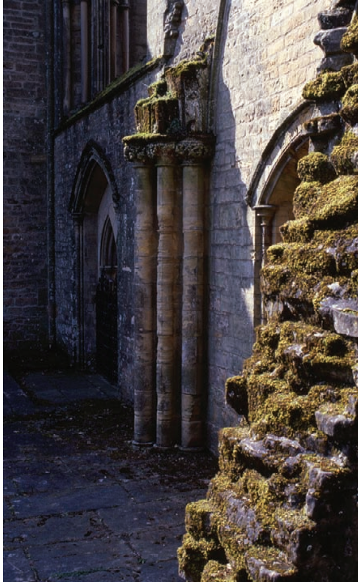
Figure 3.5 The West Front of the Priory Church, Newstead Abbey, Nottinghamshire: where protective roof coverings have been lost and cannot be reinstated, the ruin will often require more frequent monitoring and maintenance than protected elements.
