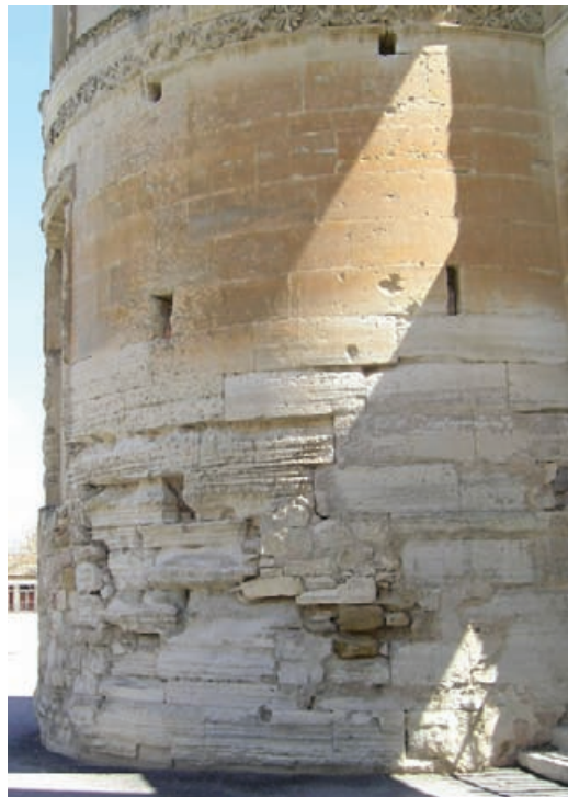
Figure 2.16 Frost damage in saturation zone created by fallen rubble.
