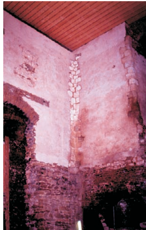
Figure 10.13 Internal view of plastered principal floor level with boarded soffit of new roof, prior to construction of new floor at level of base of new plaster.
