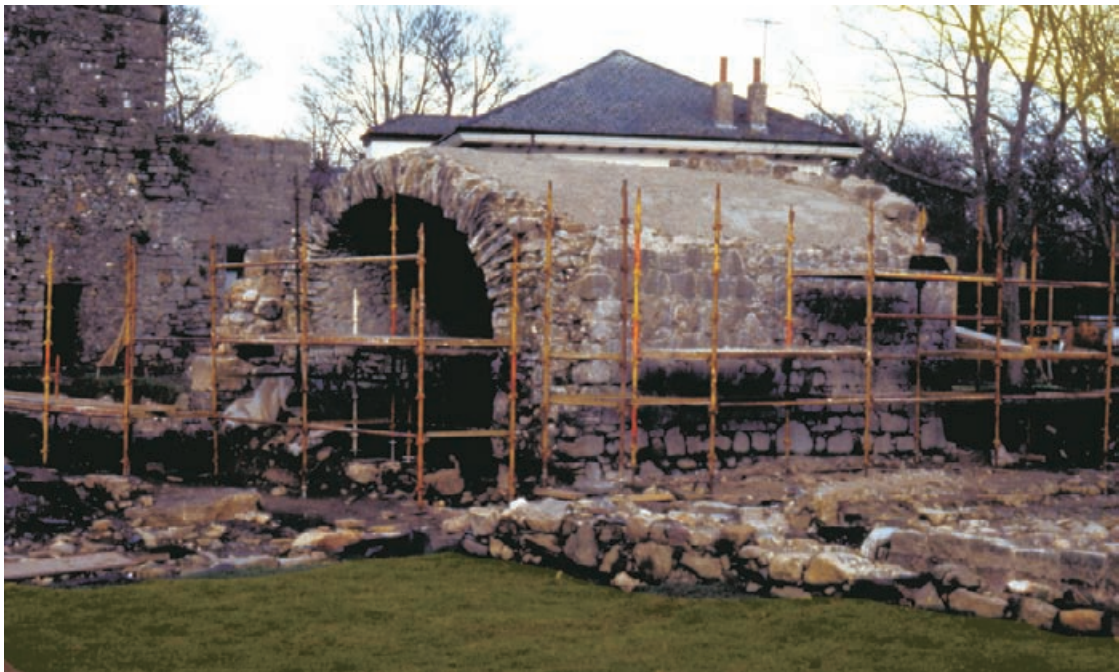
Figure 4.31 The Chapter House vault consolidated and prepared with a hydraulic lime-based screed.
