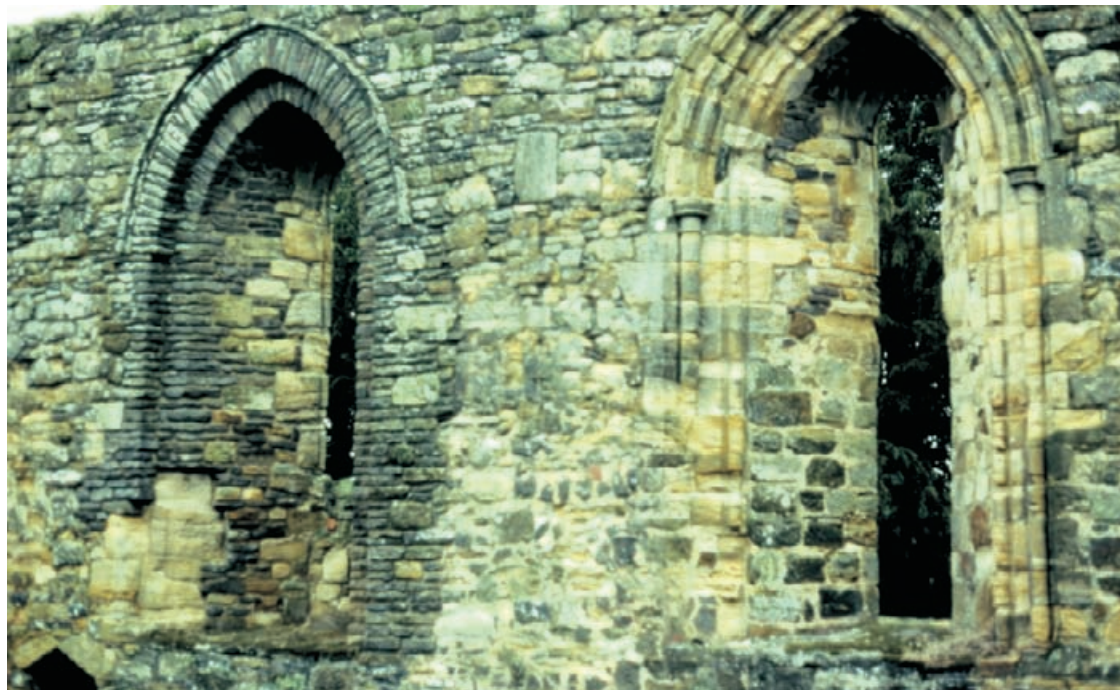
Figure 4.55 Philosophy in place at Battle Abbey, Sussex. In the 1920s the left hand window head and masonry on each side were rebuilt. To distinguish the rebuild from the original, seen on right, the stones were roughly shaped voussoirs and jambs which recreate the scale and design of the original but remain permanently distinguishable from it. This illustrates a typical Society for the Protection of Ancient Buildings approach of the time.
