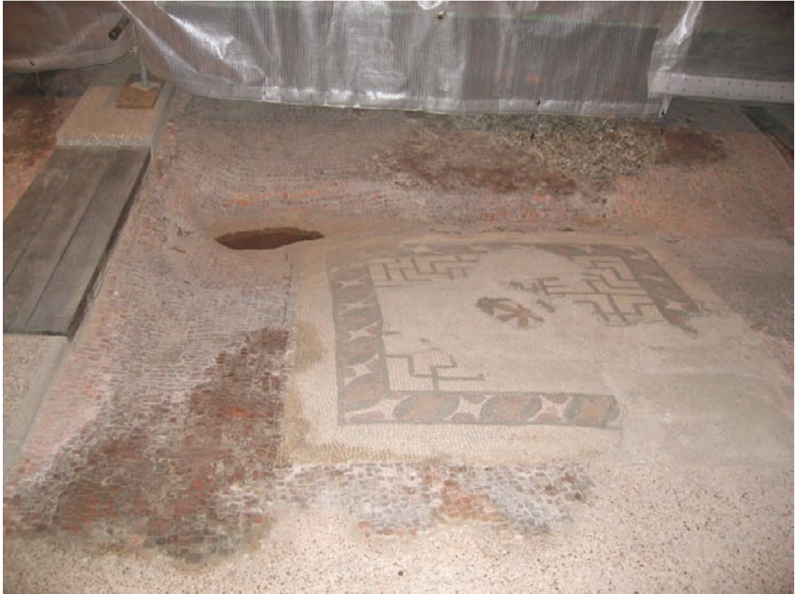
Figure 5.35 Detail within the enclosure building at Fishbourne, with groundwater ponding on the mosaic surface and causing staining (photograph: C. Woolfitt).
