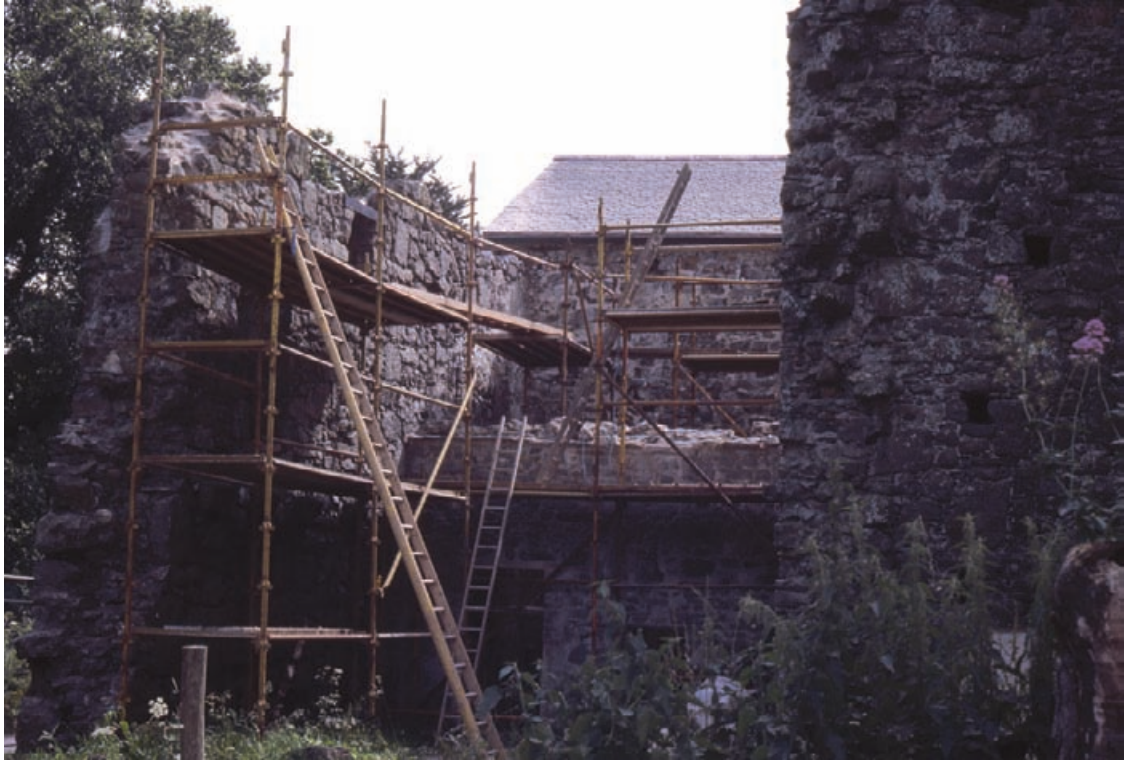
Figure 3.14 Rushen Abbey on the Isle of Man. Access scaffolding should be considered as a means of providing close access for a condition survey. The closer the access, the greater degree of accuracy and certainty that can be achieved by condition survey.
