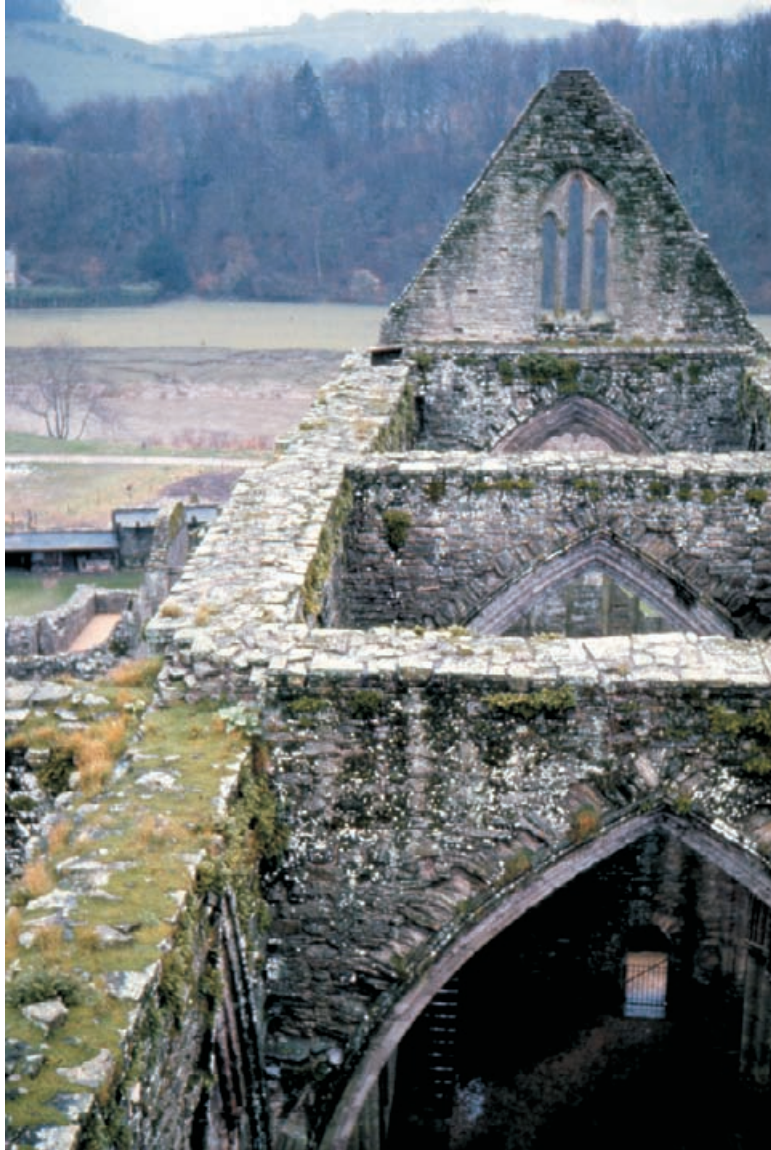
Figure 6.10 Wall tops at Tintern Abbey showing formation of grass and bryophytes in the foreground and biocide-treated surfaces beyond.
