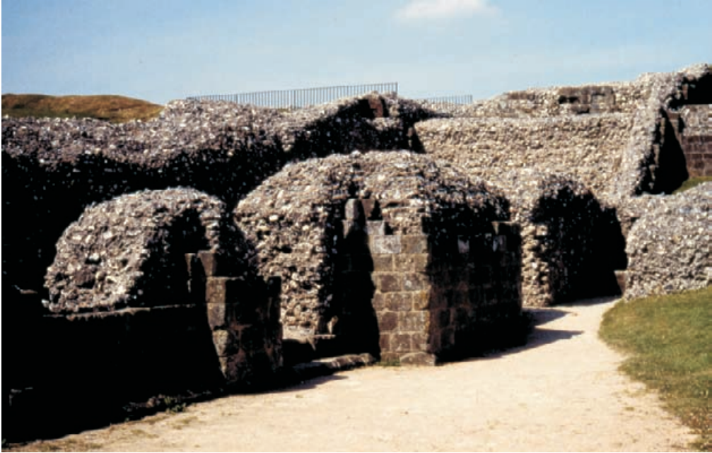
Figure 4.14 Early form of cement-based mortar and flint capping in large surface areas. These attempts to throw water off the wall head have the undesired side effect of taking water into the core through cross-cracking, where it remains trapped. Visually the core work is too far forward. Old Sarum.
