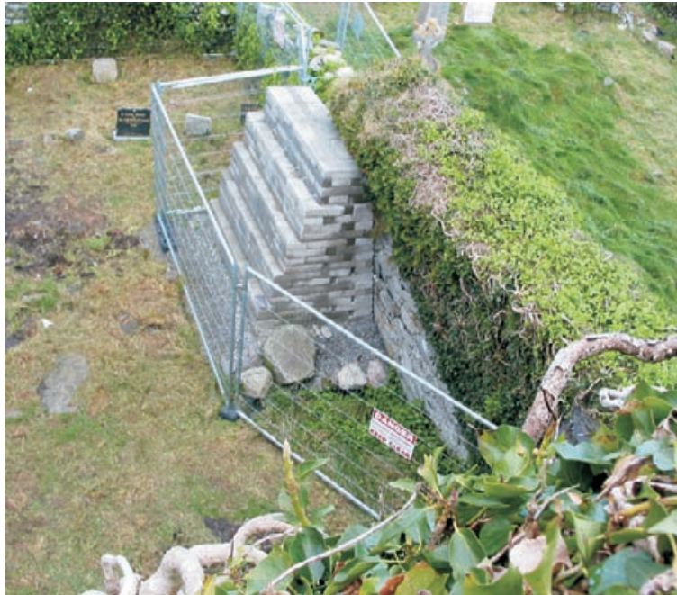
Figure 4.7 Leaning and fractured wall provided with simple temporary buttressing of concrete blocks, and ringed with security fencing. Myross Church, Ireland.
