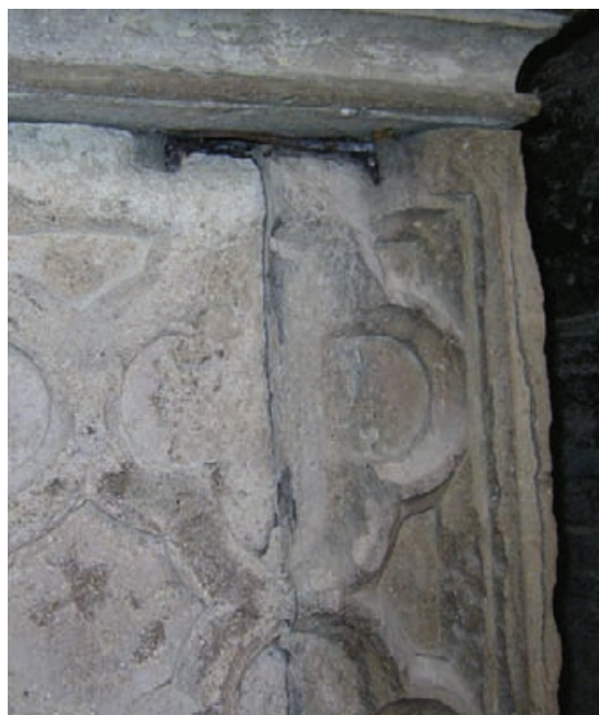
Figure 2.50 Corrosion damage from medieval iron cramps.
