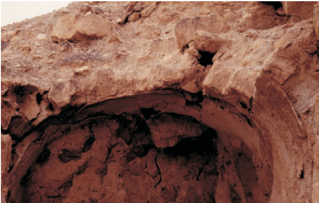
Figure 10.28 Detail of the broken and freshly damaged edge of the frigidarium vault, showing its extreme fragility.
