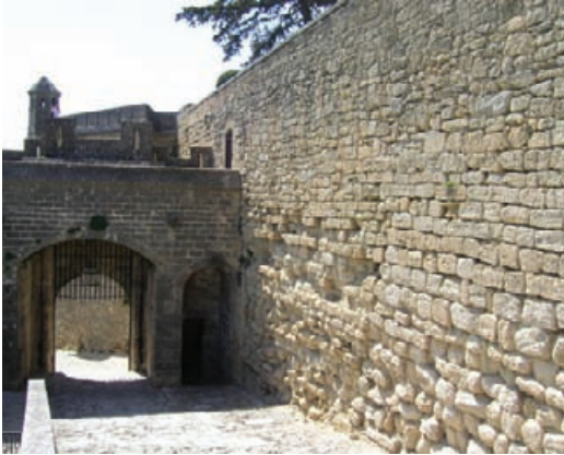
Figure 2.17 Frost damage related to the creation of an eighteenth century terrace behind an existing bastion wall.
