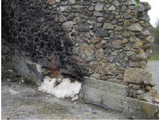
Figure 2.59 Undermined wall and collapse.
