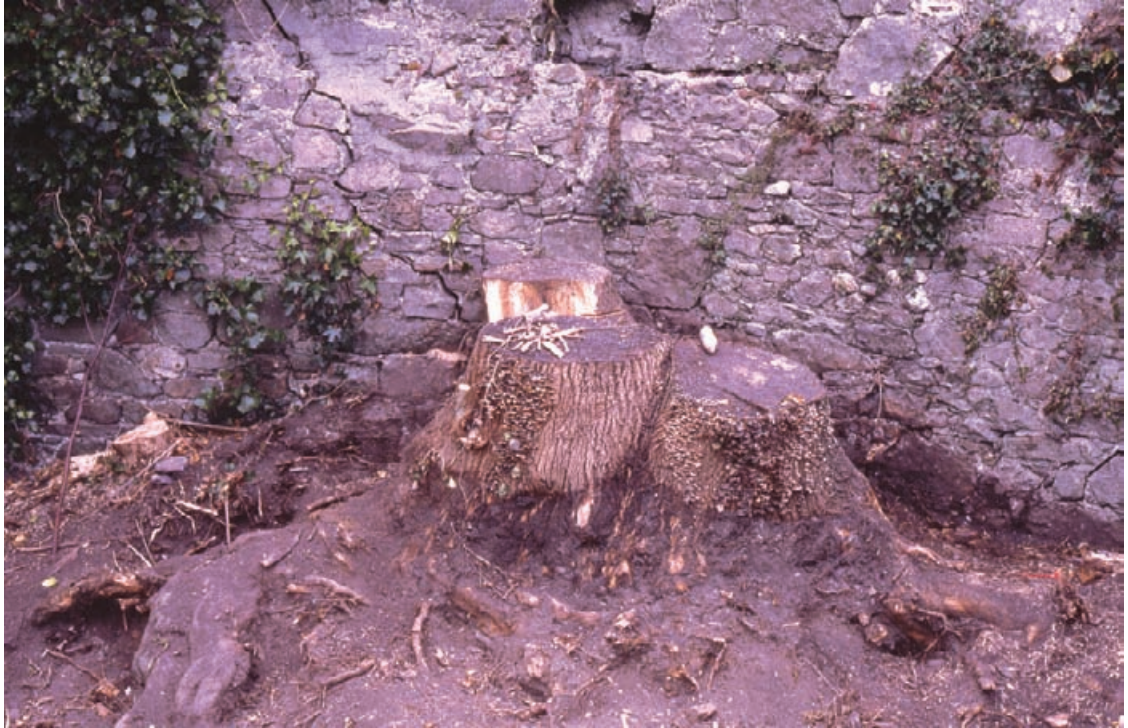
Figure 3.11 Detail of masonry wall at Rushen Abbey on the Isle of Man. Invasive plant growth should only be removed from the monument under the supervision of the conservation architect or surveyor to avoid further damage.
