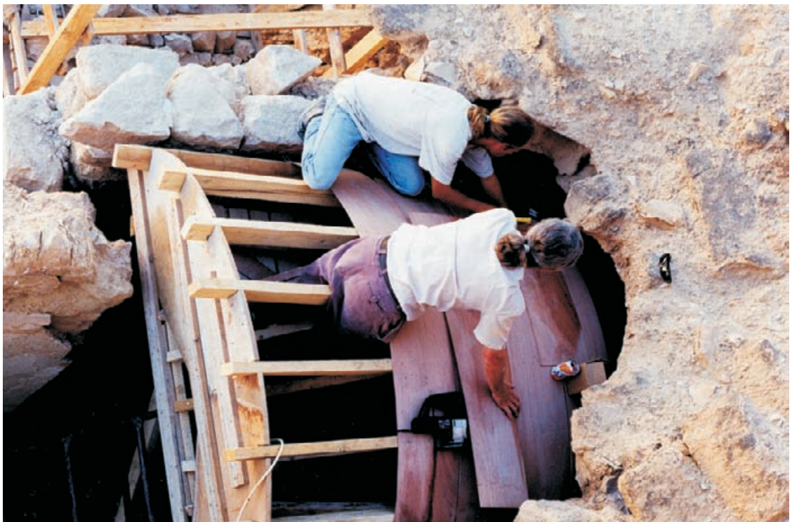
Figure 10.31 Completed form work seen against the raised eastern wall of the frigidarium.
