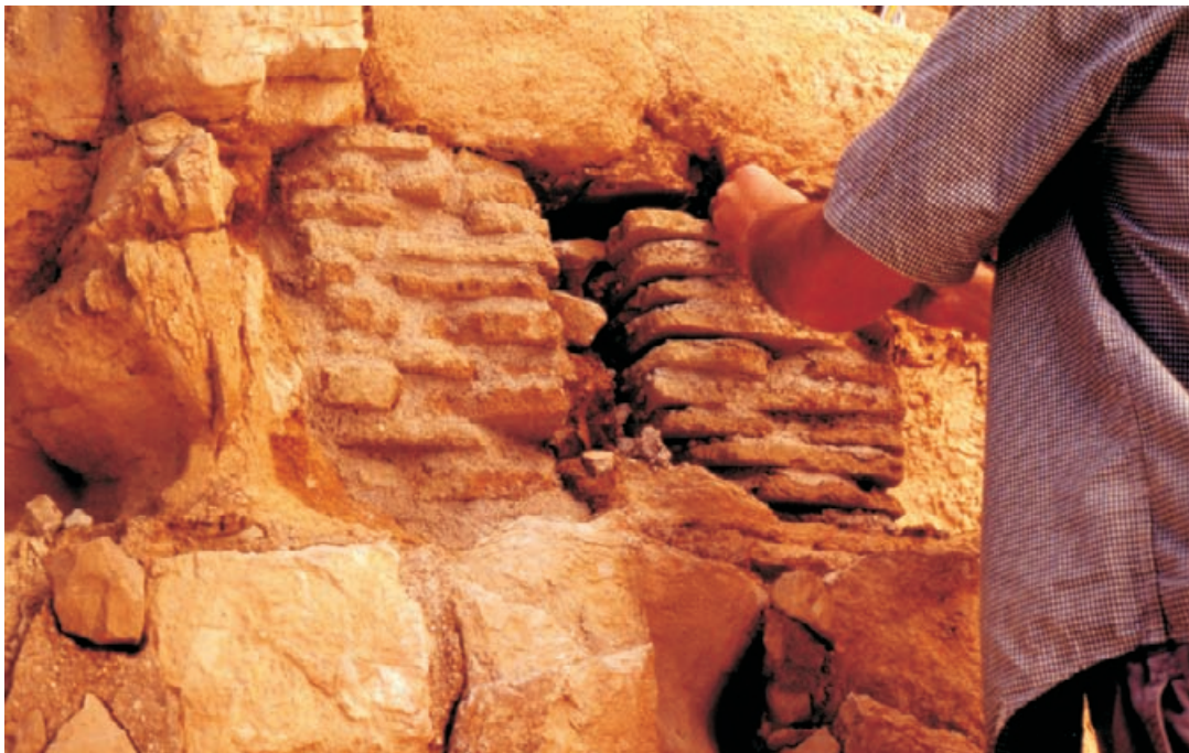
Figure 10.19 Repair of the cavernously decayed stones of the Northern Palace was carried out using “tiles” cut from salvage, weathered stone bedded in pozzolanic lime mortar. Each stone was repaired individually. Joints were packed with mortar and stone in the final stages. The split faces of the tiles blend comfortably with the rough, weathered texture of the surviving masonry and are quickly coloured by the mud washing over the mountain during rainfall. Repaired stones are always easily identifiable at a 2 metre range.
