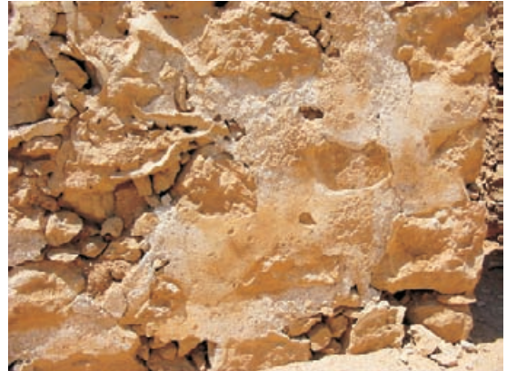
Figure 4.71 Polished Herodian plaster. Only a small percentage of plaster survives within a white cement frame which had been mistakenly used to hold the plaster in position. At the top of the picture only the cement frame survives.
