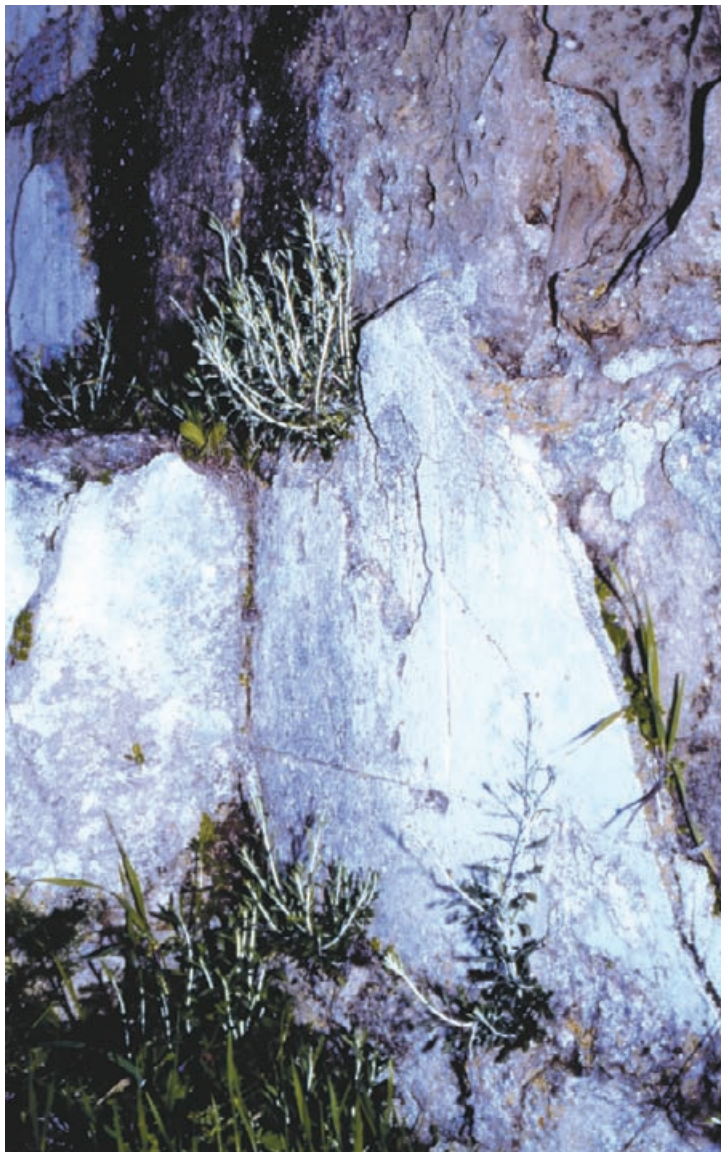
Figure 5.10 Wall plaster, lined out in imitation of ashlar, with detachment caused by the combined effects of vegetation and exposure to weather (photograph: C. Woolfitt).
