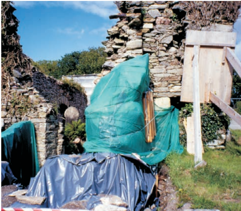
Figure 4.9 Temporary protection and insulation of masonry against rain and frost and temporary support works, County Cork, Ireland.
