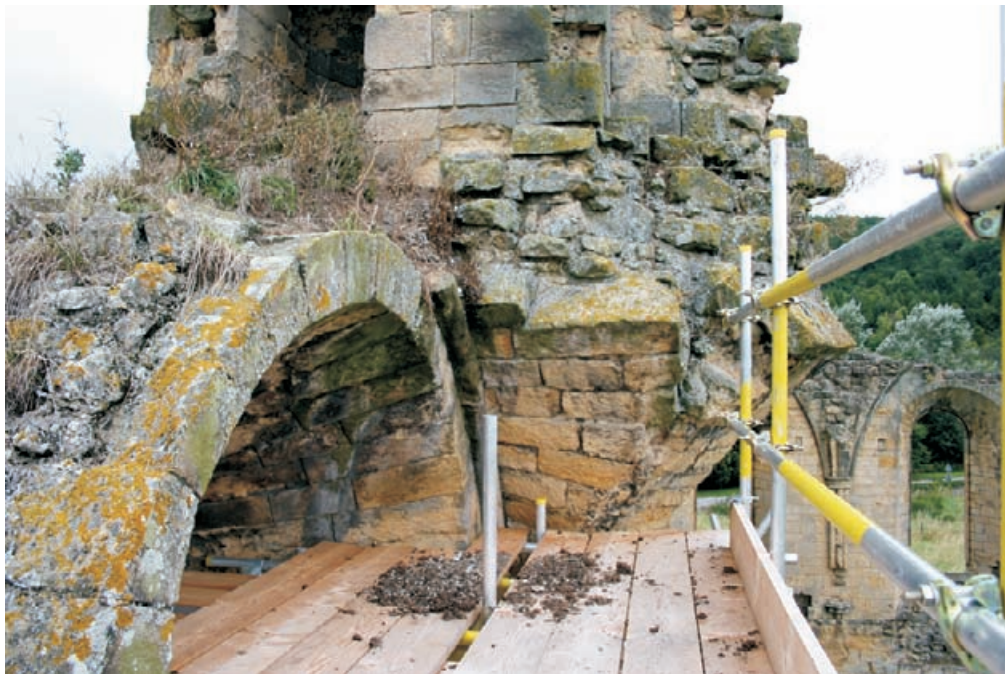
Figure 4.38 Consolidation of overhanging masonry with long restraining cramps set into core work at Byland Abbey.
