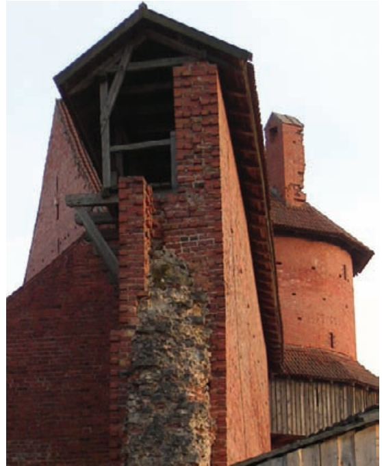
Figure 2.51 Problems with new vitrified brick, Latvia.
