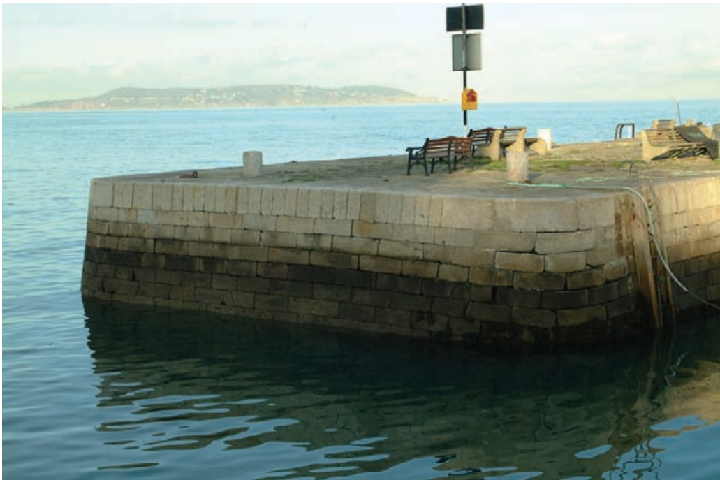
Figure 7.5 Subsidence of the corner of this 19th century granite harbour due to extensive dry jointing and undermining.
