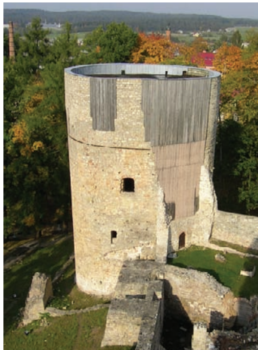
Figure 2.21 Wall head protection of Baltic tower, Latvia.
