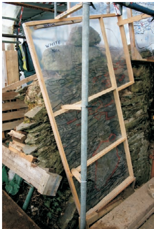
Figure 4.20 The planning frame is shown at the battered angle of the wall top connected to the scaffold tube. Temporary supports in the form of plate and props is shown bottom left.
