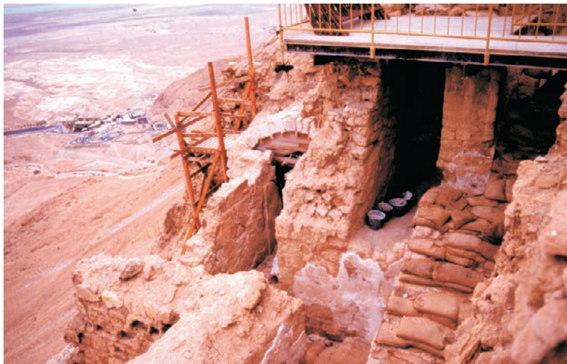
Figure 10.29 View from the lower terrace of the small bathhouse complex during reinstatement of the vault.
