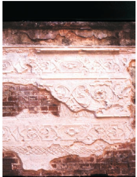
Figure 4.72 Finished consolidation work on decorative fragments of eighteenth century plaster which involved the removal of cement mortar fillets and patches and the substitution of lime putty and ceramic fills. The plaster was cleaned of organic growth using a small hand-held steam gun and was treated with a shelter coat of lime, marble dust and casein.
