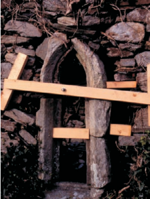
Figure 4.6 Small lancet window largely unconnected to its original masonry has been provided with corset plates bolted through the opening to provide temporary stability.
