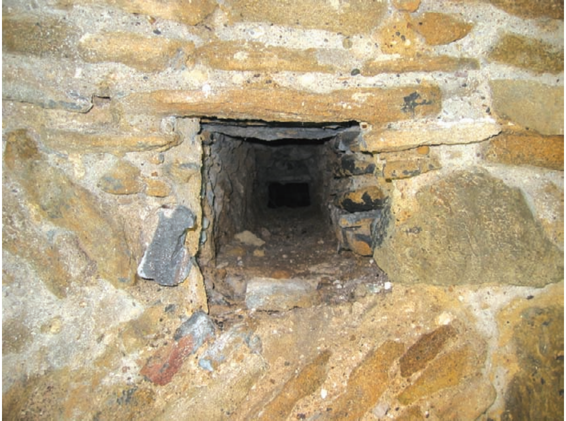
Figure 10.10 Detail of channel for drainage of original roof through east elevation. View of external face which has been unblocked.
