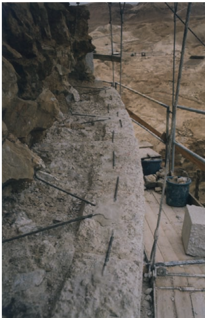
Figure 10.23 Detail of cast block fixing showing stainless steel dog cramps grouted in hydraulic lime and the dovetail fixing method back into the core of the rock. The fill between rock and cast rocks is a weak hydraulic lime and stone aggregate.
