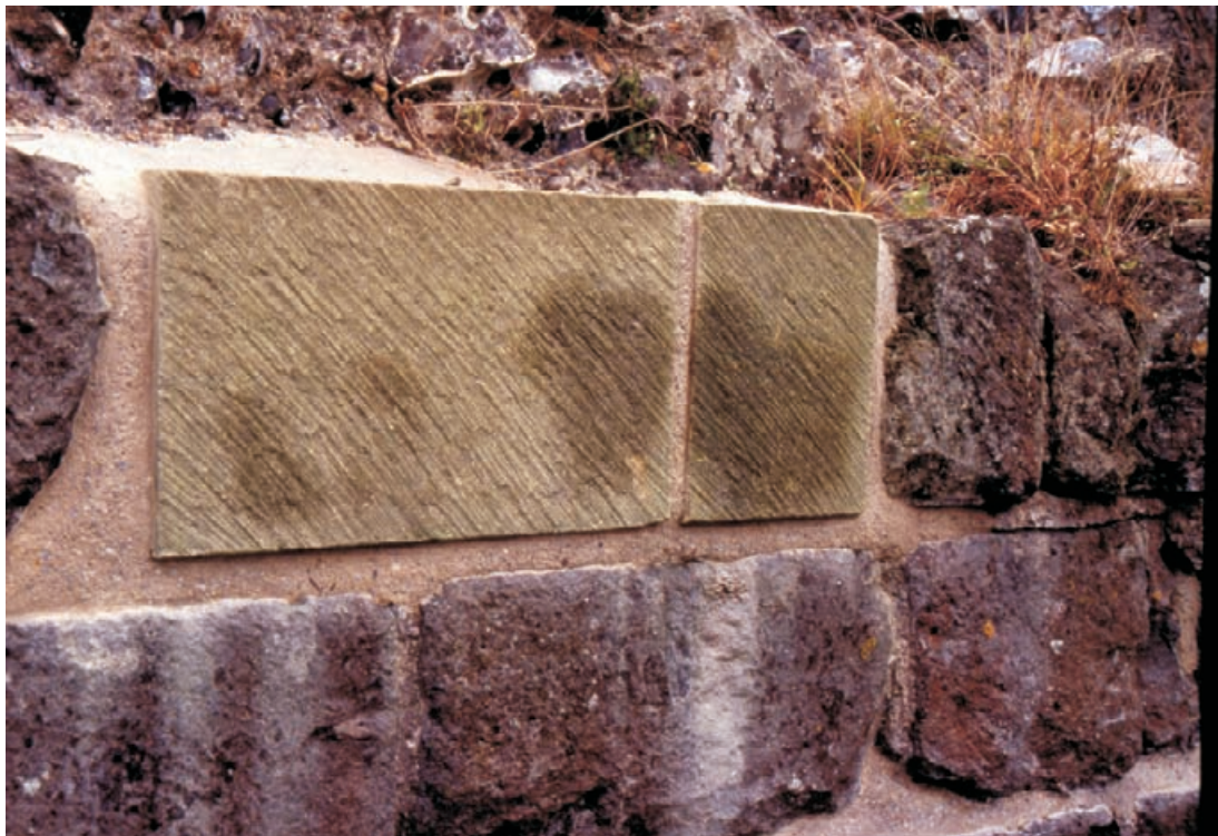
Figure 4.54 New sawn stones are rather more comfortable in a setting of squared ashlars but suffer from arrises which are too sharp and bedding which is out of line. There is also far too much mortar on the top bed, placed in an attempt to provide a weathering. This should be compared with 4.20. New mortar has an unnatural, flat face.
