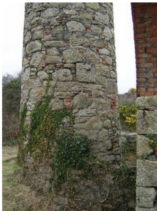
Figure 2.25 Localised erosion related to downstream vortices.
