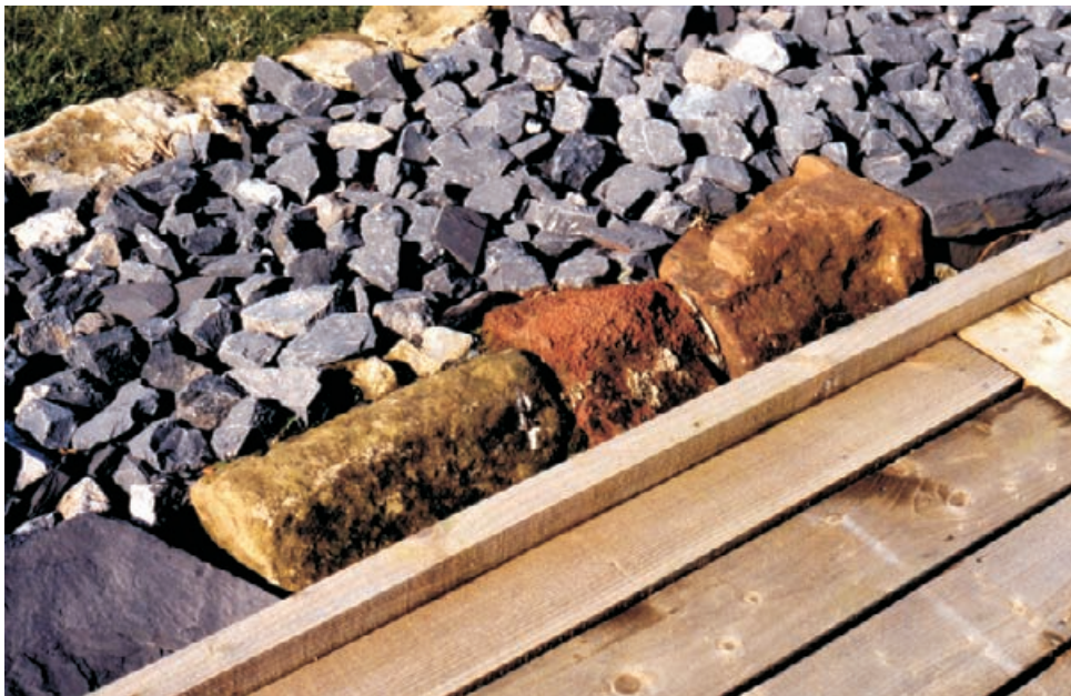
Figure 4.17 Most of this wall lies below original floor levels, with only a few stone facings showing above ground. The fragile core has been covered with geotextile membrane and sand, then set with unmortared limestone scalplings. The result is a free-draining protection which allows the wall line to be clearly read. Loose, large stones discourage visitors from walking on the walls and a more comfortable board walk is provided immediately adjacent to the wall. (see Figure 4.11, C2)
