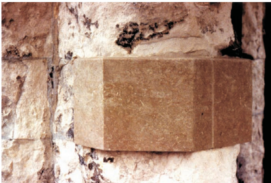
Figure 4.53 This replacement stone has been set in a damaged medieval entrance arch still used by vehicular traffic. The stone is the correct chamfered profile taken from the head of the arch and is placed in its correct line in the jamb. Although the new stone projects from the weathered masonry no mortar weatherings are used; instead the stone has a very slight fall on its top bed and a pencil-round arris. Providing the bedding mortar is deep and well packed this stone will shed water effectively. Guildford, Surrey, UK.
