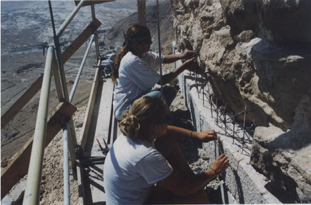
Figure 10.22 Assemblage of cast stones with stainless steel dowels and restraint fixings. The conservators are checking the final position of the face line.
