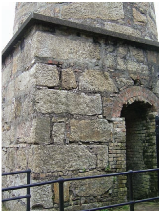
Figure 2.24 Chimney base showing effects of wind vortex erosion.
