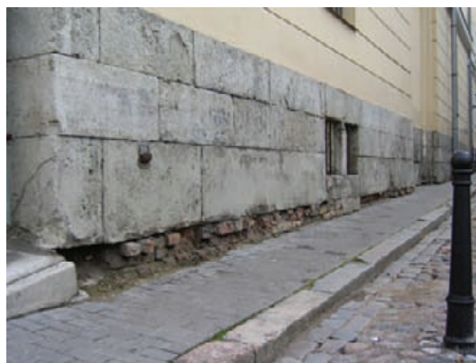
Figure 2.22 De-icing salt damage, Old Arsenal, Riga.
