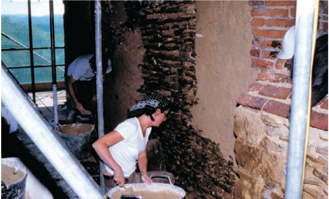
Figure 10.7 Plastering trials were carried out to establish the mortar mix and final appearance and finish.
