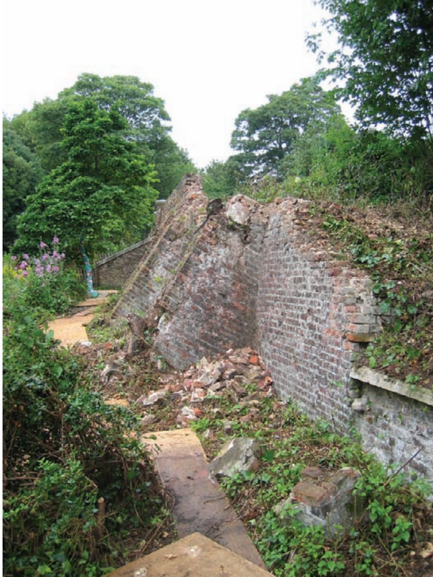
Figure 3.9 Waterlow Park: sixteenth and seventeenth century lower terrace garden walls after removal of invasive plant growth. The upper section of the wall had collapsed.
