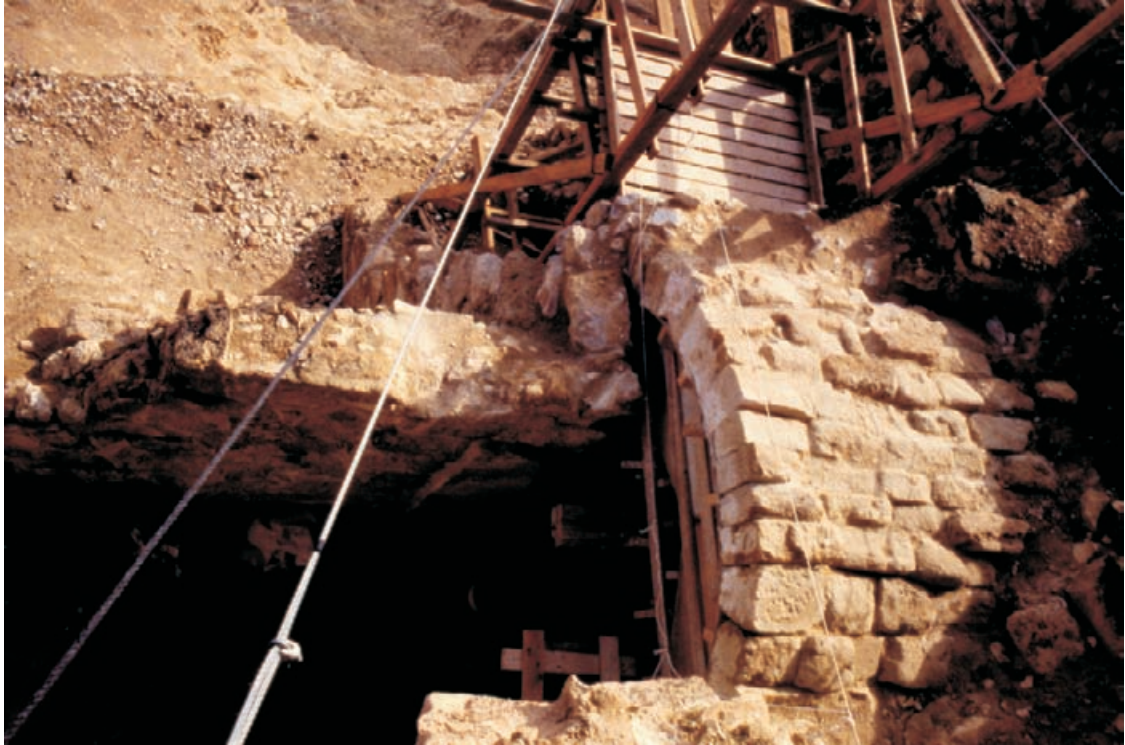
Figure 10.34 Completed vault showing the caldarium and the edge of a precipice beyond.
