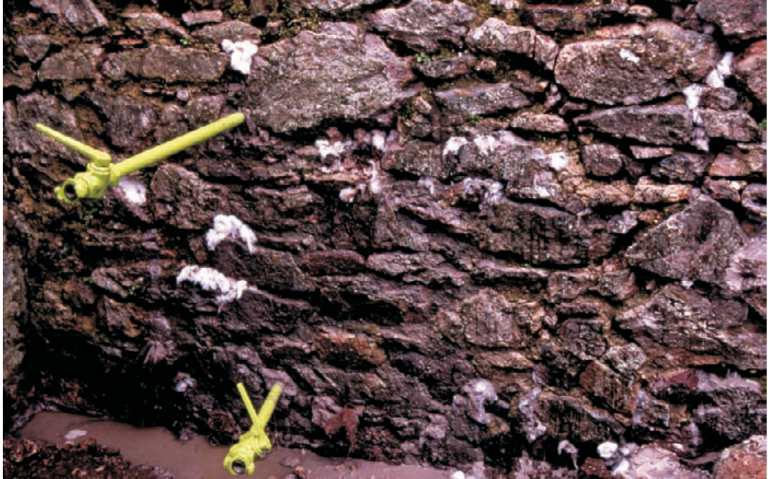
Figure 4.49 Masonry wall showing grout nozzles installed. These can be simply coupled to the grout feed hose.
