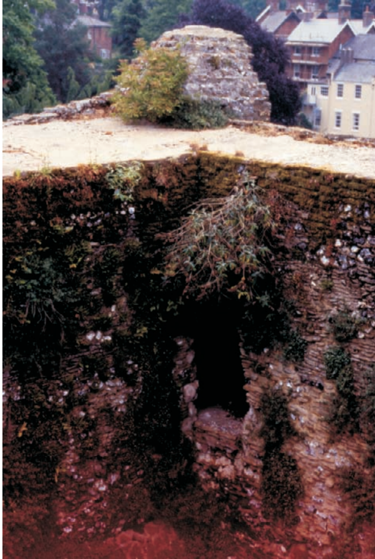
Figure 10.2 The internal south-east corner of the tower at wall-head level, illustrating the extent of plant colonisation and screeds sloping into the tower.
