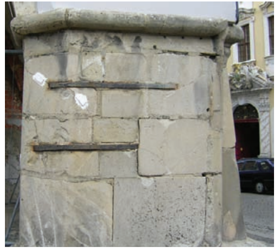
Figure 2.54 Long steel cramp failures showing cracked anchor stones.
