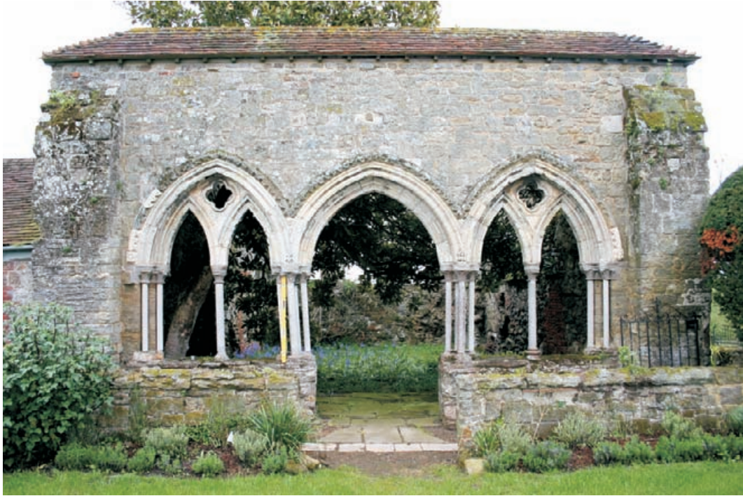
Figure 4.44 Distortion of this medieval arcade is due to multiple causes including loss of restraints and counter-forts during ruination. Most seriously, the low wall on the left of the picture below the twisted cluster of columns is badly fractured. Only the central shaft is making contact with the wall and the arch springing.
