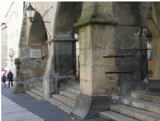
Figure 2.53 Forward lean of masonry façade in Saxony.
