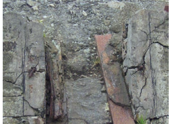
Figure 2.46 Damage caused by rust growth.
