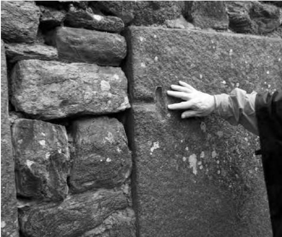
A close-up of the curious block with a keystone cut in a vertical position.
