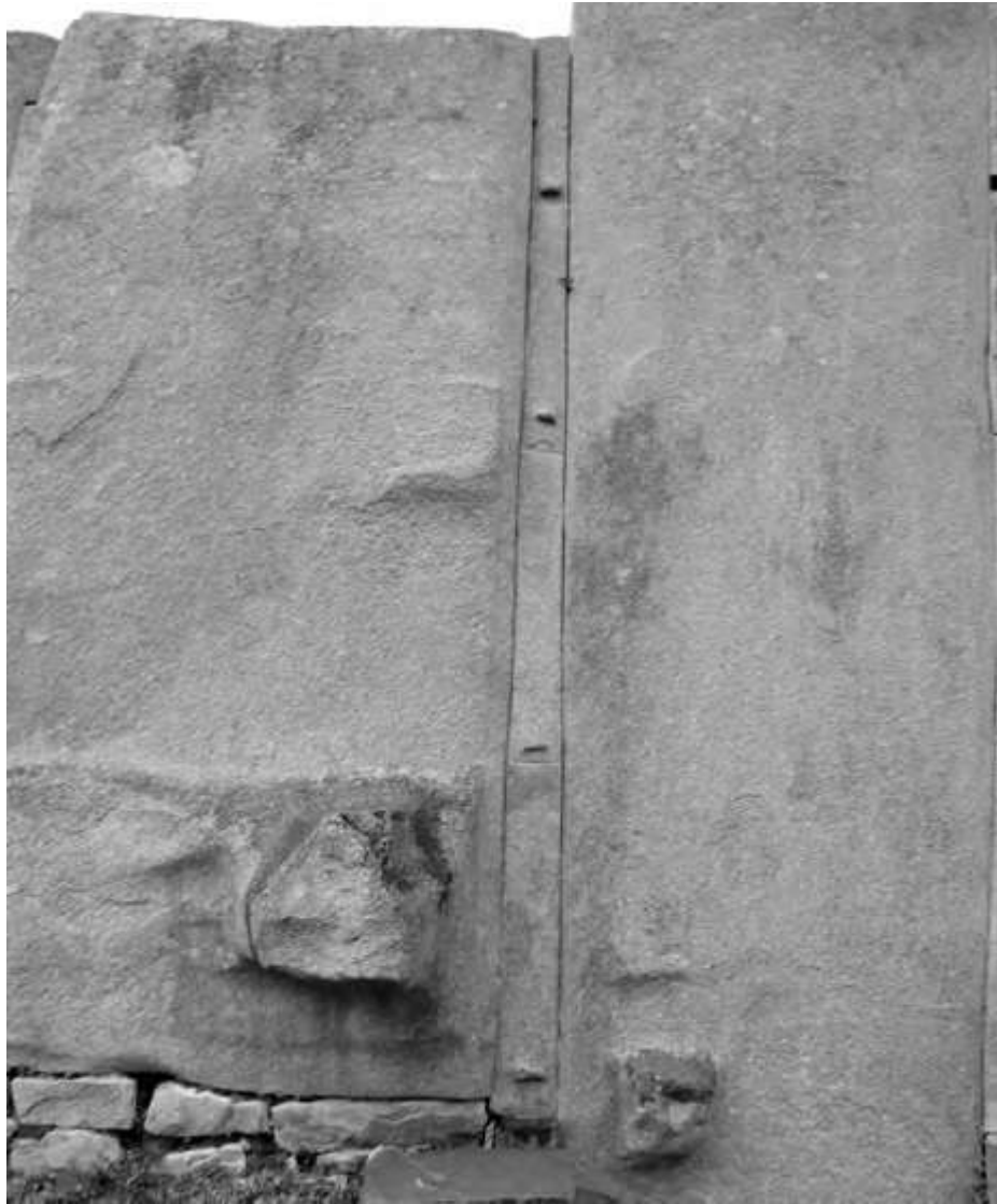
Close up of the thin sheets of rock at the Wall of Six Megaliths at Ollantaytambo.
