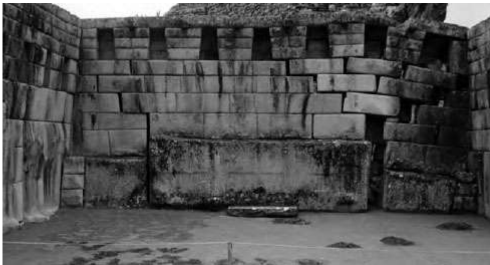
A view of the megalithic wall at the Main Temple with its wall pulling apart.
