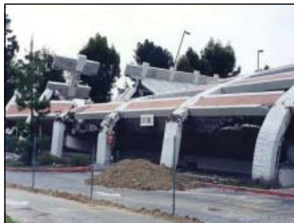
Aftermath of California's Northridge quake of July 17, 1994 (photo: Cal Tech.)
