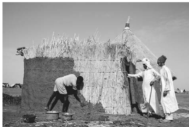
Men in Rashayda build a mud hut. In many areas of Sudan, there is little building material to work with other than what nature has provided. Even some government facilities, such as immigration and customs centers, are wattle-and-daub structures. © CORBIS. REPRODUCED BY PERMISSION.
