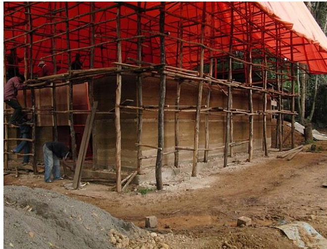
Picture 8. The first floor wall, built with rammed earth is completed. The picture also illustrates the scaffolding and weather protection. June 2010. [25]
