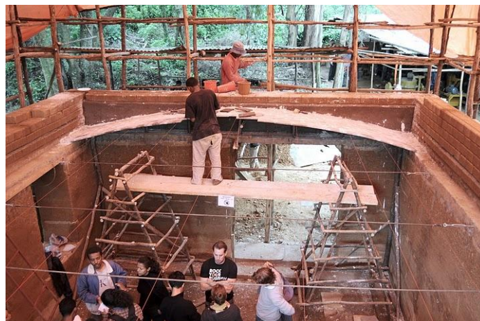
Picture 9. The construction of the 1 st floor vault is under process. 3 different layers of tiles containing 8 % cement were used. The CSSB-walls of the 2 nd floor are being constructed. July, 2010. [25]
