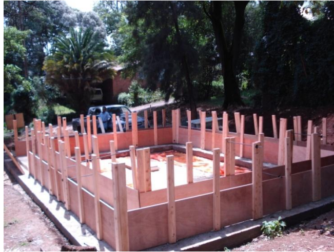
Picture 7. The concrete foundation is completed and formwork for the rammed earth is placed in position. May 2010. [5]
