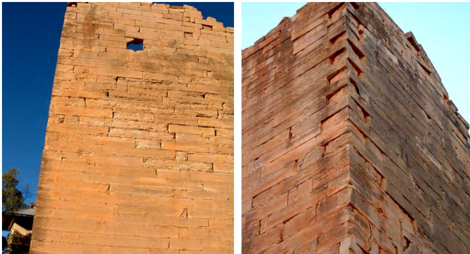
Figure 4. Regular rectangular sandstone blocks of up to 3 m length were used to construct the walls of the Temple, without the use of any mortar.
