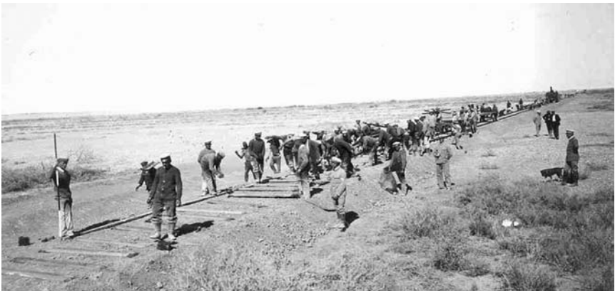
Construction of the Luderitz railway line using Herero slave labor. Courtesy of Klaus Dierks.
