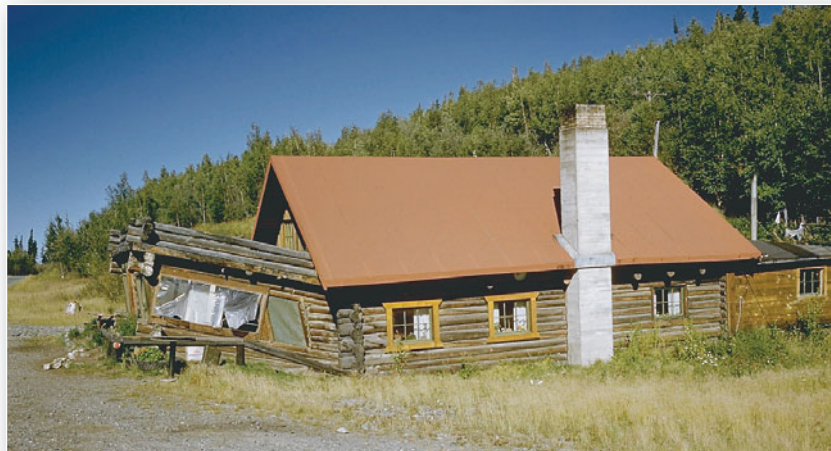
FIGURE 17.23 Permafrost melting and structure collapse.
