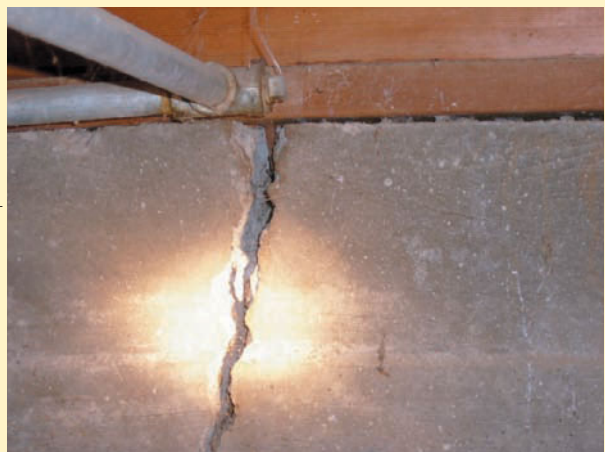
Foundation cracks due to expansive soils can cause serious damage to buildings that is expensive to repair.
