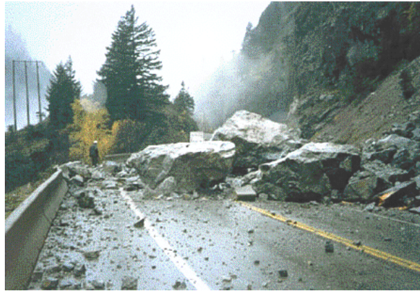
{PRIVATE} Figure 11h-5: Rockfalls from steep hillsides frequently disrupt road traffic in the mountainous regions of British Columbia, Canada. (Source: Image provided by Natural Resources Canada - Geoscape Vancouver ).
