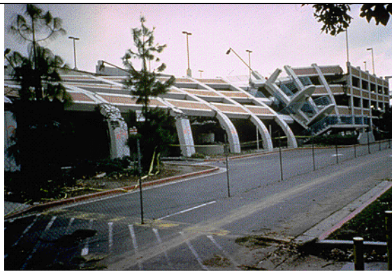
{PRIVATE} Figure 10m-8: A view of a parking lot on the campus of California State University. Columns of reinforced concrete failed after the 1994 Northridge earthquake and its aftershocks. ( Source: Photography by M. Celebi, US Geological Survey. Image provided by the National Geophysical Data Center, NOAA ).
