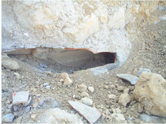
Fig. 2.15 Nabataean terracotta pipe (main Wadi Musa network) damaged by bulldozer, 2007 (Courtesy PNT)
