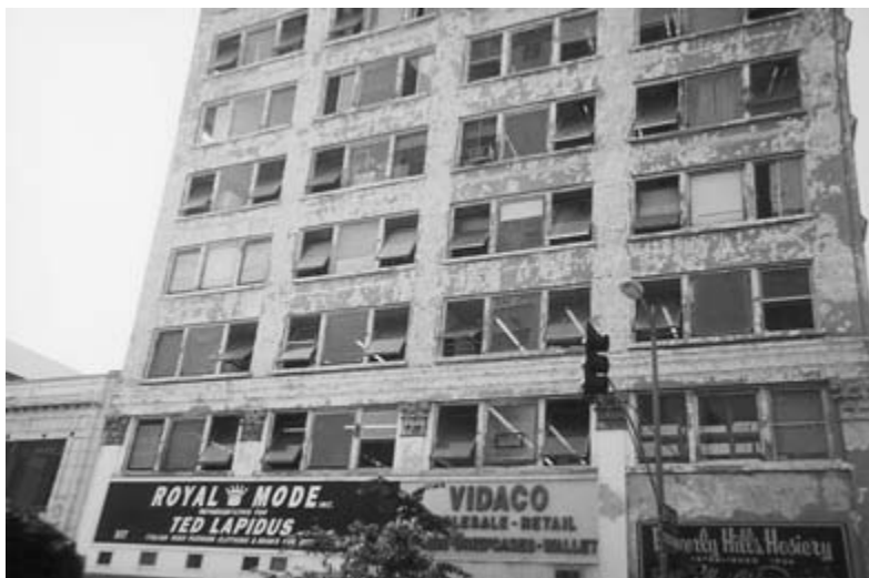
Old office building in the Los Angeles downtown, near fashion wholesale centers. Photographer: Robert J. S. Ross.
