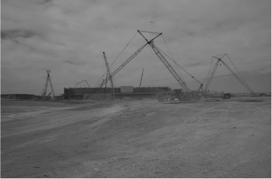
Louisiana Energy Services' uranium enrichment facility in Eunice, halfway through its four-year construction (see page 211). March 2008.
