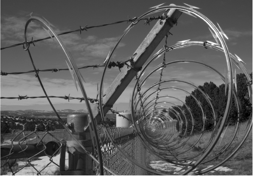
Booster pump station at the Buckman well field outside Santa Fe. February 2007.
