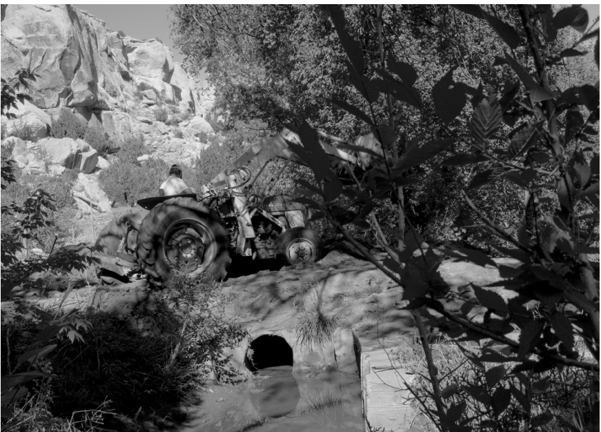
William on his "new" tractor attempting to fix a leak between two segments of culvert under a dirt bridge over the ditch. May 2008.
