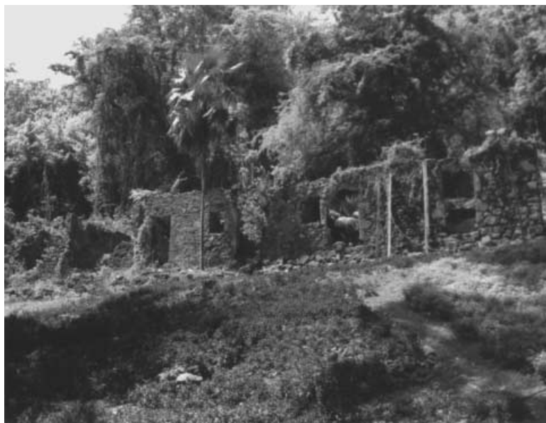
Figure 10: Crumbling walls of the slave quarters on the seventeenth-century Habitation Anse Latouche , Martinique
