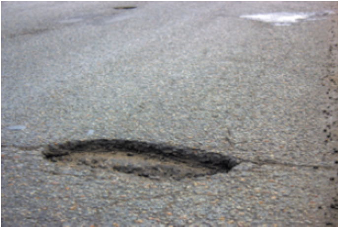
pothole 坑洼 kēng wā
