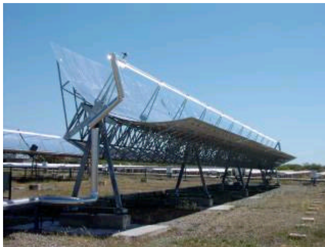
Figure 2-45: AndaSol: EuroTrough collectors [DLR 2003]
