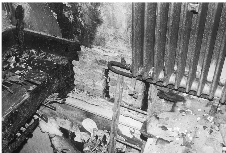
Figure 2.2 Convent fire view showing the area near the radiator
