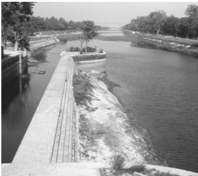
FIGURE 2.2 Seepage from an unlined canal is raising the water table.
