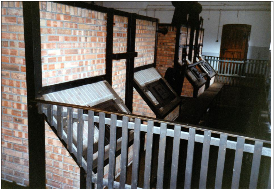
DOCUMENT 12: Gasifiers at the rear end of the two Topf triple-muffle cremation furnaces in the crematorium at the Buchenwald Camp. From: Mattogno/Deana 2015, Vol. III, Photo 205, p. 131.
