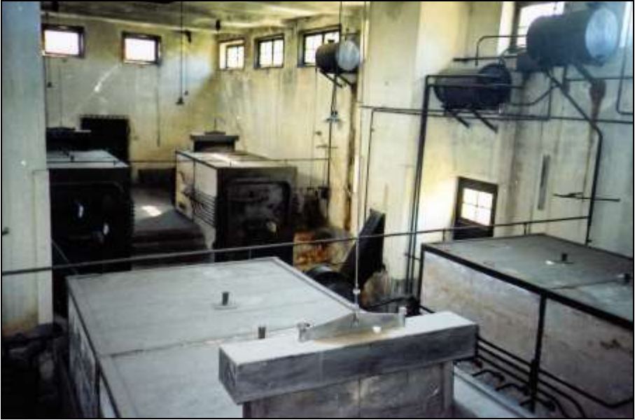
Photograph 345: The four furnaces viewed from above. On the right-hand wall, top, are the naphtha tanks.
