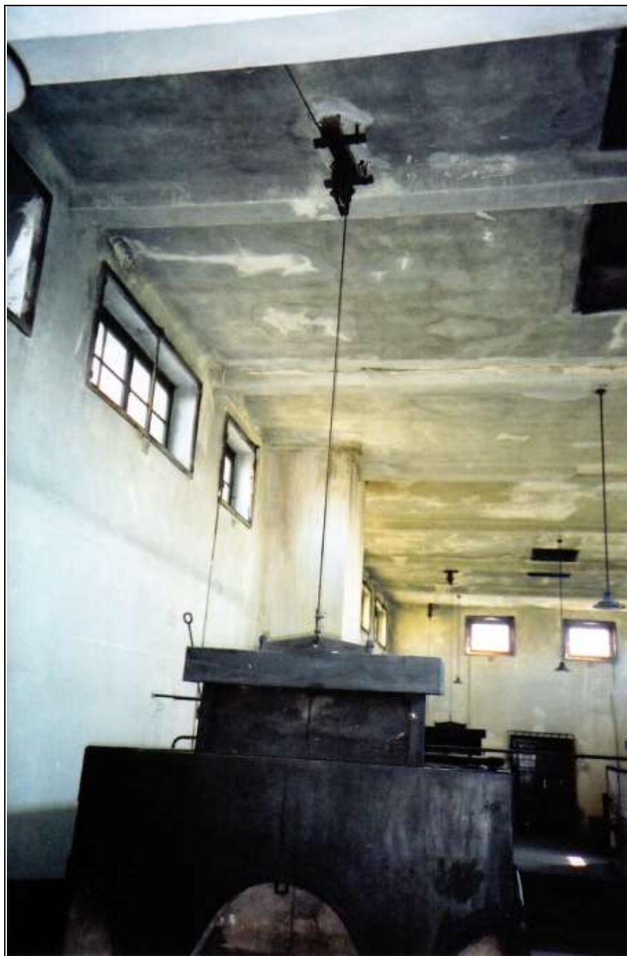
Photograph 360: left-hand furnace of front pair, front view; the damper's steel cable and pulley attached to the ceiling.
