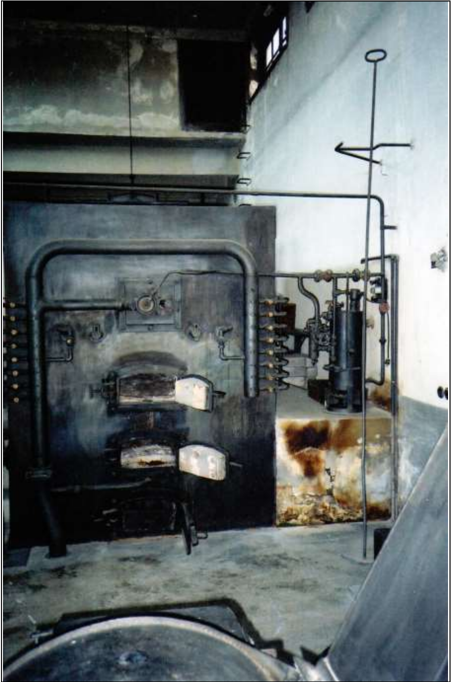
Photograph 349: as above; on the right, next to the wall, is the naphtha preheater behind a long scraper.
