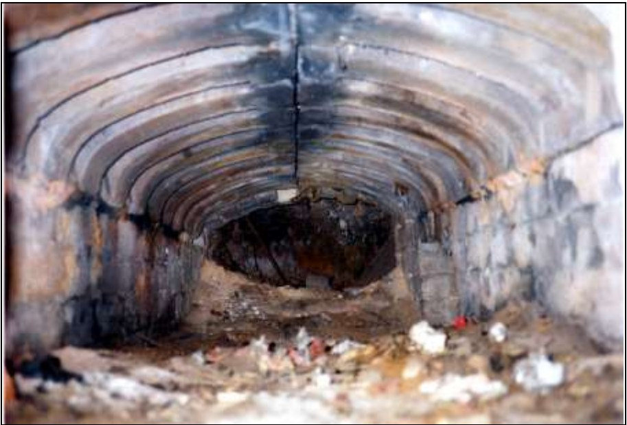
Photograph 275: as above, ash chamber.
