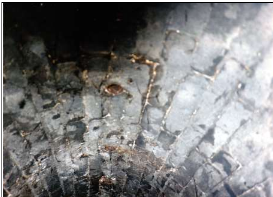
Photograph 61: Vaulted ceiling of the right-hand muffle; outlets of pipes connected to the blower.
