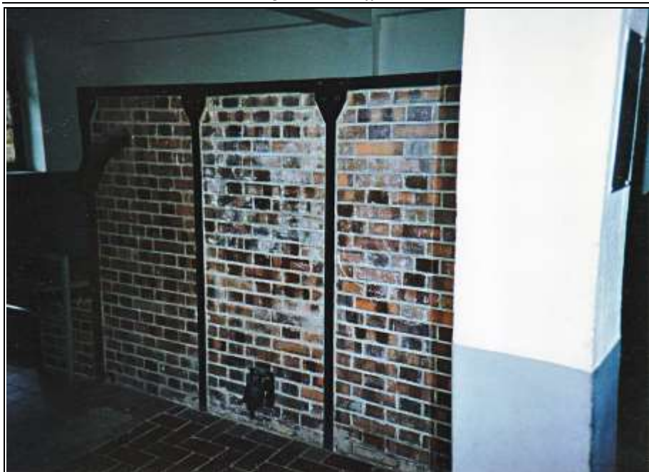
Photograph 73: Left side of the furnace: Door of the combustion-air-intake channel whose channel leads into the ash chamber of the left-hand muffle.
