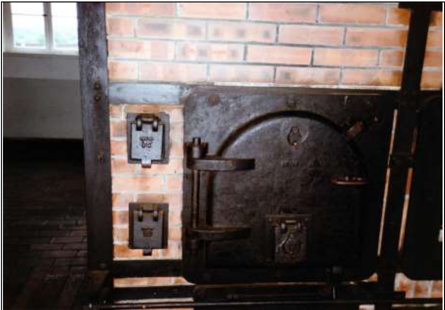
Photograph 150: as above, left-hand muffle. To the left of the large muffle door: doors closing the combustion-air channels of the muffle (top) and of the ash chamber (bottom).
