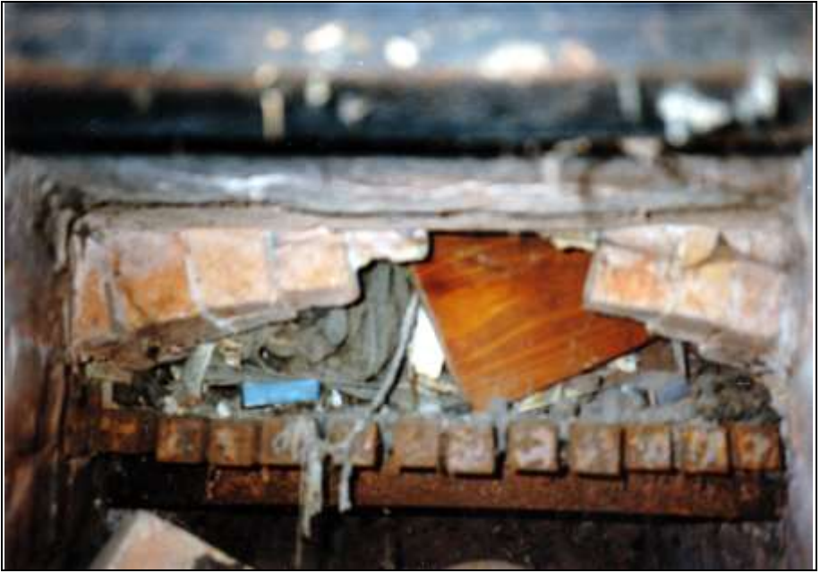
Photograph 177; as above; view into the gasifier's ash chamber with the grate.
