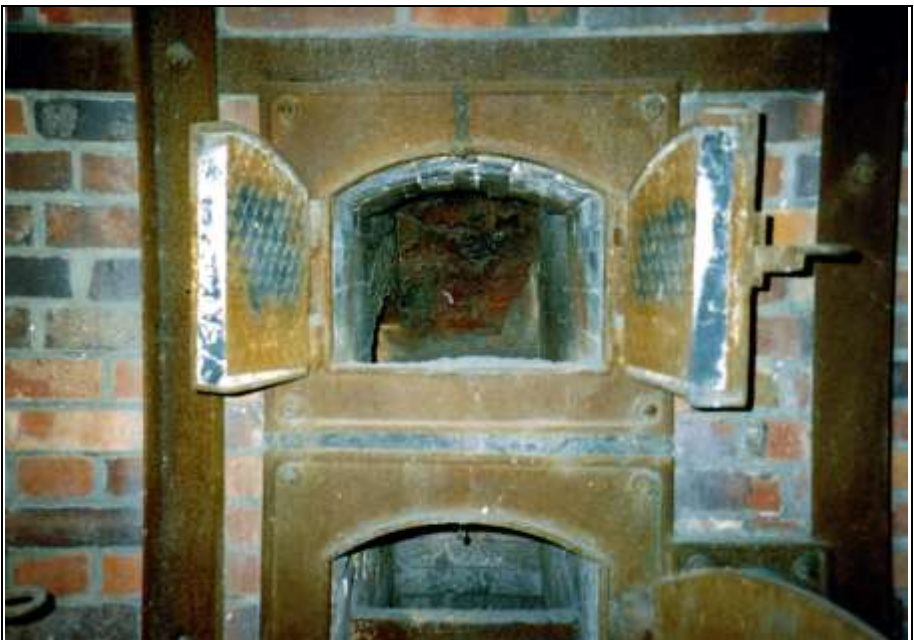
Photograph 261: Coke-loading door of the main gasifier.
