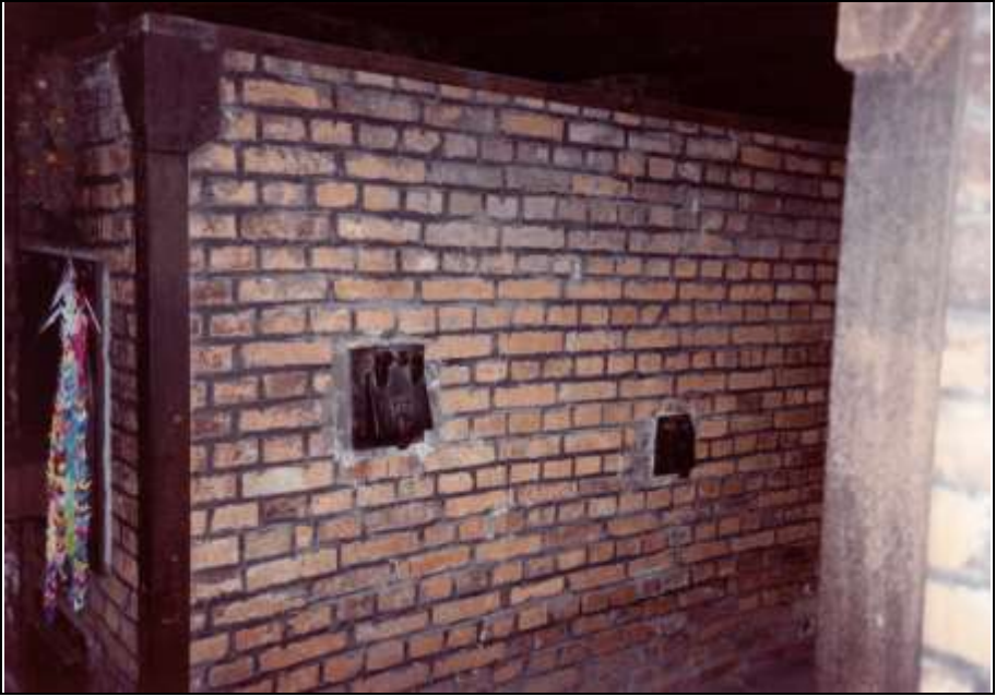
Photograph 96: Furnace No. 1, right-hand side. Original doors of combustion-air channels. The Polish refabrications did not include those channels. The number, type and position of the doors are also wrong. The larger door originally belonged to an eight-muffle furnace, and the smaller door was located lower. Cf. Photo 73.
