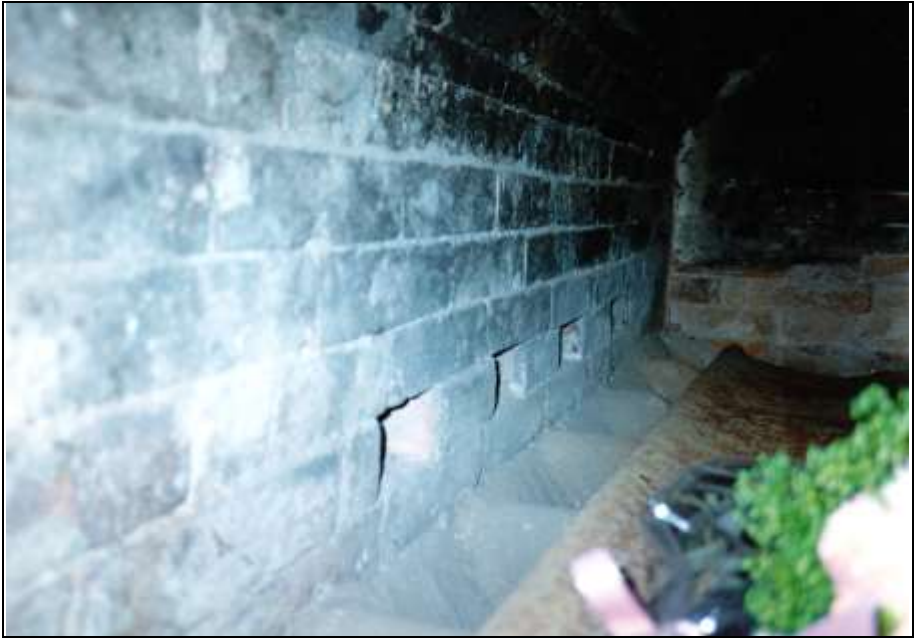
Photograph 54: Left-hand muffle with four holes for introducing combustion air.
