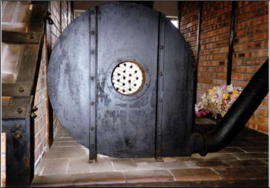
Photograph 195: Combustion-air blower for the oil burner of the furnace fueled with either naphtha or coke. Rear view.
