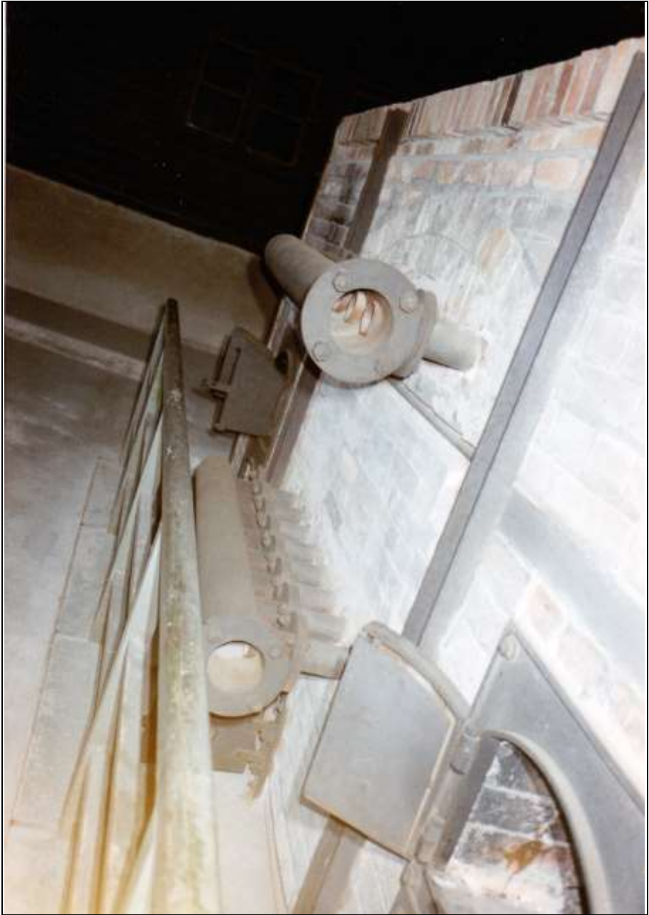
Photograph 308: as above. Hot-water pipes of the recuperator.
