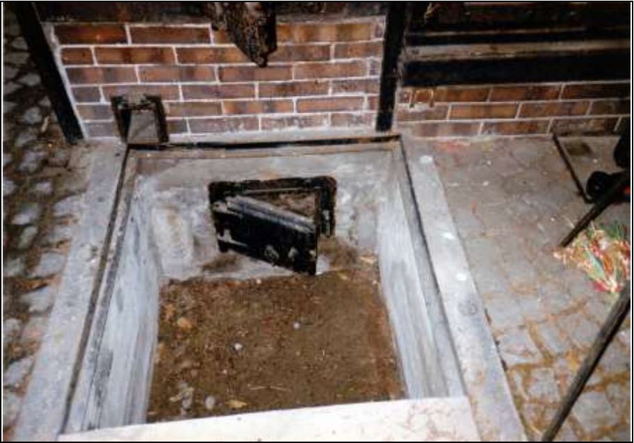
Photograph 7: Left-hand gasifier: slag/ash-removal door and service pit.
