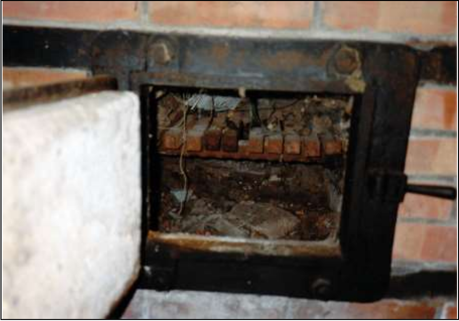
Photograph 167: as above, view into the gasifier's ash chamber with the grate.
