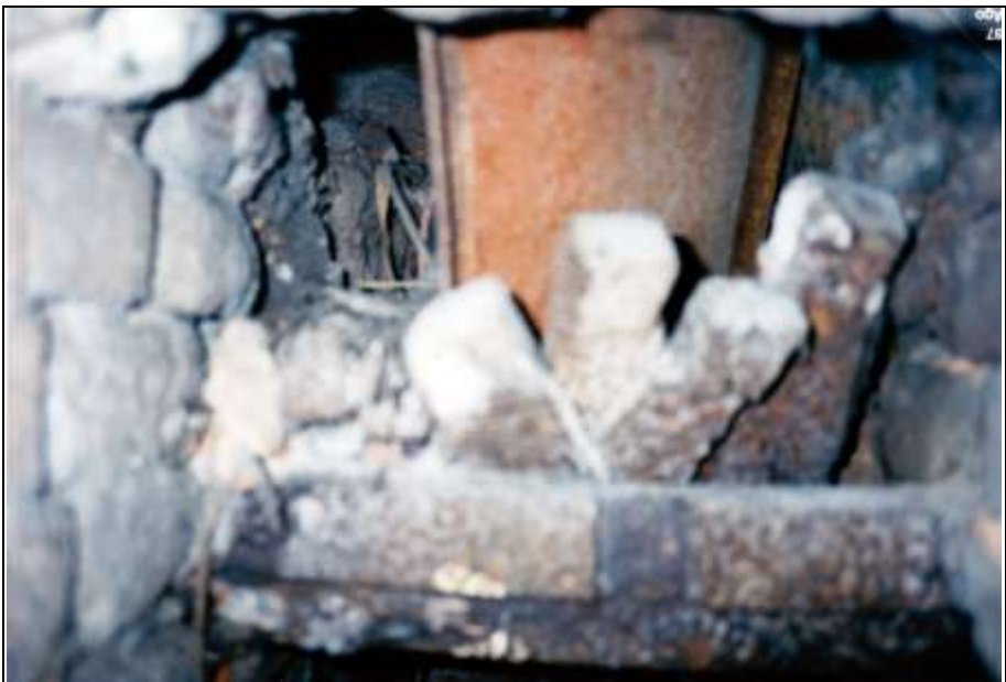
Photograph 277: Inside the right-hand furnace's main gasifier viewed through the ash-chamber door. The hearth's grate has been damaged, with only four remaining bars merely leaning against the outer support bar.
