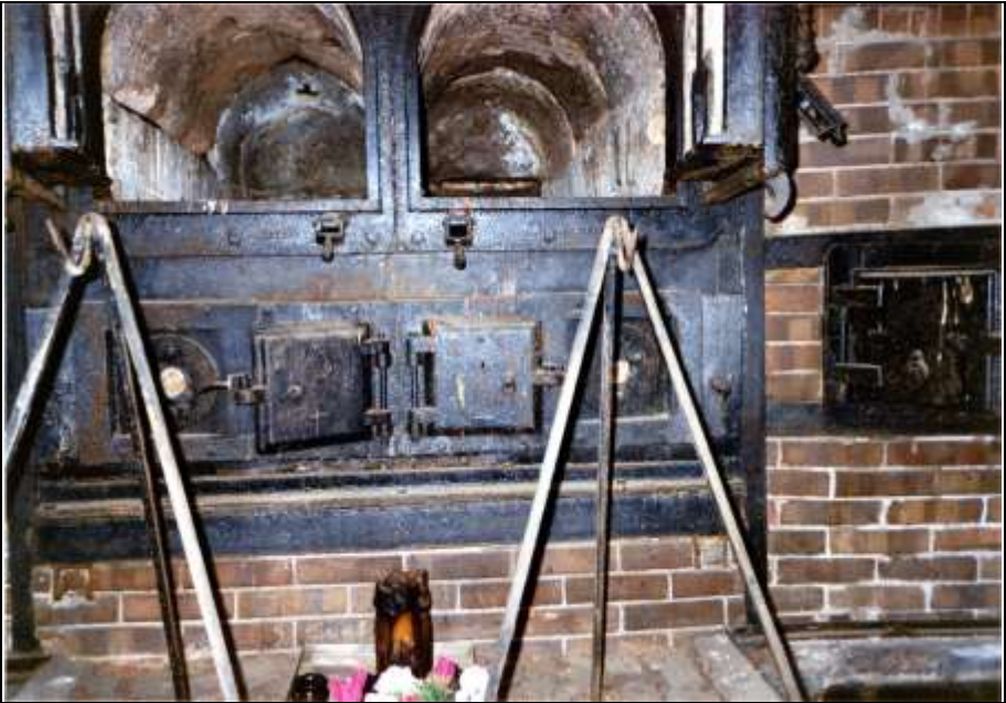
Photograph 3: Ash doors of the muffles. At the sides the original combustion-air-intake holes.
