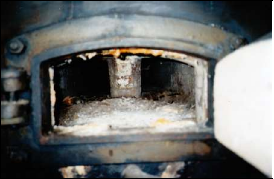
Photograph 354: as above; inside of the post-combustion chamber seen through its rear service door.
