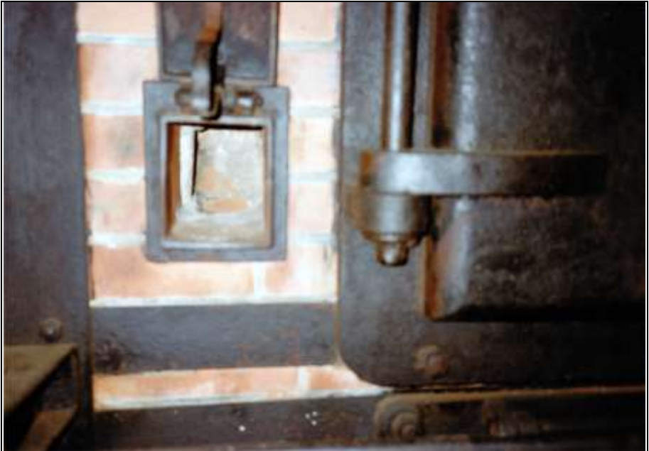
Photograph 152: as above, the ash chamber's combustion-air-supply channel.
