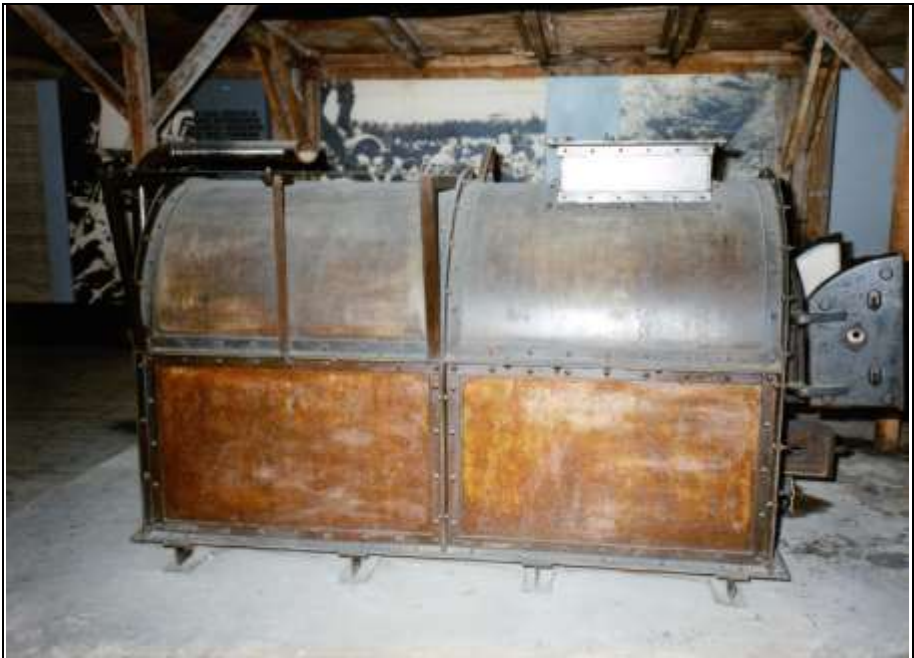
Photograph 325: as above. In the upper part of the furnace can be seen the combustion-air pipe for the burners (left), the support bars for the fan and its motor (center), and the base of the chimney (right).
