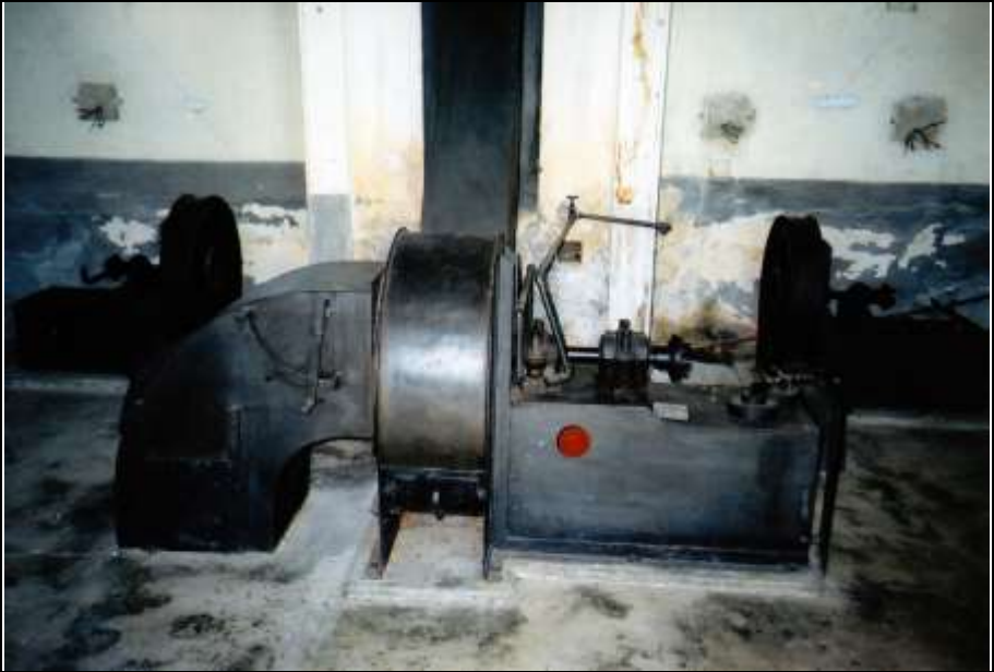
Photograph 356: Forced-draft blower of the front pair of furnaces, with suction duct (left), chimney duct (center) and the motor (right). In the background left and right the two combustion-air blowers.
