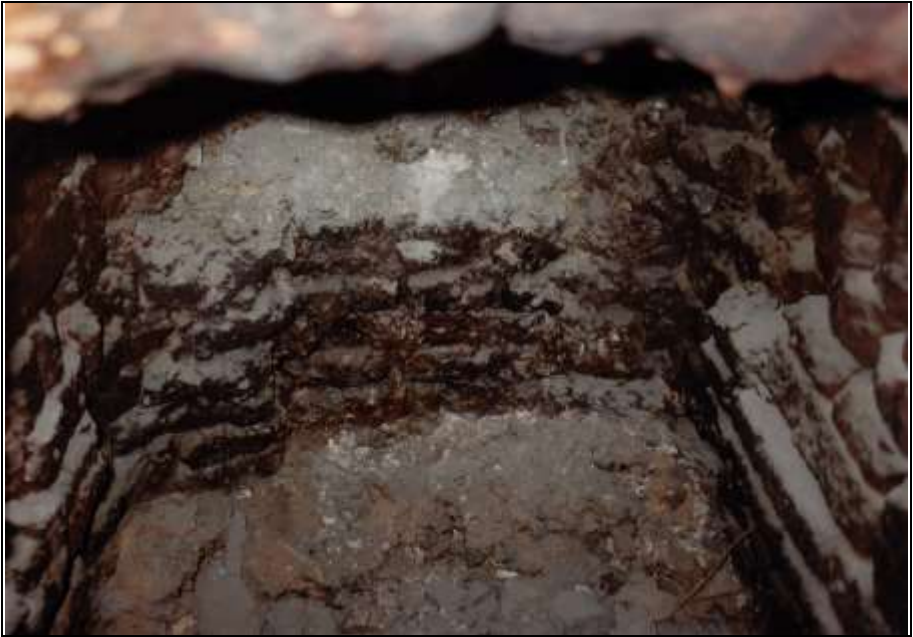
Photograph 164: as above; inside of the gasifier. The masonry shows signs of fusion.
