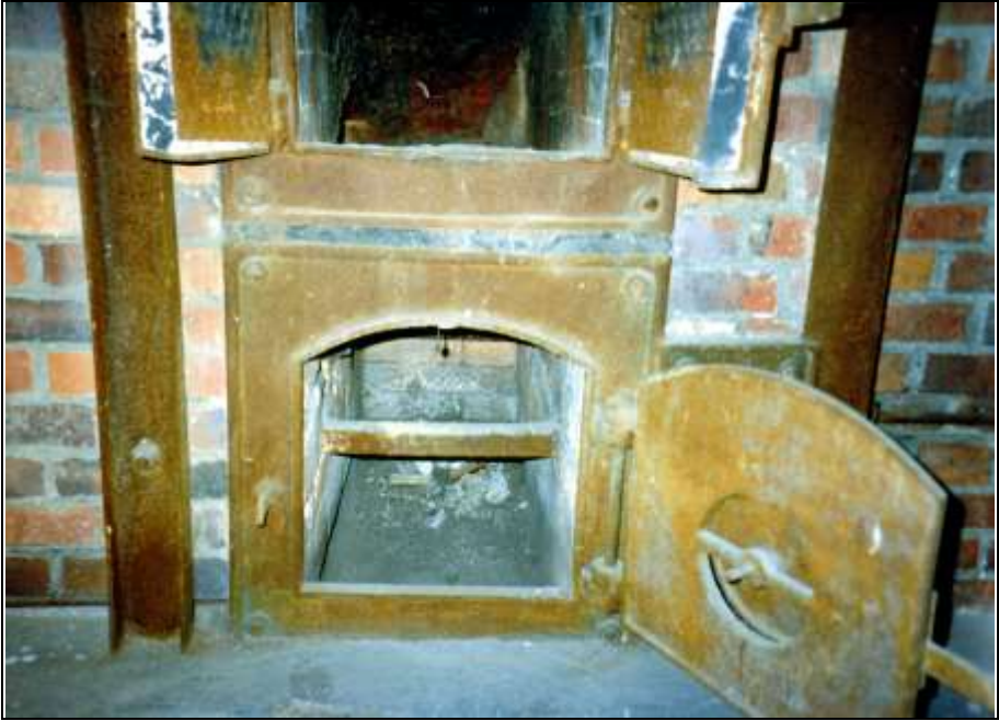
Photograph 262: Ash-chamber door of the main gasifier.
