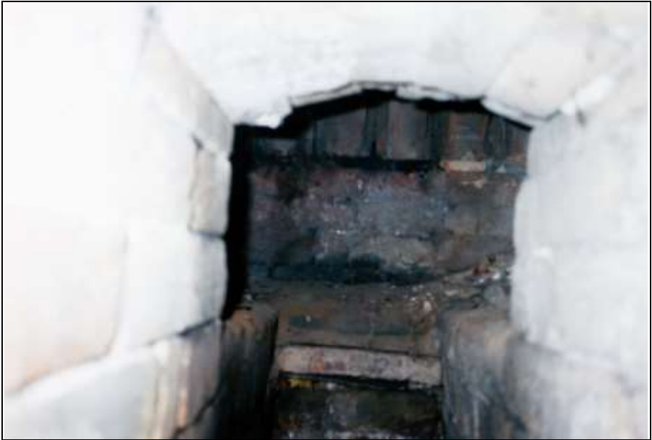
Photograph 283: Right-hand furnace, inside of the auxiliary gasifier with the muffle's ash chamber wall in the background and the muffle grate above.
