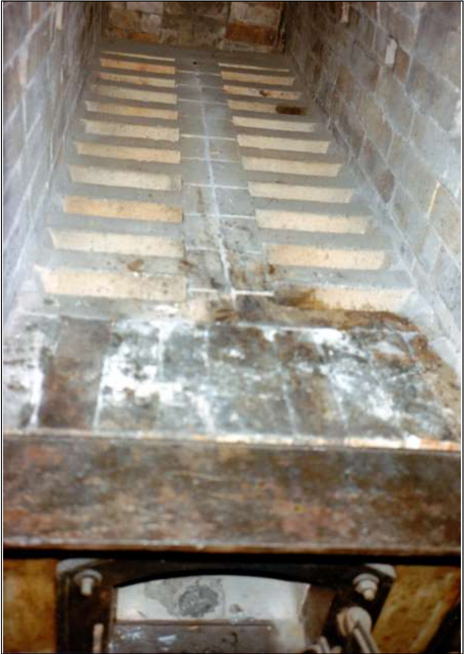
Photograph 322: as above; the refractory grate; bottom: ash-chamber door.
