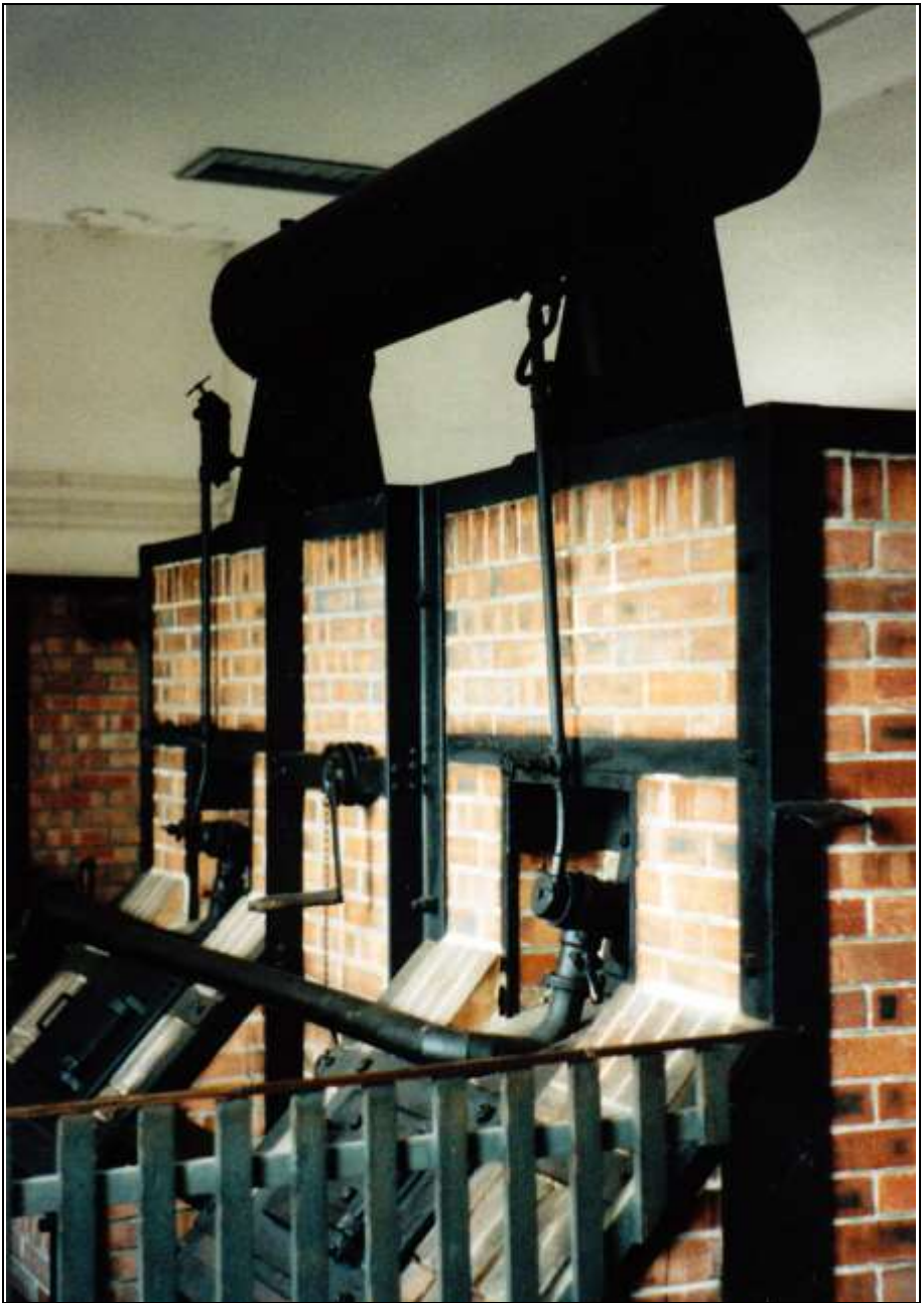
Photograph 201: as above, right-side rear view; tube connection with naphtha burner.
