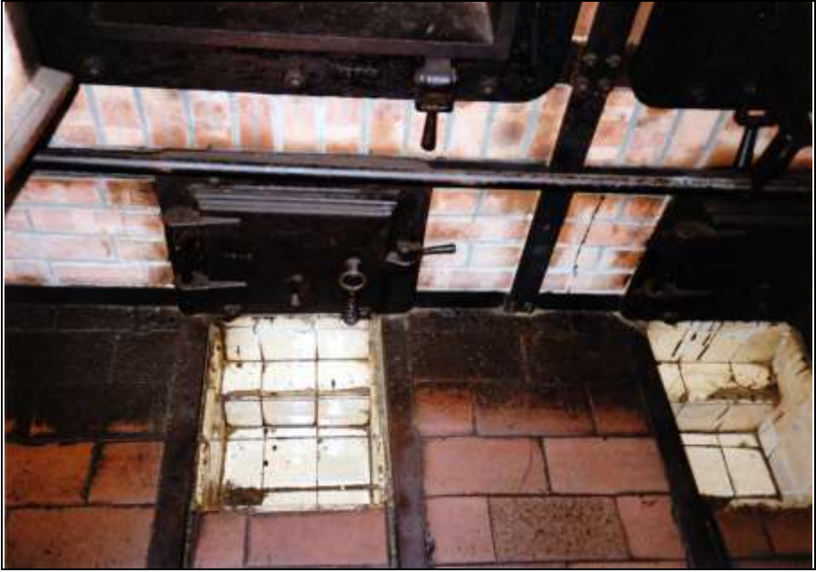
Photograph 155: TOPF coke-fired triple-muffle cremation furnace. Front-side service pits with the left and center muffles' ash doors.
