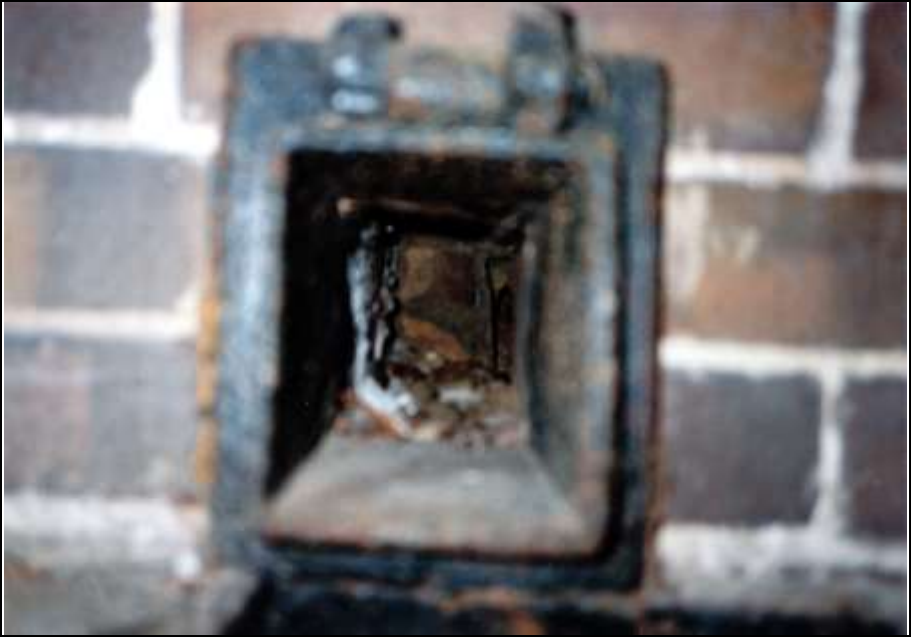
Photograph 6: Left-hand gasifier's primary air intake.
