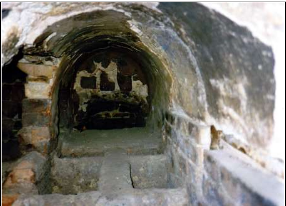
Photograph 40: Inside of the right-hand muffle with muffle grate.
