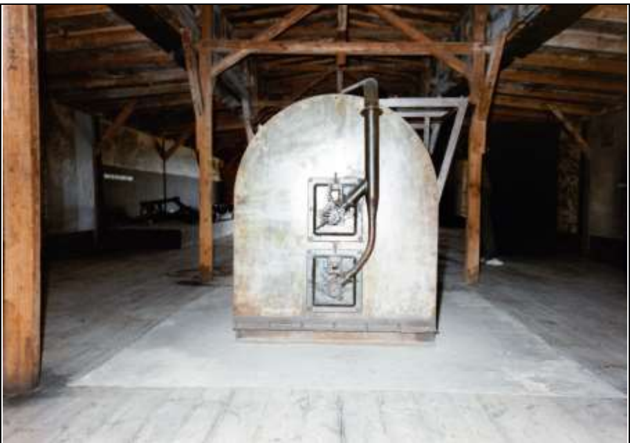
Photograph 327: rear view; combustion-air pipe with main (center) and auxiliary burners (bottom).
