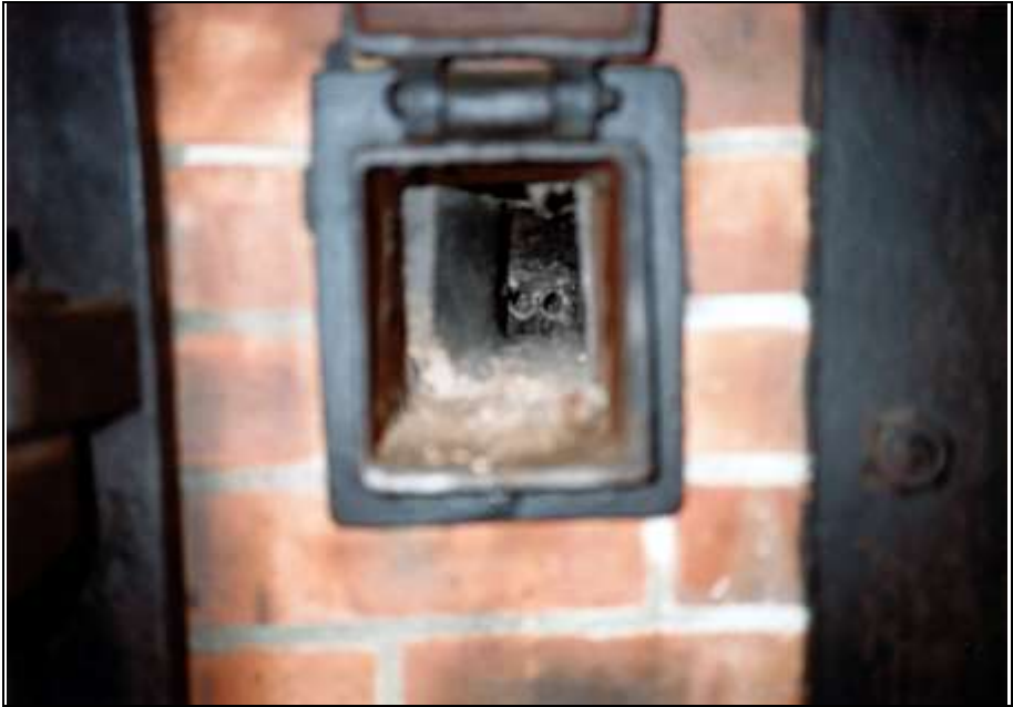
Photograph 149: as above, the muffle's combustion-air-supply channel.
