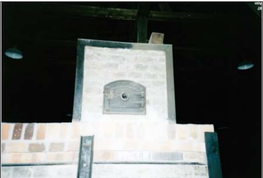
Photograph 310: as above, smoke duct with inspection door.
