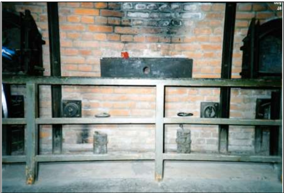
Photograph 289: as above; first recuperator.
