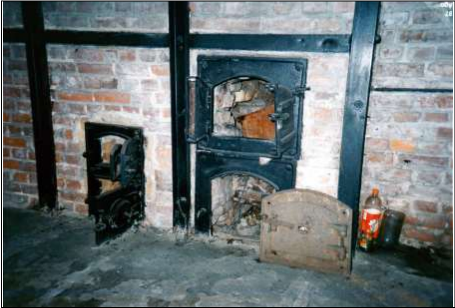
Photograph 276: Right-hand furnace. To the left: coke-loading door (center) and ash door (bottom) of the auxiliary gasifier. Center: double-leaf coke-loading door of the main gasifier with the ash-chamber door beneath.
