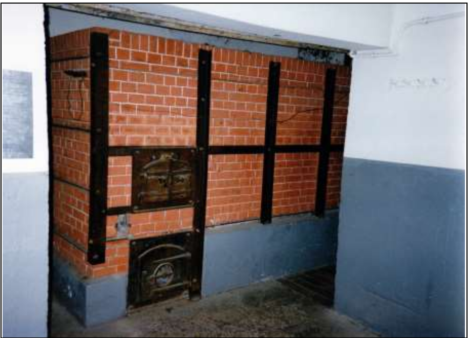
Photograph 245: left-hand side view; the gasifier's coke-loading door (top) and ash door (bottom).
