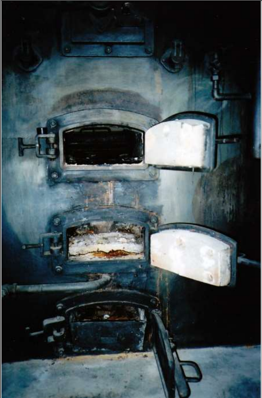
Photograph 351: Left-hand furnace of the front pair, rear view; the three service doors: for the muffle (top), the post-combustion chamber (center) and the ash chamber with the ash receptacle (bottom).
