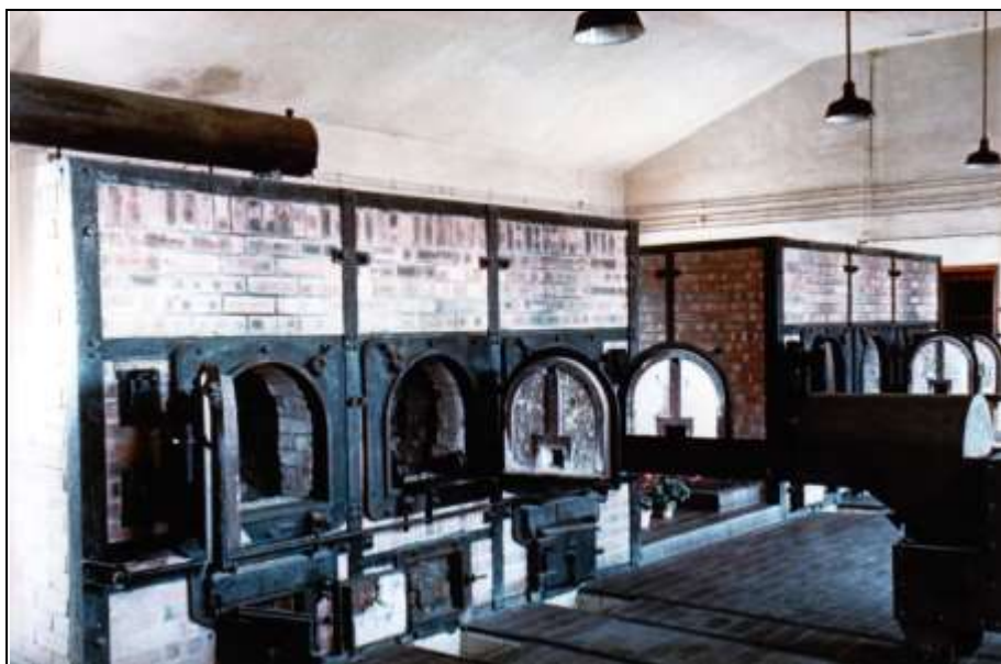
Photograph 116: TOPF triple-muffle cremation furnace in the crematorium at Buchenwald Concentration Camp.
