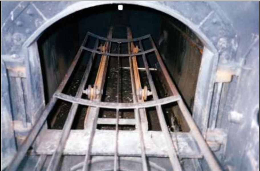
Photograph 334: Interior. The introduction stretcher moved with four metal rollers on two angle irons. The opening in the back wall housed the main burner. The refractory lining has been completely removed.
