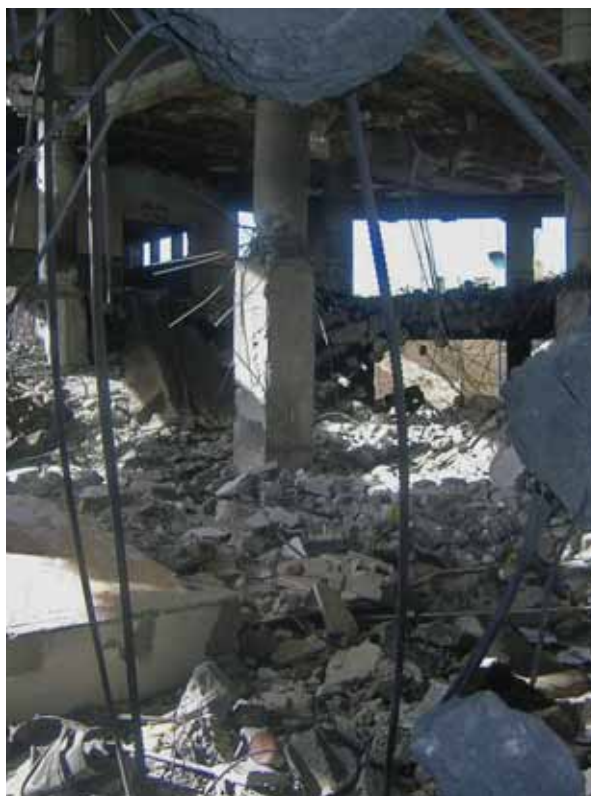
Damaged building in the Gaza Strip
