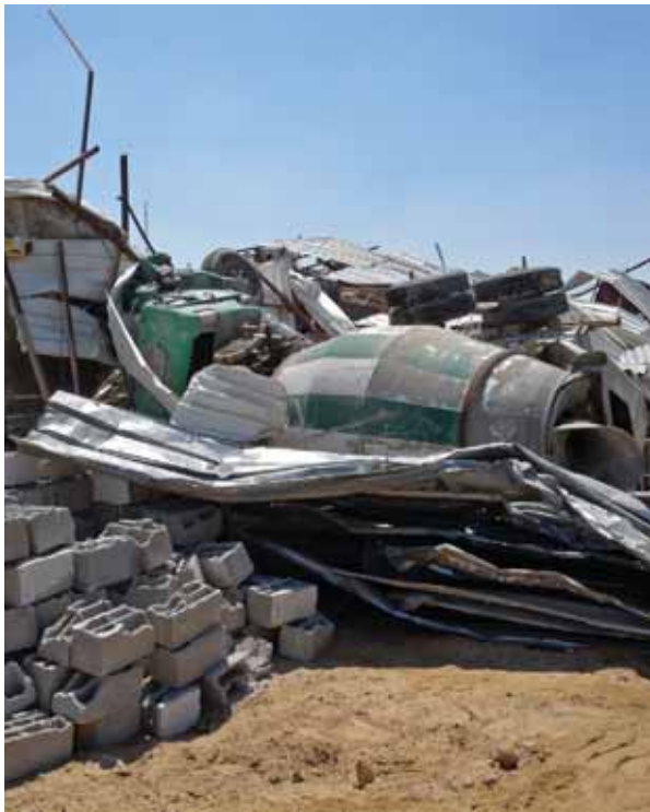
Bulldozed cement plant near Rafah
