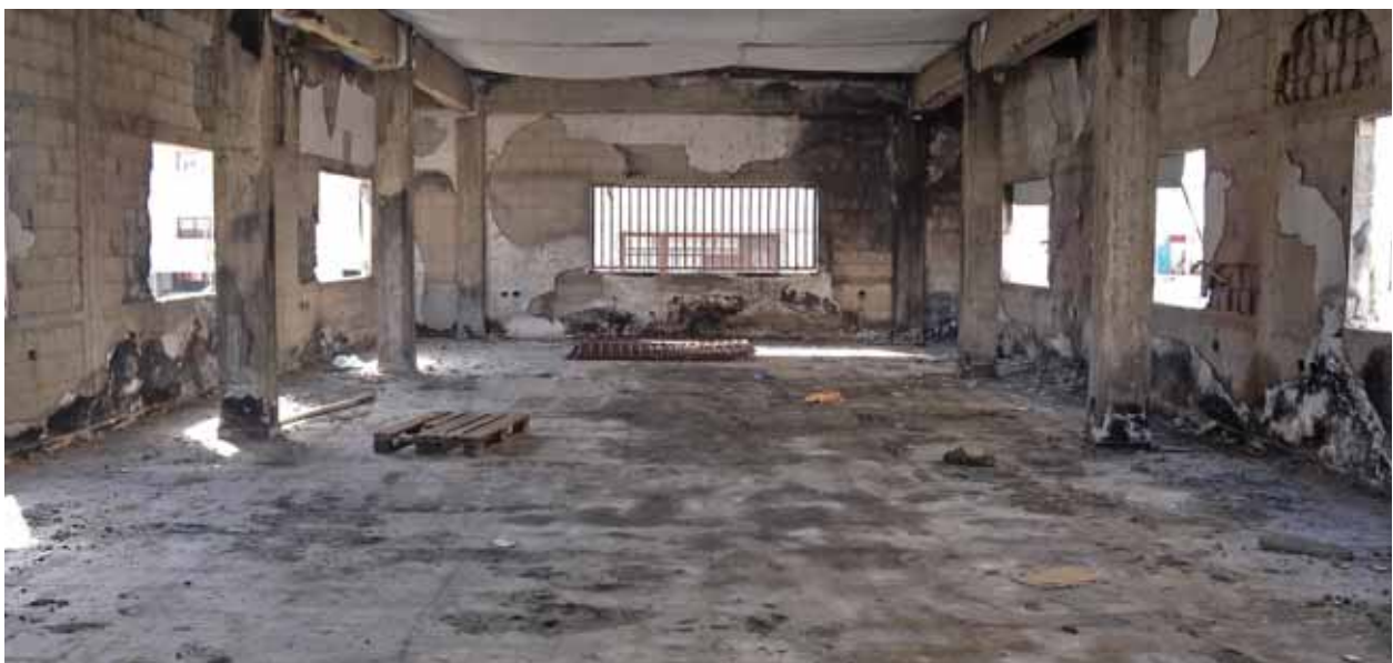
Burnt out interior of the Red Crescent building in Gaza City
