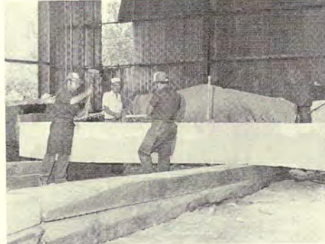
A special crew under the direction of Joe B. Davis, a retired plant superintendent, was hired to cut and pitch the slabs to the exact dimensions provided by "Mr. Christian." Special crews were hired because the project was so demanding that it would disrupt the regular Elberton Granite Finishing Corporation production schedule.
