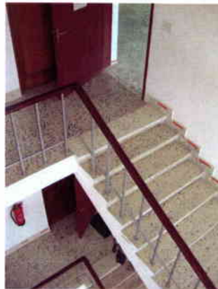
Figure 4 Lack of fire egress
