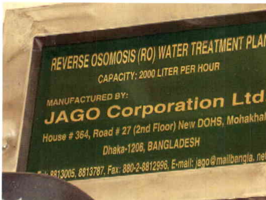
Picture 2: Plate affixed on the water purification plant of Bangladesh Contingent
