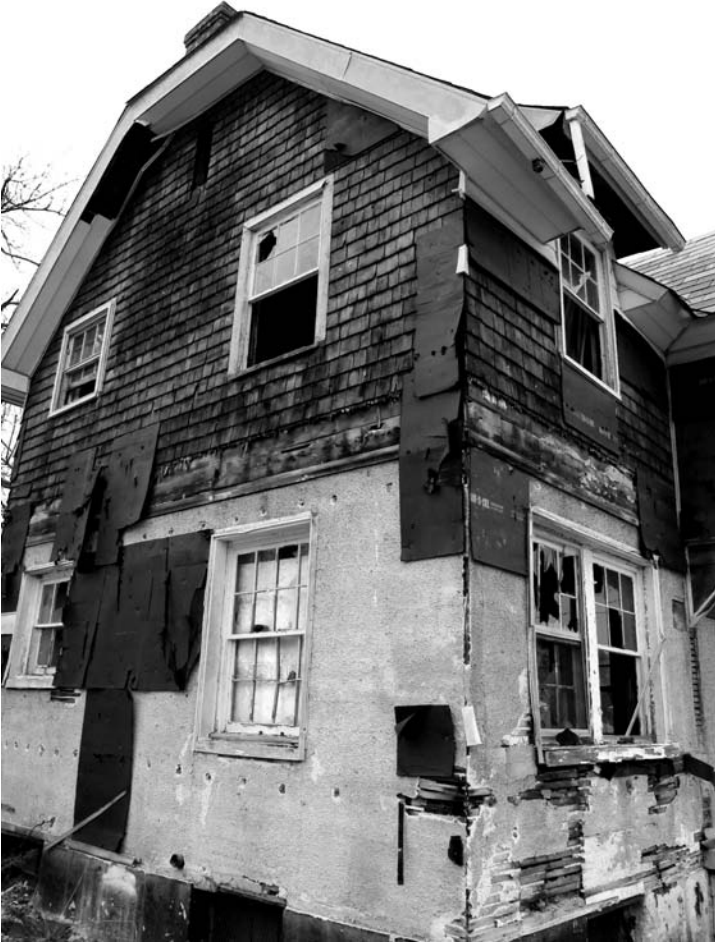
FIGURE 14. Throughout the city, abandoned houses like this one in Civic Park are ravaged by thieves known as scrappers in search of any metal they can resell—doorknobs, radiators, aluminum siding, but especially copper wiring and plumbing. (Photo by Gordon Young)
