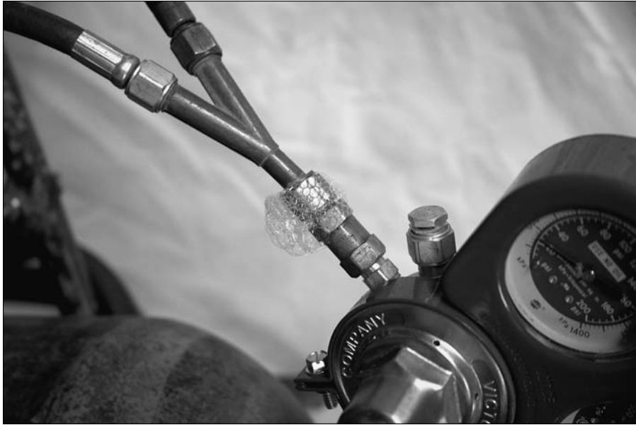
Figure 3-4: An example of a leak- ing oxygen hose.
