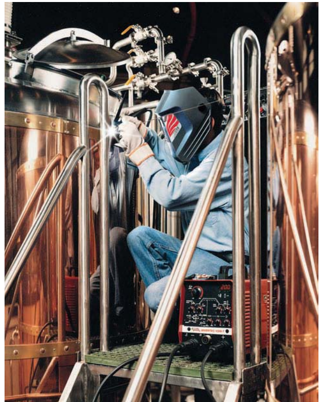
Figure 4.16 An operator GTA welds a cap ring on a pneumatic tank Courtesy of Lincoln Electric Company
