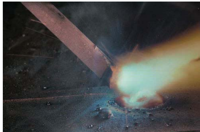
Figure 2.3 If the flux is broken off the end completely or on one side, the arc can be erratic or forced to the side Courtesy of Larry Jeffus
