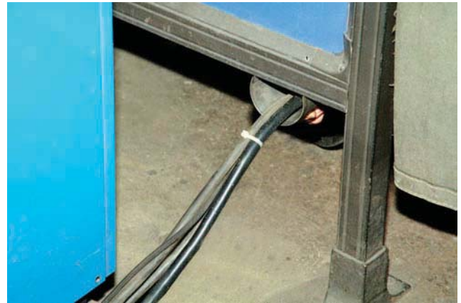
Figure 4.24 A bracket holds the leads off the floor Courtesy of Larry Jeffus
