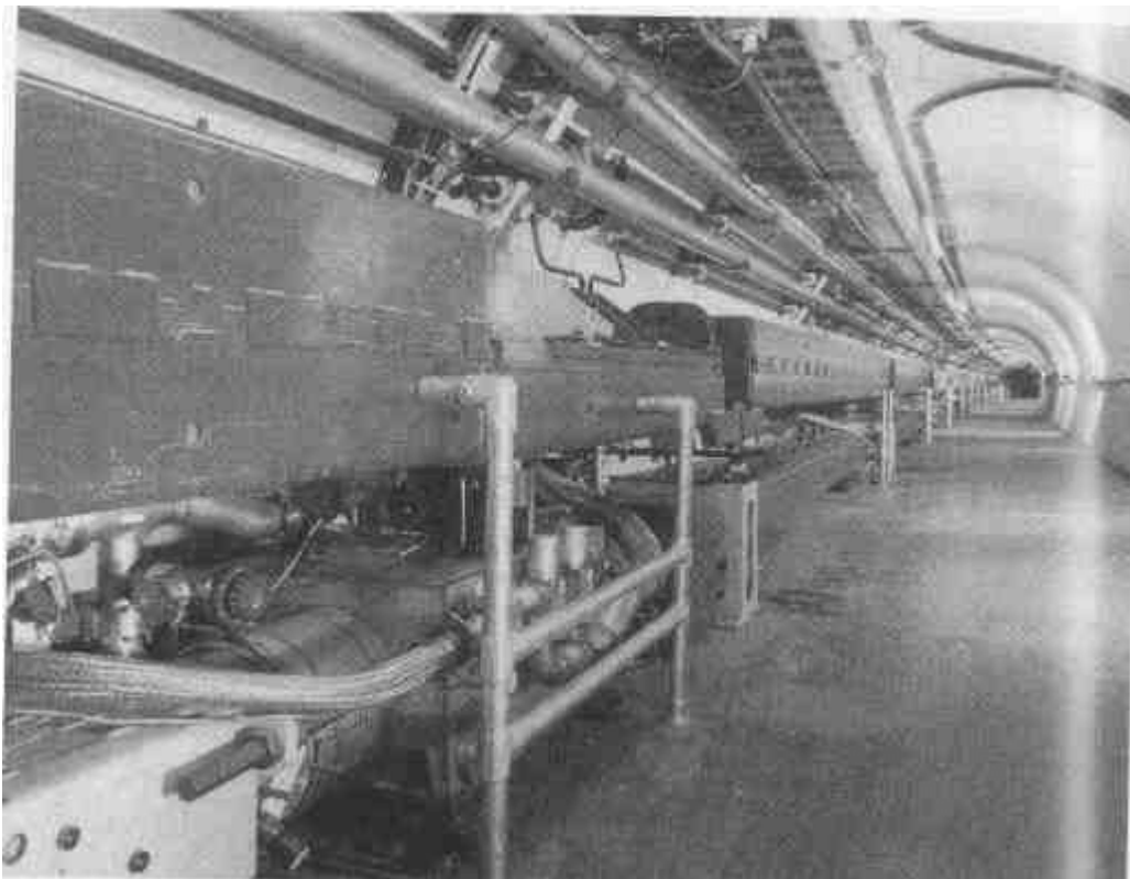
A portion of the accelerator tunnel, 4 miles long, located 20 feet below the ground, housing the proton-antiproton beams, and the array of superconducting magnets (lower ring) used to steer and accelerate them to energies approaching 10^{12} electron volts. {Fermilab Photo}
