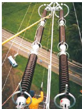
☑ Insulators of a 380-kV transmission line: Made of porcelain or glass, the insulators carry the conductor ropes, which have a very high voltage compared to the earth potential of the masts. They ensure that this high voltage does not lead to a flashover (similar to lightning) between the conductors and the mast. Source: Arbeitskreis Schulinformation Energie
