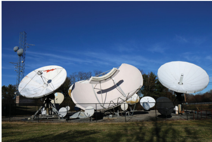
Figure 10.13a Antennas at the studios of the WDBJ television station in Roanoke, Virginia. The reflector antennas are all used for satellite communications. The center antenna is a Simulsat design capable of receiving signals from multiple satellites. The large antenna at the left of the photograph has a Gregorian configuration with a shaped subreflector. The two antennas on the mast link to WDBJ's broadcast antenna on Poor Mountain.
