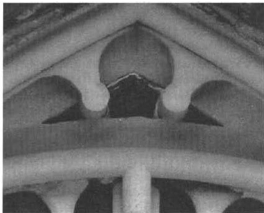
Figure 13 Exterior view of the light box at the east end of Rosslyn
