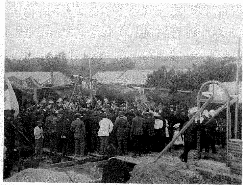
Charles Aburrow, Deputy District Grand Master of the Transvaal, laying the foundation stone of the new temple for Royal George Lodge at Krugersdorp, Transvaal, 29 October 1898 (copyright, and reproduced by permission of, the United Grand Lodge of England).
