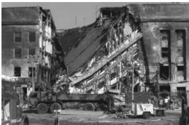
The west-facing wall of the Pentagon sags where a hijacked American Airlines flight with 64 passengers aboard was purposely crashed into this spot in an act of terrorism. (R. D. Ward/Department of Defense)
